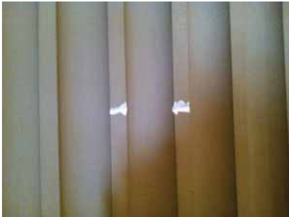
Fig. 3.1.C.13 Typical damage and deterioration noted to the decorative plaster throughout.
