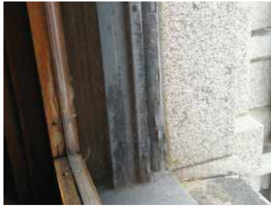
Fig. 2.1.A.18 Generally faded and peeling paint observed at the wood window frames.
