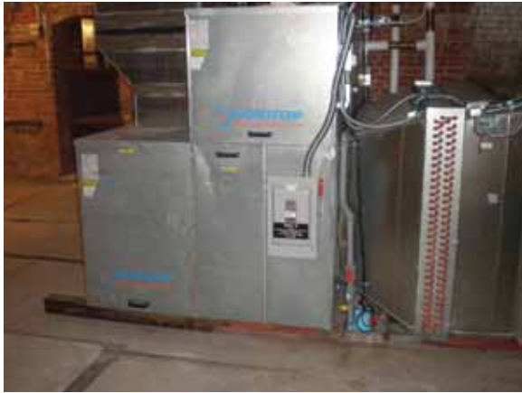
Fig. 2.4.A.24 – Geothermal heat pump
