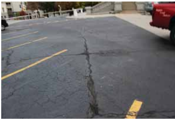
Figure 2.3.A.8 Poor Site Asphalt Condition
