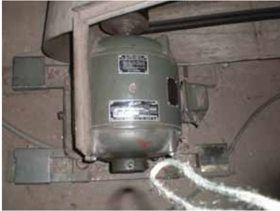
Fig. 2.4.A.43 – Standard efficiency motor for exhaust fan in attic
