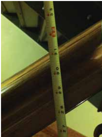
Fig. 2.1.B.8 The height to the top of the handrails, measured above the stair tread nosing, throughout the stairways from the Basement Floor to the Third Floor.
