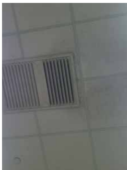
Fig. 3.1.C.1 Soiling of the acoustic ceiling tiles near air diffusers.
