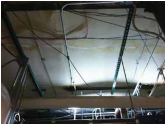
Fig. 3.1.C.6 Evidence of water damage noted at the ceiling on the Sub-basement Floor.
