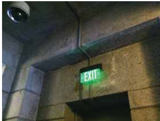
Fig. 3.1.C.22 Water damage noted at the granite cladding on the walls of the south accessible entrance vestibule on the Basement Floor.
