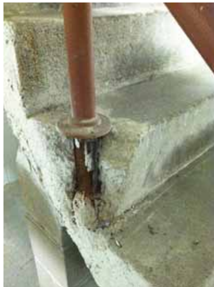
Fig. 2.1.B.10 Loose railing at the stairway leading from the south tunnel to the main floor of the sub-basement.
