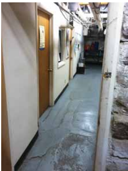
Fig. 3.1.C.47 Spalling and deteriorating concrete flooring with the paint wearing off observed on the Sub-basement Floor.
