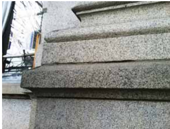
Fig. 2.1.A.12 Widespread deterioration of the material between the joints of the granite panels.
