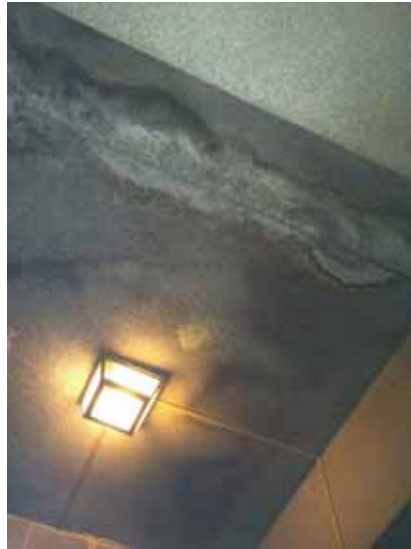
Fig. 3.1.C.2 Water damage noted at the granite cladding on the ceiling of the west emergency exit vestibule on the Basement Floor.
