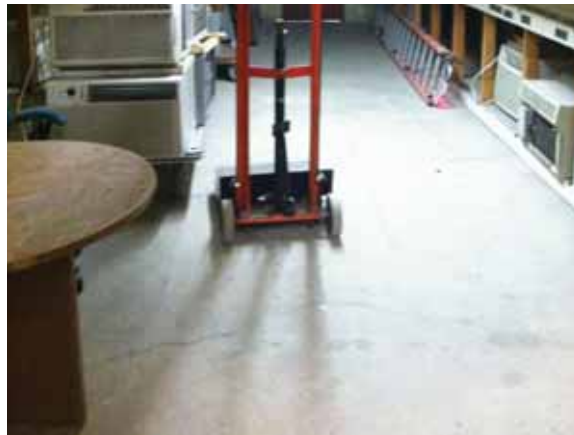
Fig. 3.1.C.48 Areas of cracked concrete flooring observed throughout the Sub-basement Floor.
