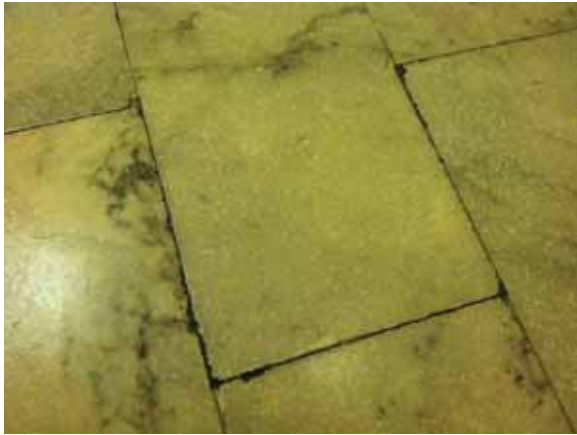
Fig. 3.1.C.33 Typical deterioration of the marble flooring observed throughout.
