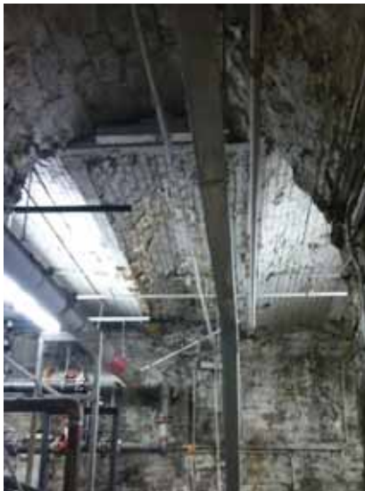
Fig. 3.1.C.7 Evidence of water damage, corrosion, and deterioration at the vaulted masonry ceilings of the areas of the tunnels included in the site survey visit.
