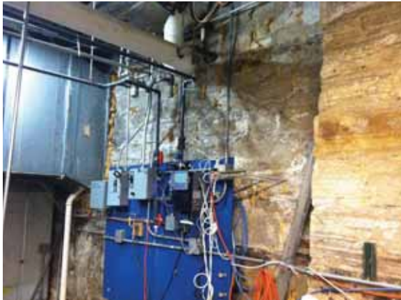
Fig. 3.1.C.30 Equipment located at a wall that appears to have issues with water infiltration and has been temporarily repaired in spots with a foaming waterproofing material.
