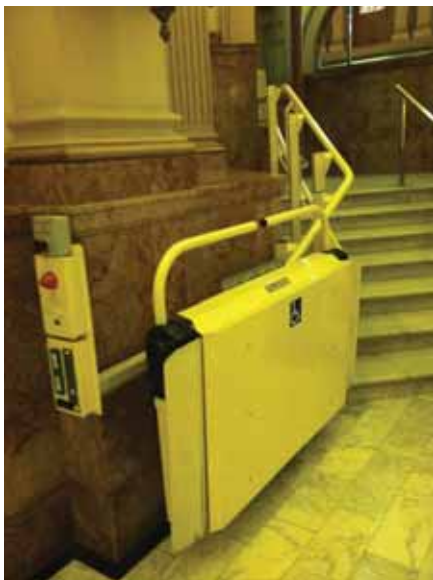
Fig. 2.1.C.7 Wheelchair lift observed on the Second Floor outside of the House of Representatives Gallery.
