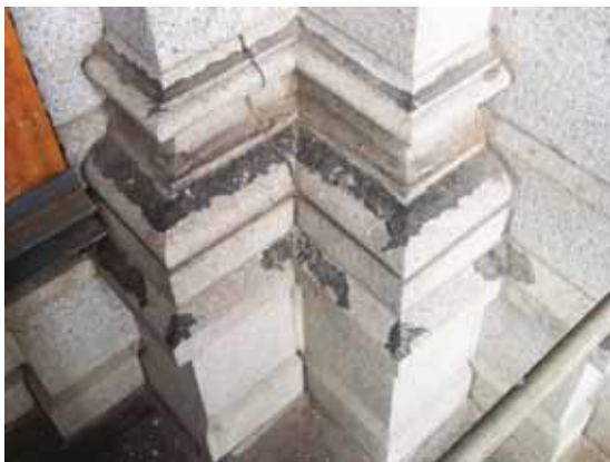
Fig. 2.1.A.10 A black rubber-like material that was applied to areas along the exposed top edges of the granite is deteriorating.
