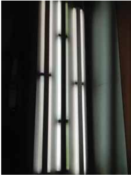
Fig. 2.4.A.15 – T-12 fluorescent luminaires
