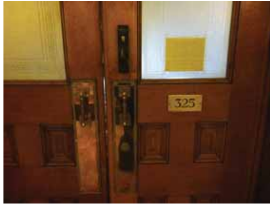
Fig. 3.1.C.52 Areas of tarnishing noted at the historic door knobs.
