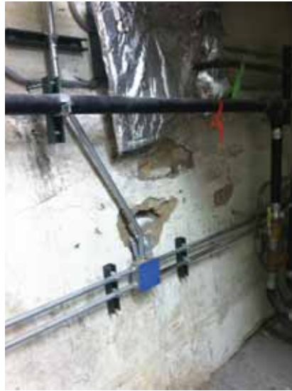
Fig. 3.1.C.27 Spalling and deteriorating concrete walls observed on the Sub-basement Floor.
