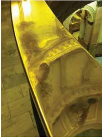
Fig. 3.1.C.55 Areas of tarnishing noted at the brass railings throughout.
