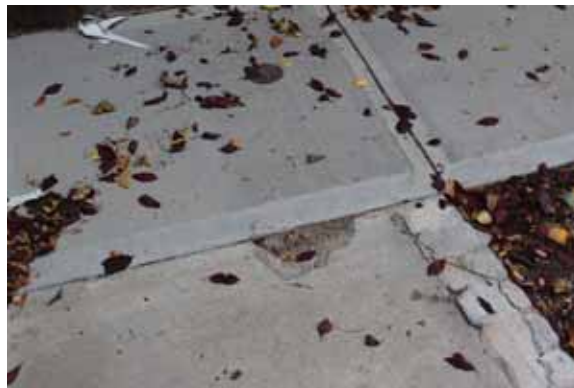
Figure 2.3.A.5 Broken Site Concrete
