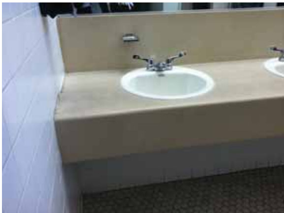
Fig. 3.1.C.57 Countertop in the Men's Restroom in the southeast corner of the Second Floor noted to be aging and worn.
