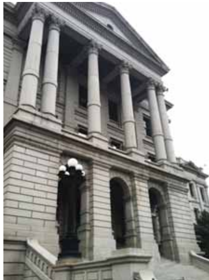
Fig. 2.1.A.6 Soiling noted around the second-story porticos above the monumental entrance porticos.
