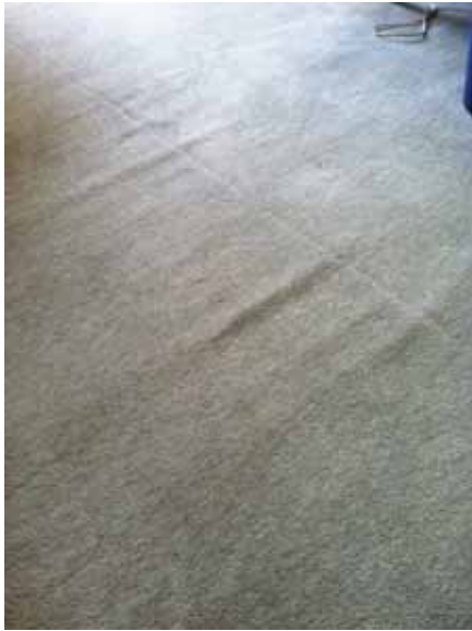
Fig. 3.1.C.39 Areas of carpet coming loose and creating a potential tripping hazard.
