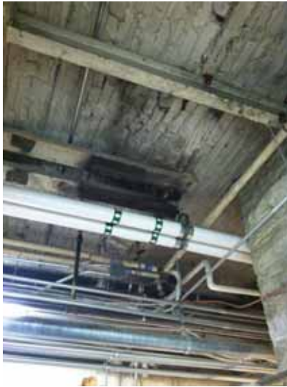
Fig. 3.1.C.5 Areas of deteriorating masonry noted at the ceiling on the Sub-basement Floor.
