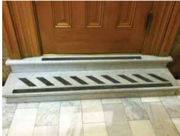
Fig. 2.1.B.4 Location noted where stairs lead directly from a door to a change in floor elevation. Landings are required for code compliance.
