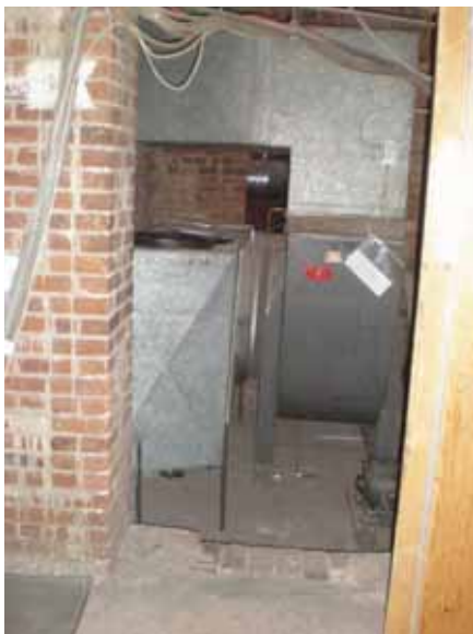
Fig. 2.4.A.44 – Exhaust fan with standard efficiency motor
