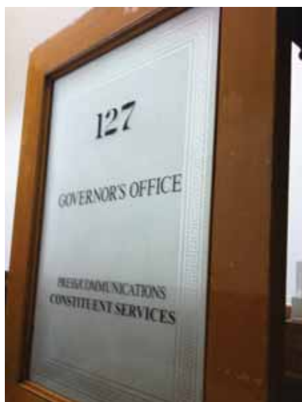
Fig. 3.1.C.51 General wear-and-tear noted at the white oak doors.
