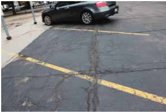
Figure 2.3.A.7 Poor Site Asphalt Condition
