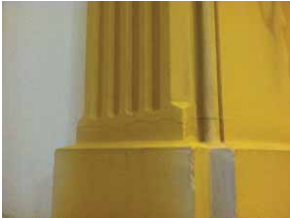
Fig. 3.1.C.12 Typical damage and deterioration noted to the decorative plaster throughout.
