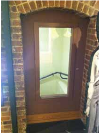
Fig. 3.1.C.24 Deteriorating and damaged brick walls observed in Mr. Brown's Attic.
