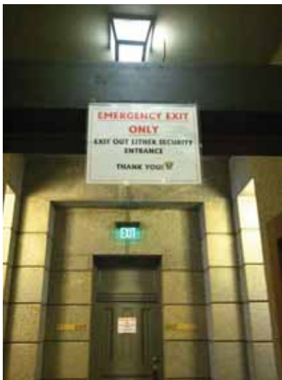
Fig. 2.1.C.12 Inconsistent signage styles observed throughout.
