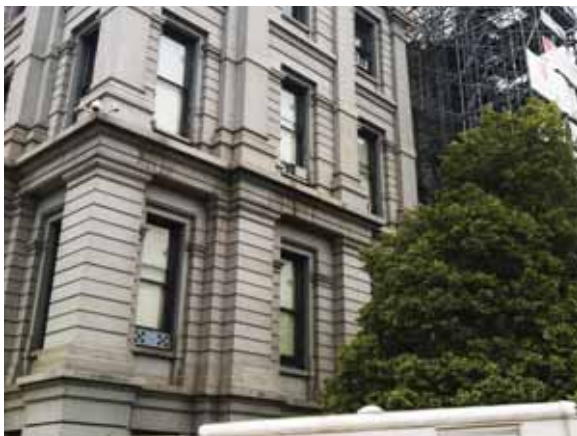
Fig. 2.1.A.4 Generally soiled granite panels noted around the exterior of the building.
