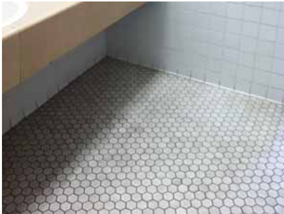
Fig. 3.1.C.46 Generally soiled floor tile observed in the Men's Restroom in the southeast corner of the Second Floor.
