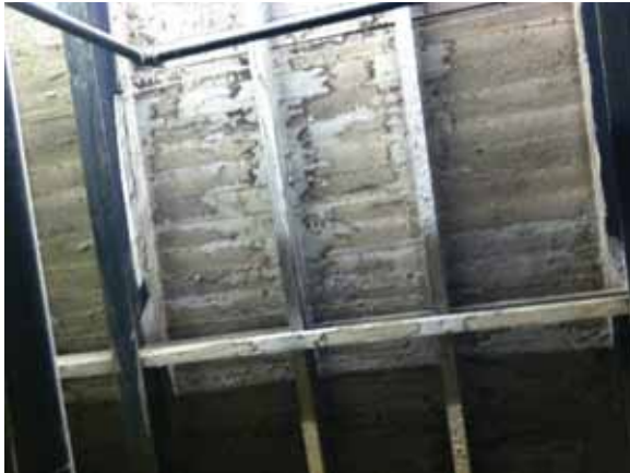
Fig. 2.1.A.23 Signs of water damage observed at the roof throughout the Attic.
