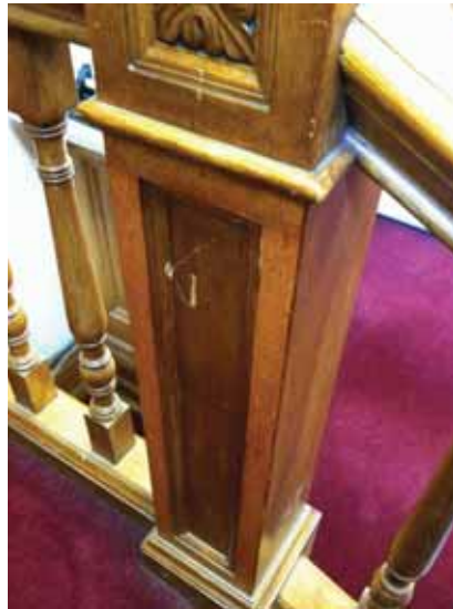
Fig. 3.1.C.53 Damage noted at the wood railing in the room located at the southeast corner of the Senate Gallery.
