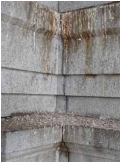
Fig. 2.1.A.9 Soiling caused by the build-up of bird droppings and dirt along the exposed top edges of the granite.
