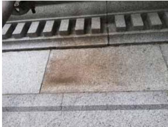
Fig. 2.1.A.5 Generally soiled granite panels noted around the exterior of the building.
