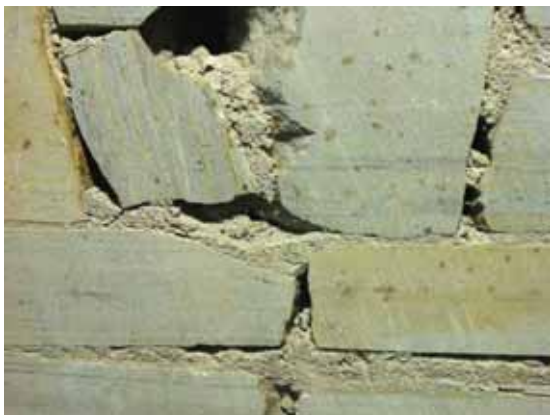
Fig. 3.1.C.26 Spalling stone walls and deteriorating or missing mortar observed on the Sub-basement Floor.
