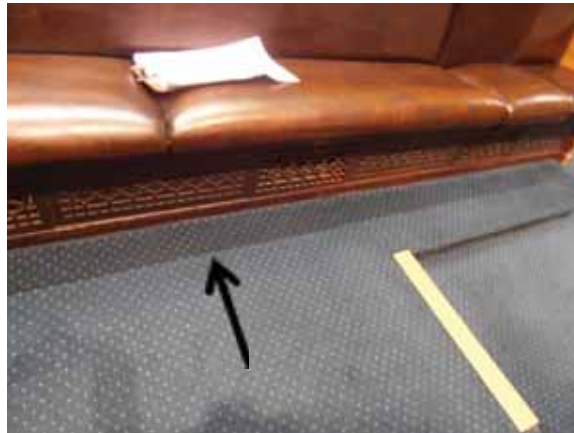
Fig. 2.4.A.28 – Supply air grille
