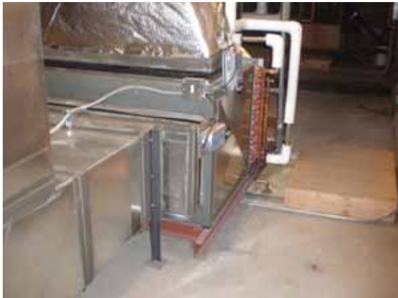
Fig. 2.4.A.25 – Geothermal heat pump
