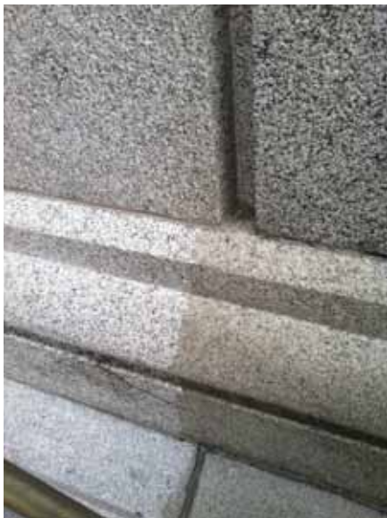
Fig. 2.1.A.15 Test-cleaning of the granite panels was observed to have started on the south end of the east side of the building.
