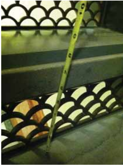
Fig. 2.1.B.6 Height of the stair risers noted in the northwest stairway between the Third Floor and the Attic Floor.
