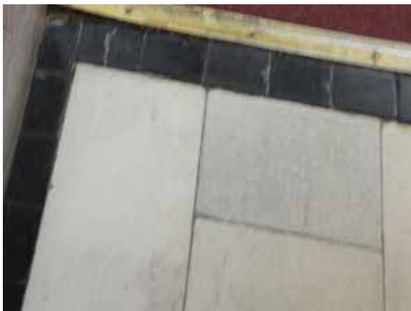
Fig. 3.1.C.35 Cracked and deteriorating black stone flooring border.
