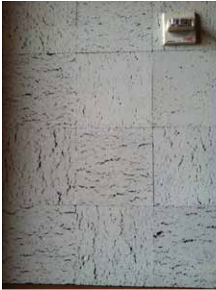
Fig. 3.1.C.18 Acoustic tiles on the walls and ceilings of the Senate Gallery and House of Representatives Gallery.
