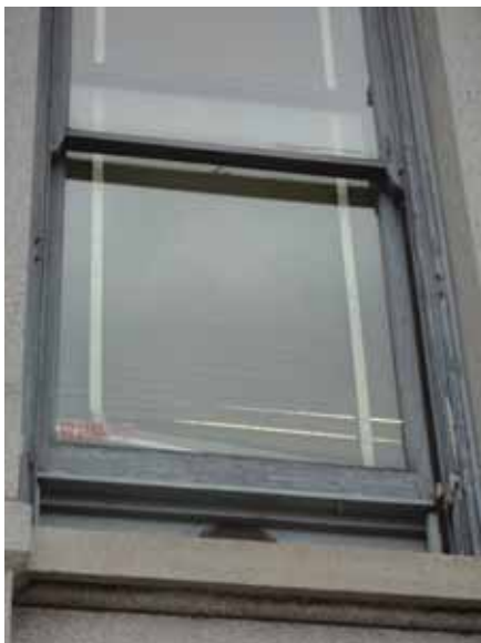
Fig. 2.1.A.16 Generally faded and peeling paint observed at the wood window frames.
