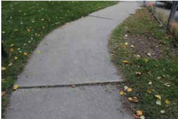
Figure 2.3.B.1 – Settlement in Concrete Along ADA Walkway
