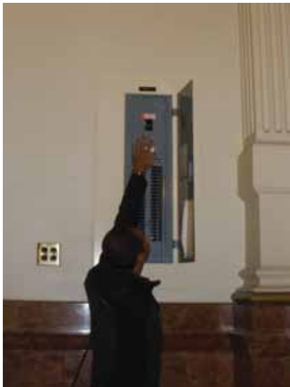
Fig. 2.4.B.4 – Over 7 feet to reach main breaker
