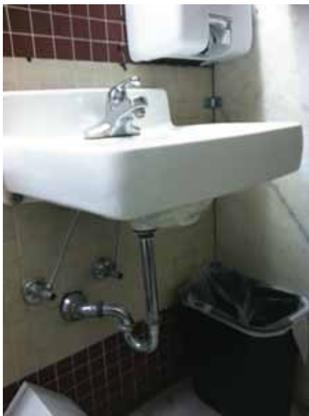
Fig. 2.1.C.2 The accessible lavatory pipes are not insulated within the wheelchair accessible toilet compartments in the public restrooms on the Basement Floor.
