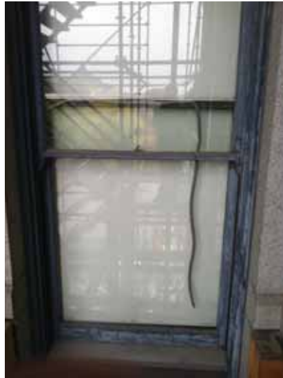
Fig. 2.1.A.17 General deterioration noted at the readily observable windows around the exterior of the building.
