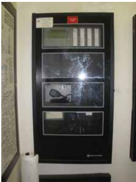
Fig. 2.4.A.19 – Fire alarm control panel
