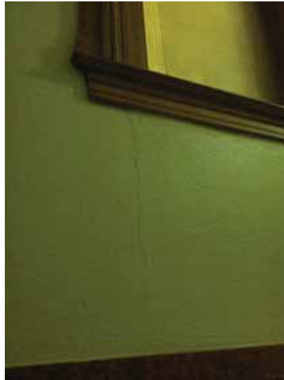
Fig. 3.1.C.9 Cracking plaster noted in areas throughout the building, especially on the Third Floor.
