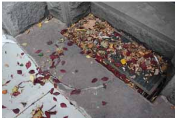
Figure 2.3.A.6 Site Pavement Crack
