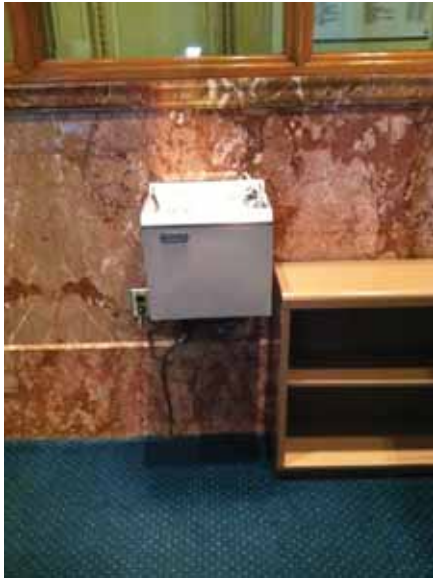
Fig. 2.1.C.6 Non-accessible drinking fountain noted in the House of Representatives Gallery.
