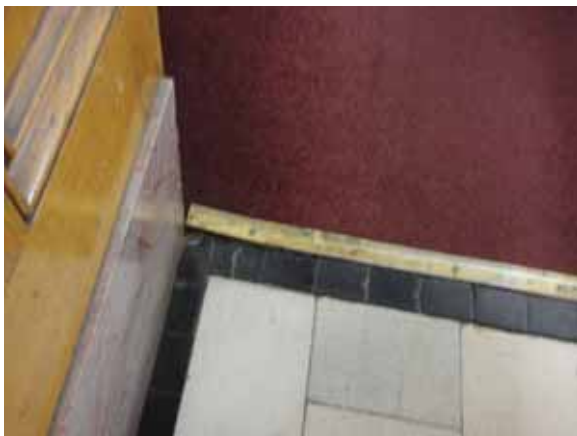
Fig. 3.1.C.41 A threshold coming loose and creating a potential tripping hazard noted during the site survey visit.
