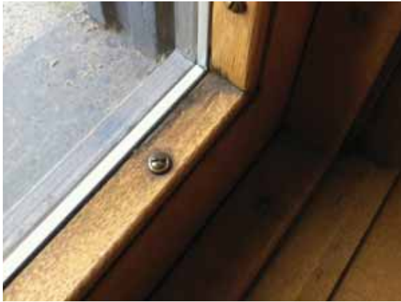
Fig. 2.1.A.20 Evidence of water damage viewed from the interior side of a window.
