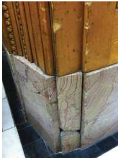
Fig. 3.1.C.16 Areas of damaged and deteriorating stone baseboard and wood wainscoting noted during the site survey visit.
