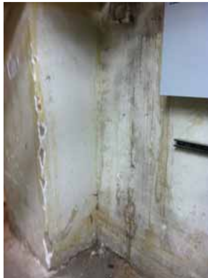
Fig. 3.1.C.28 Evidence of water damage noted in areas throughout the Sub-basement Floor.
