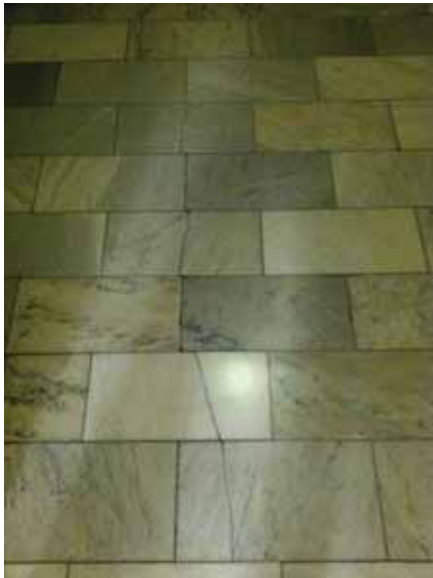
Fig. 3.1.C.34 Cracked and scuffed marble flooring.
