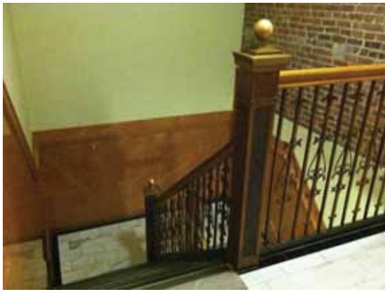
Fig. 2.1.B.7 Handrails currently exist on only one side of the stairs.
