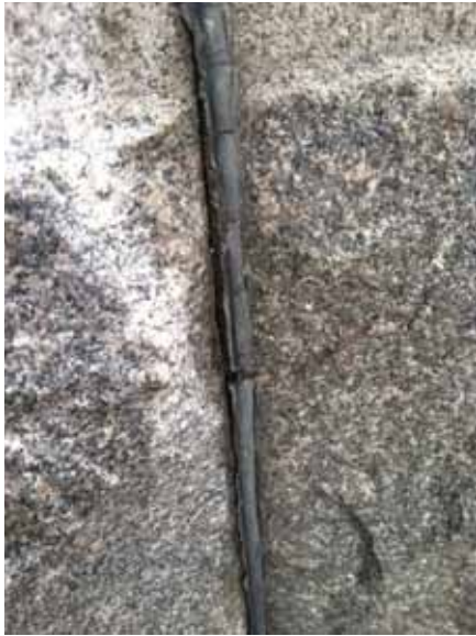
Fig. 2.1.A.14 Widespread deterioration of the material between the joints of the granite panels.
