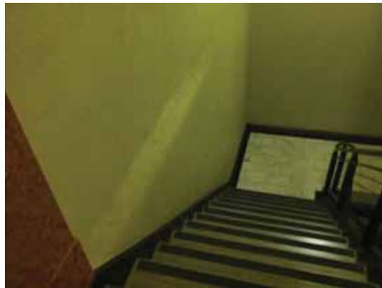
Fig. 3.1.C.10 Area of damaged plaster or gypsum board noted in the northwest stairway between the Basement Floor and the Sub-basement Floor.
