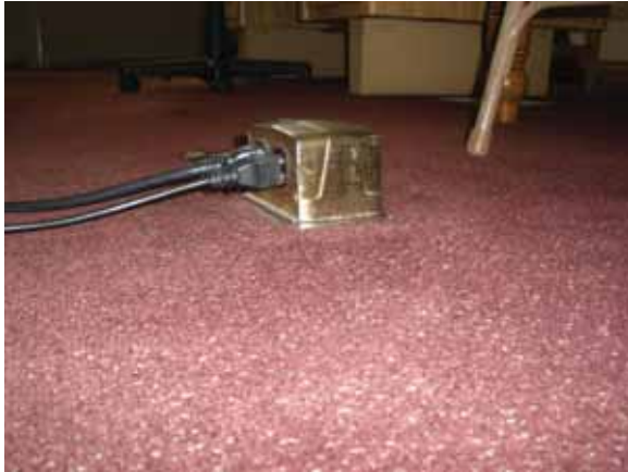
Fig. 2.4.A.23 – Above floor receptacle
