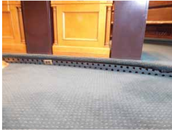
Fig. 2.4.A.45 – Supply air griller
