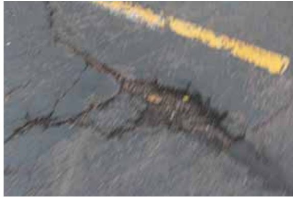
Figure 2.3.A.10 Poor Site Asphalt Condition
