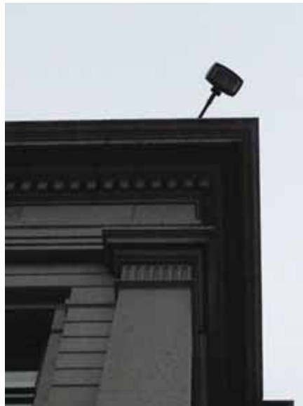
Fig. 2.4.A.17 – Roof mounted luminaires
