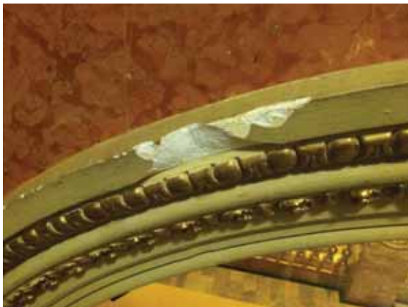
Fig. 3.1.C.14 Damaged decorative plaster noted in the northwest stairway.
