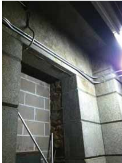
Fig. 3.1.C.21 Water damage noted at the granite cladding on the walls of the west emergency exit vestibule on the Basement Floor.
