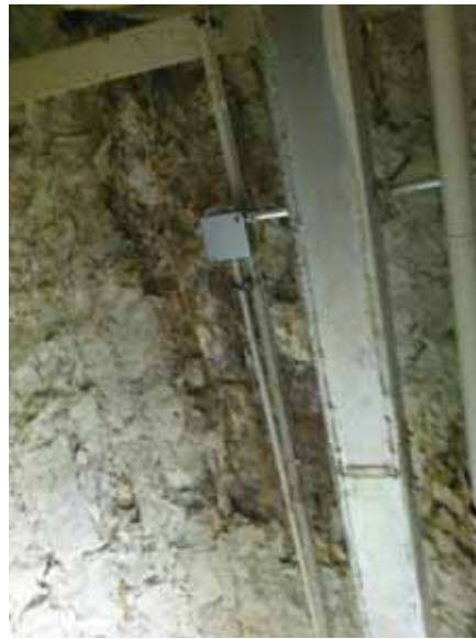
Fig. 3.1.C.8 Evidence of water damage, corrosion, and deterioration at the vaulted masonry ceilings of the areas of the tunnels included in the site survey visit.
