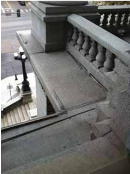
Fig. 2.1.A.2 General soiling and deterioration noted along the top edges of the readily observable sections of the granite ledges.
