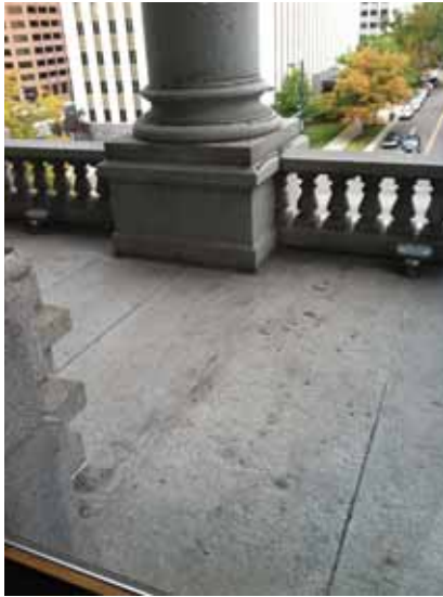
Fig. 2.1.A.8 Evidence of water damage, with spalling of the granite, noted at a readily observable second-story porch above a monumental entrance portico.
