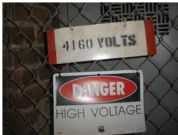
Fig. 2.4.A.1 – Wrong voltage on sign
