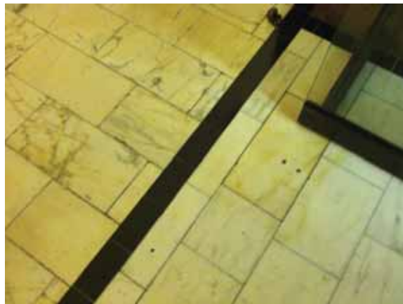
Fig. 3.1.C.31 Areas of soiled stone flooring noted throughout.
