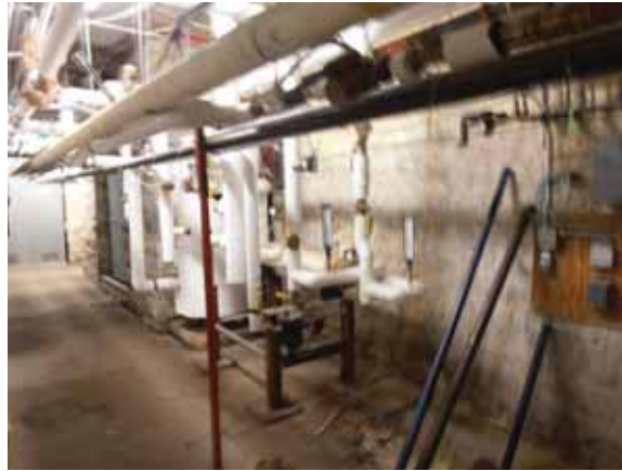
Fig. 2.4.A.33 – Domestic hot water heater
