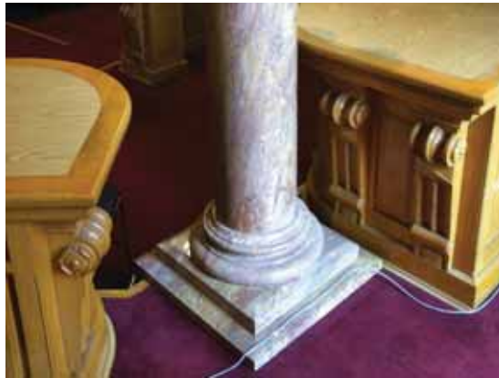
Fig. 3.1.C.43 Electrical cords running loosely across the floor of the Old Supreme Court Chambers and creating a potential tripping hazard.
