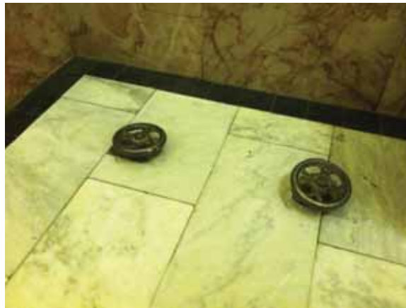
Fig. 3.1.C.37 Two metal valve wheels projecting above the marble flooring and creating a potential tripping hazard on the Second Floor outside of the Offices of the General Assembly.
