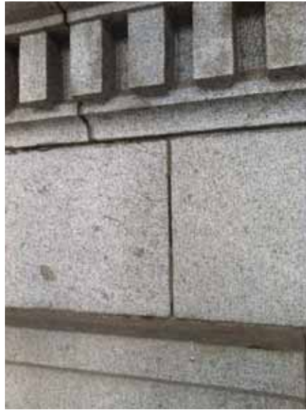
Fig. 2.1.A.11 Widespread deterioration of the material between the joints of the granite panels.
