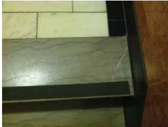
Fig. 3.1.C.36 Cracked stone flooring observed in the northwest stairway.
