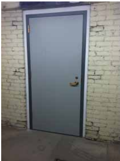
Fig. 3.1.C.25 Damaged and deteriorating brick walls observed on the Sub-basement Floor.
