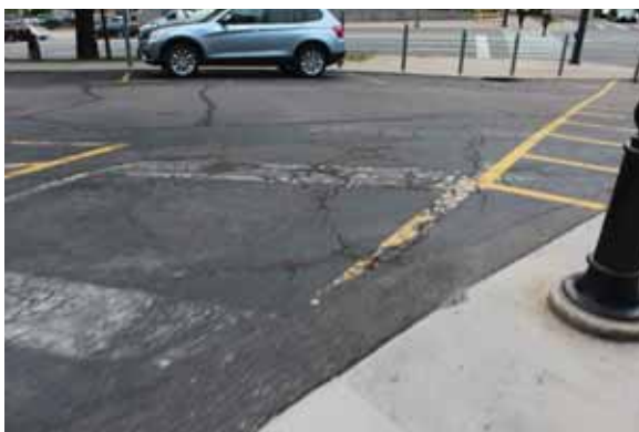
Figure 2.3.A.9 Poor Site Asphalt Condition
