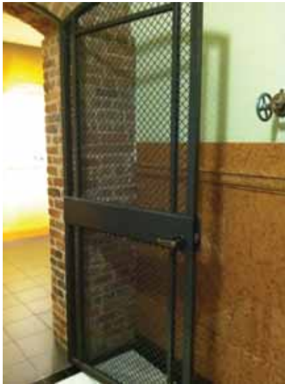
Fig. 2.1.B.2 Non fire-rated doors leading from the northwest and southwest exit stairways to the Attic Floor.
