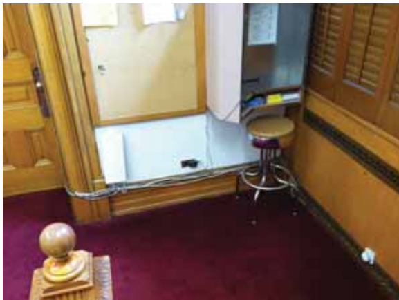
Fig. 3.1.C.56 A bundle of exposed cables run along the base of a wall in a room adjacent to the Senate Gallery.
