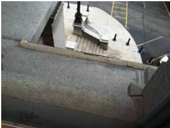
Fig. 2.1.A.3 General soiling and deterioration noted along the top edges of the readily observable sections of the granite ledges.
