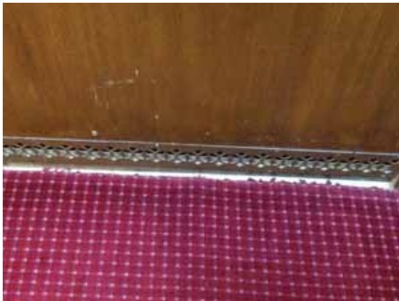
Fig. 3.1.C.40 Areas of carpet flooring observed to be coming loose along the perimeter of the floor.
