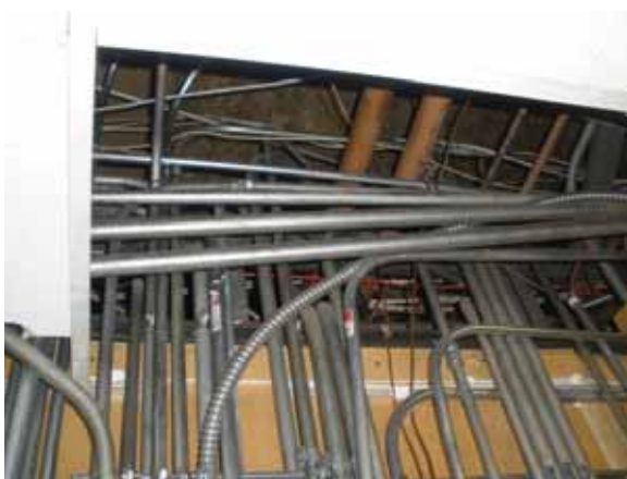
Fig. 2.4.B.1 – No sealed penetrations in electrical room
