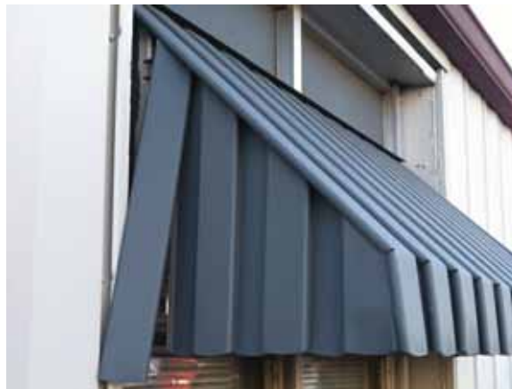
Fig. 2.1.A.11 Damaged and deteriorating metal canopies observed around the exterior of the building.
