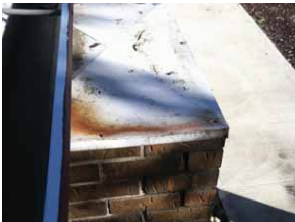
Fig. 2.1.A.9 Corrosion of a metal capping piece noted above a portion of a brick infill wall.
