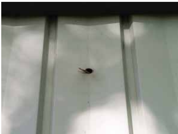
Fig. 2.1.A.3 An unrepaired hole observed with loose wires sticking out.
