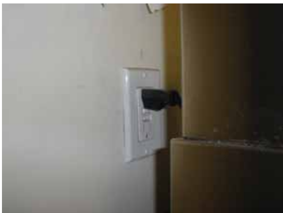
Fig. 2.4.A.13 – Receptacle not connected to wall
