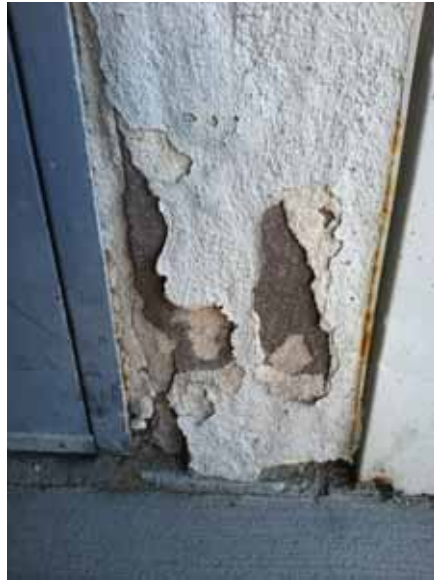
Fig. 2.1.A.21 Deteriorating stucco observed around the door to the visitor's entrance on the west side of the building.
