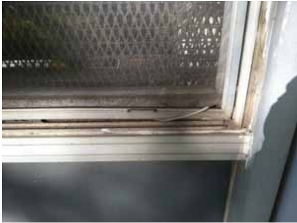
Fig. 2.1.A.31 Typical instance of deteriorating weatherstripping observed at the windows around the exterior of the building.
