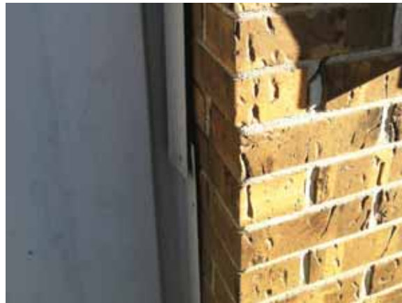
Fig. 2.1.A.4 Metal trim observed to be coming loose around the exterior of the building.
