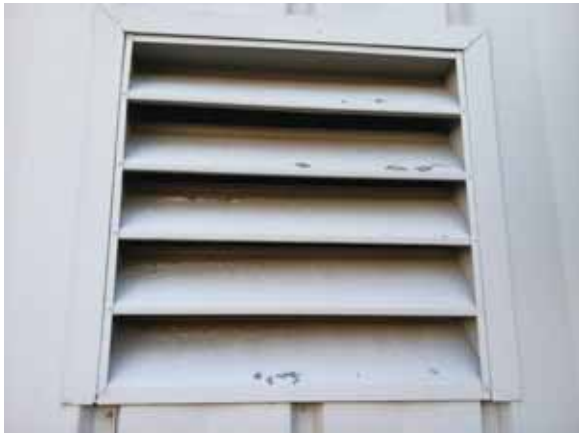
Fig. 2.1.A.19 Peeling paint observed at a metal grille cover.
