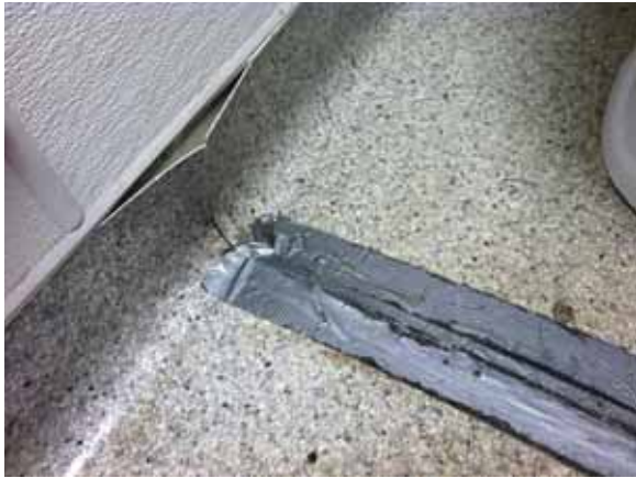
Fig. 3.0.C.26 The vinyl sheet flooring in Room B-9: Women's Restroom is in especially poor condition with deterioration and taped seams observed throughout.
