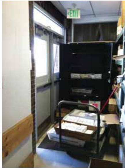
Fig. 2.1.B.1 Items blocking the corridor leading to the northwest exit from the print shop.
