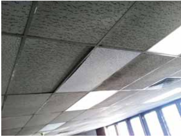
Fig. 3.0.C.1 Sagging, soiled, and deteriorating 2x4 acoustic ceilings observed in areas of the building.
