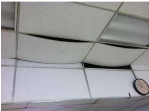
Fig. 3.0.C.3 Sagging of the individual 2x4 acoustic ceiling tiles observed throughout the IDS Print Shop.
