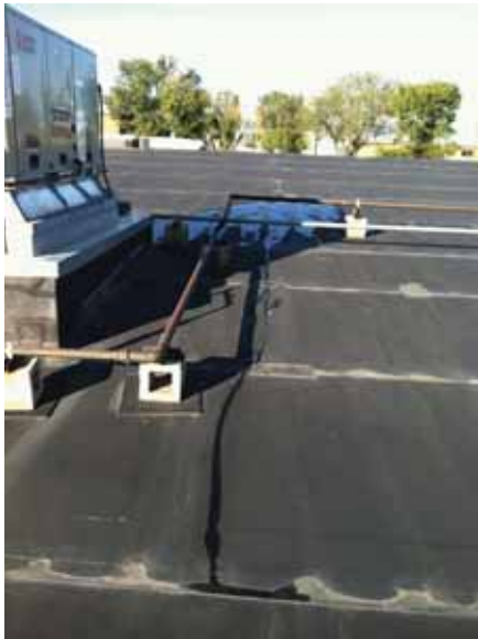
Fig. 2.1.A.45 Areas of standing water observed during the site survey visit.
