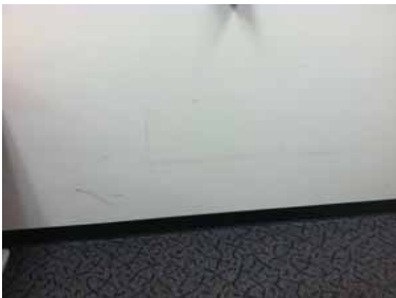
Fig. 3.0.C.13 Typical wear-and-tear noted at the gypsum board walls throughout.
