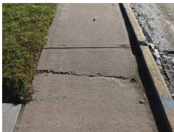
Figure 2.3.A.5 – Site Concrete Crack, Recommended for Replacement
