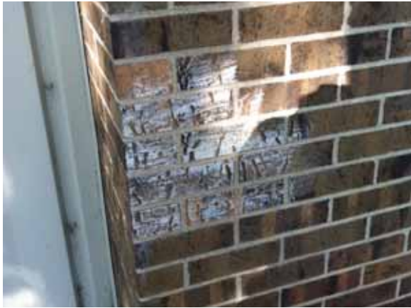
Fig. 2.1.A.18 White residue observed at a brick wall on the east side of the building.
