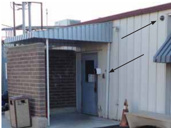
Fig. 2.1.B.13 Key code entry system and intercom/ buzzer system observed at the visitor's entrance on the west side of the building with a security camera noted south of the entrance.
