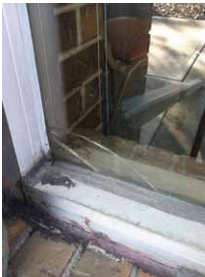
Fig. 2.1.A.27 Broken glass observed at a few windows, especially along the east side of the building.
