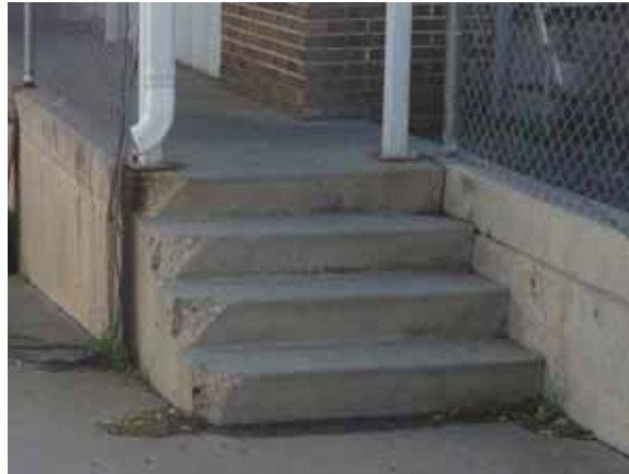
Fig. 2.1.B.8 The stairway at the northwest loading dock is not equipped with handrails as required by code.
