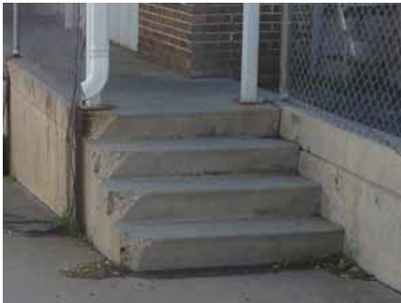
Fig. 2.1.A.49 Spalling concrete observed at the exterior stairway at the northwest loading dock.
