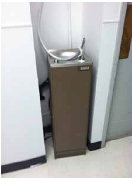
Fig. 2.1.C.1 Typical non-accessible drinking fountain observed throughout the building and loose tubing observed on top of the fountain.
