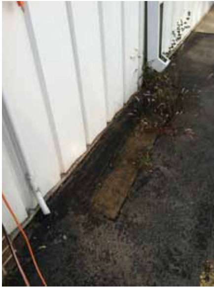
Fig. 2.1.A.53 A corroding metal panel embedded within the asphalt observed near the back (north side) of the building.
