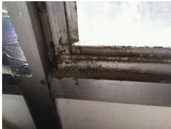
Fig. 2.1.A.28 Evidence of deterioration and water intrusion observed on the interior side of the windows.
