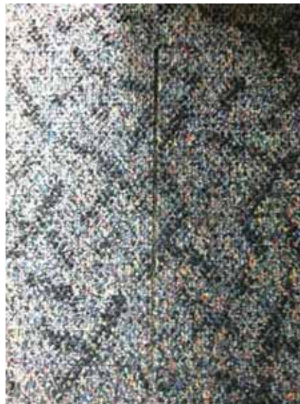
Fig. 3.0.C.30 Deterioration of the carpet seams observed during the site survey visit are creating a potential tripping hazard.
