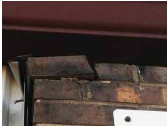
Fig. 2.1.A.16 Areas of damaged and deteriorating brick and mortar observed around the exterior of the building.
