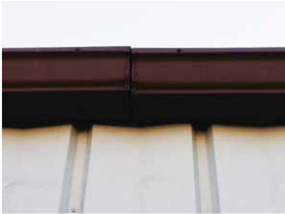
Fig. 2.1.A.7 Corrosion observed at the top of the metal panels around the exterior of the building.
