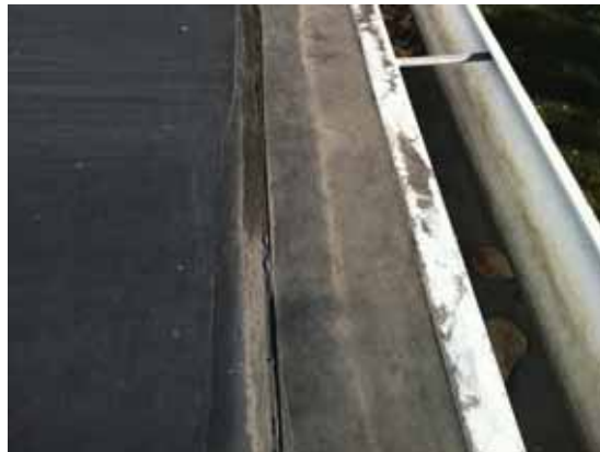
Fig. 2.1.A.42 Typical instance of sealant missing entirely along the seams of the rubber membrane and exposing the roof system to water penetration.
