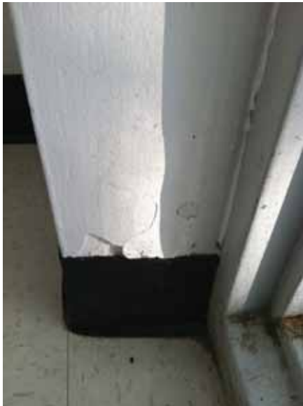
Fig. 3.0.C.12 Deterioration of the gypsum board observed during the site survey visit.
