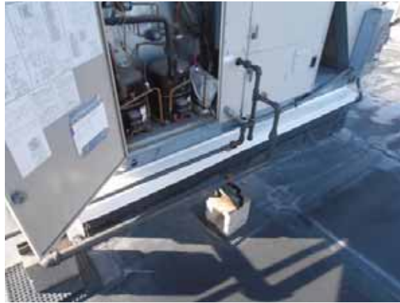
Fig. 2.4.A.20 – Gas piping connection at RTU
