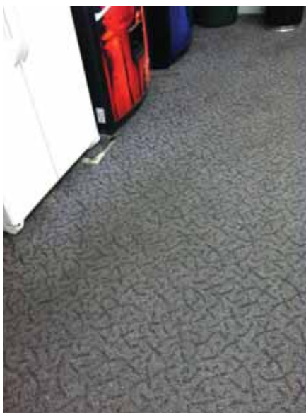
Fig. 3.0.C.28 General deterioration and soiling observed at the carpet flooring throughout.
