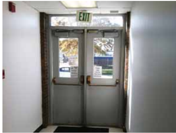
Fig. 3.0.C.34 An inadequately secured exit sign observed at the exit on the east end of the south side of the building poses a life-safety hazard to building occupants who pass underneath.
