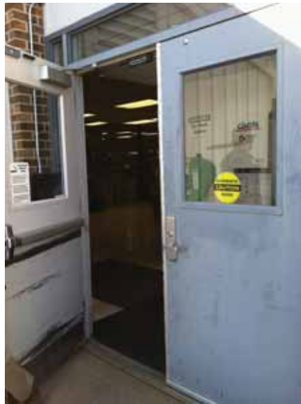
Fig. 2.1.A.34 General wear-and tear noted to the inside and outside face of the exterior doors around the building.
