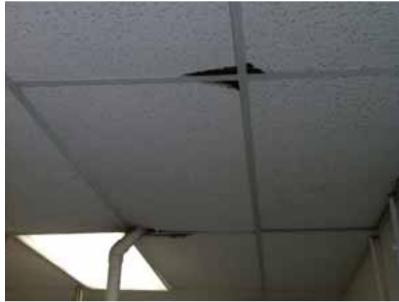
Fig. 3.0.C.4 Typical instance of deterioration of the 2x4 acoustic ceiling observed during the site survey visit.
