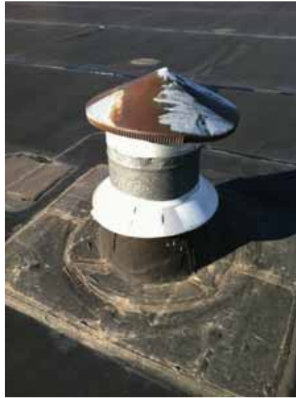
Fig. 2.1.A.47 Evidence of corrosion noted at a roof vent cover.
