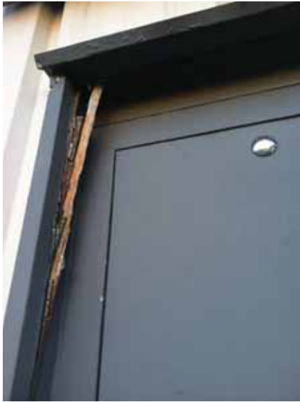
Fig. 2.1.A.35 Deterioration of the door frame noted at a door located on the west side of the building to the north of the visitor's entrance.
