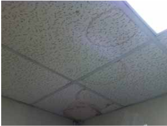
Fig. 3.0.C.7 Typical instance of soiled and deteriorating 2x4 acoustic ceiling tiles with evidence of water damage observed throughout the building.
