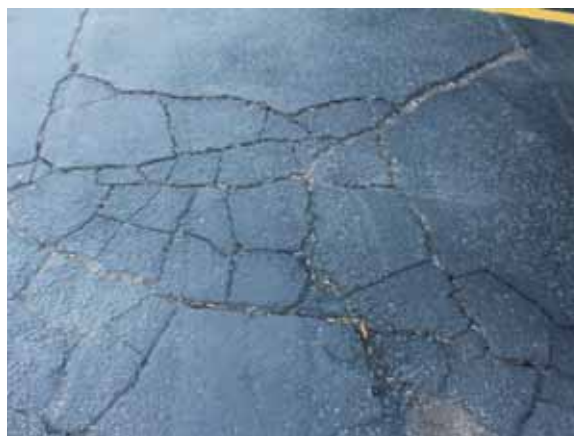
Figure 2.3.A.6 – Poor Site Asphalt Condition
