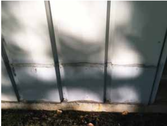
Fig. 2.1.A.1 Deteriorating areas of previously repaired metal panels observed around the exterior of the building.
