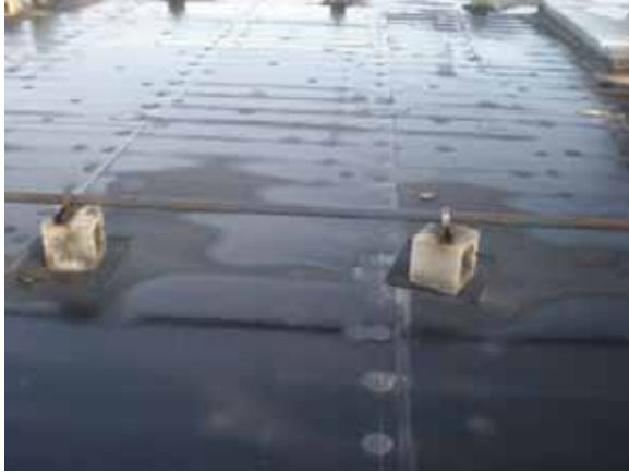
Fig. 2.4.A.17 – Gas piping on roof
