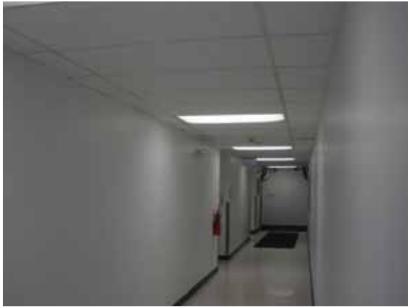
Fig. 2.4.A.7 – Hallway lensed luminaires
