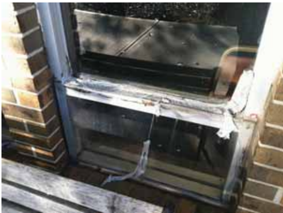
Fig. 2.1.A.32 Duct tape appears to have been applied along the base of a few windows on the east side of the building in a likely attempt to mitigate the issues with the deteriorating sealant and weatherstripping.
