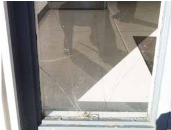
Fig. 2.1.A.39 Cracked glass observed at the sidelight south of the pair of doors on the north end of the east side of the building.
