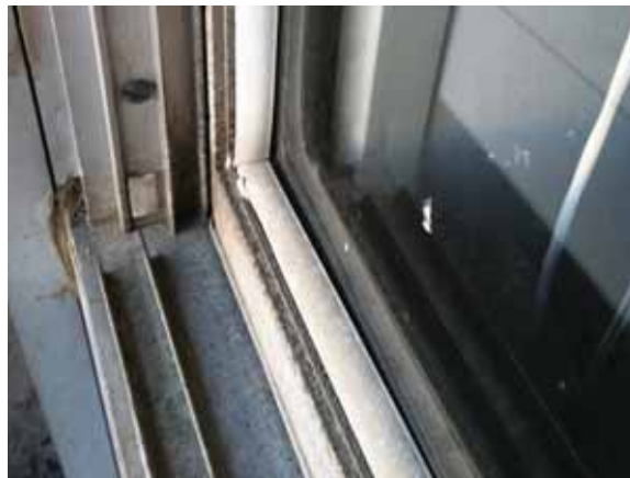
Fig. 2.1.A.24 General deterioration of the window frames noted around the exterior of the building.
