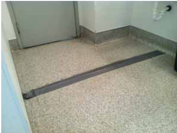
Fig. 3.0.C.27 The deterioration of the seams of the vinyl sheet flooring in Room B-9: Women's Restroom is creating a potential tripping hazard.
