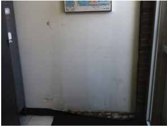
Fig. 3.0.C.11 Wear-and-tear and cracking of the gypsum board wall observed in the northeast entry vestibule.
