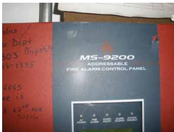
Fig. 2.4.A.10 – Fire alarm control panel
