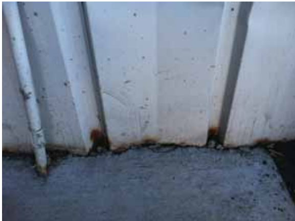
Fig. 2.1.A.8 Corrosion observed at the base of the metal panels around the exterior of the building.
