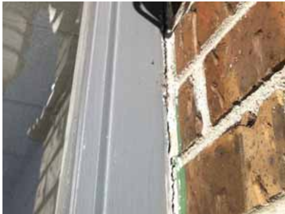
Fig. 2.1.A.36 Deterioration of the sealant noted at the door assembly on the south end of the east side of the building leading to the exterior courtyard.
