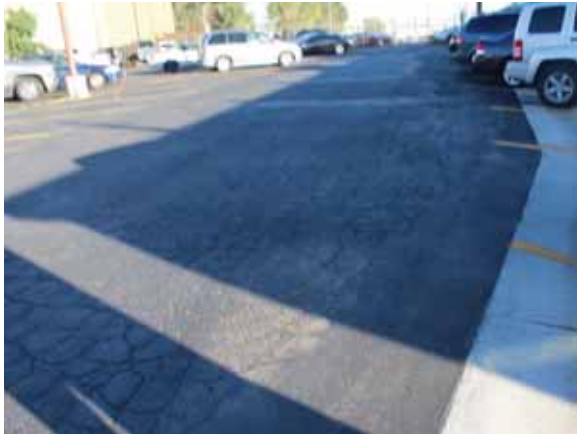
Figure 2.3.A.7 – Poor Site Asphalt Condition
