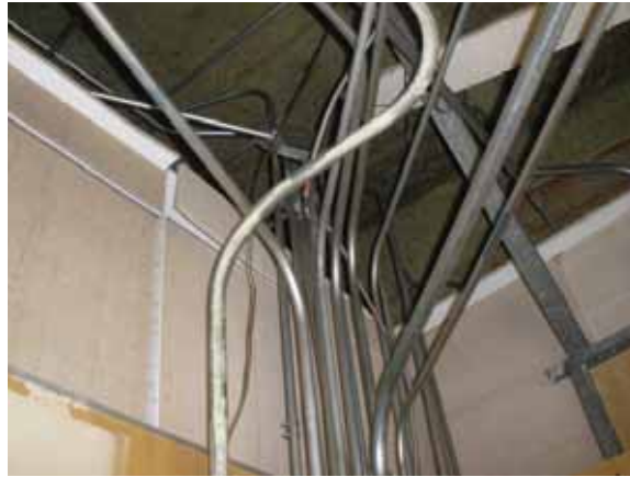
Fig. 2.4.B.2 – No sealed penetrations in electrical room
