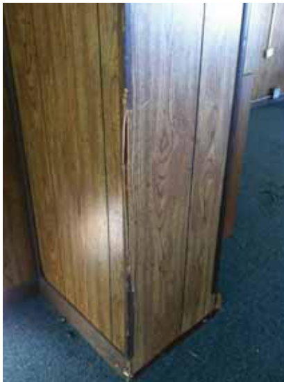
Fig. 3.0.C.17 General wear-and-tear and damage noted to the laminated wood paneling throughout the areas included in the site survey visit.
