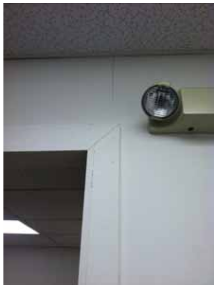
Fig. 3.0.C.15 Cracking of the gypsum board walls observed above some of the door openings throughout.
