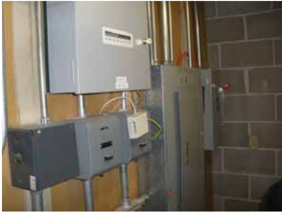
Fig. 2.4.A.3 – Main electrical room panelboards
