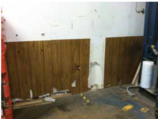
Fig. 3.0.C.18 Extensive damage to the laminated wood paneling wainscoting and the gypsum board wall observed in the north loading dock and storage room.
