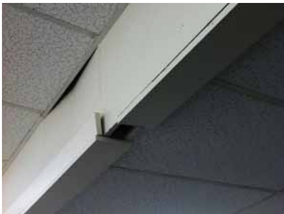
Fig. 3.0.C.9 Cracked and damaged material covering a beam observed at the ceiling in the office space located at the southern central portion of the building.
