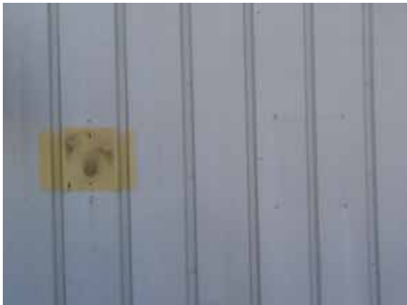
Fig. 2.1.A.2 Unrepaired holes leaving the building envelope vulnerable to water penetration and discoloration of the metal panels observed in areas around the exterior of the building.
