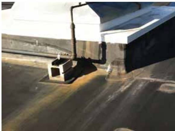
Fig. 2.1.A.46 Corrosive dust observed on the rubber roofing membrane near metal equipment and roof components.
