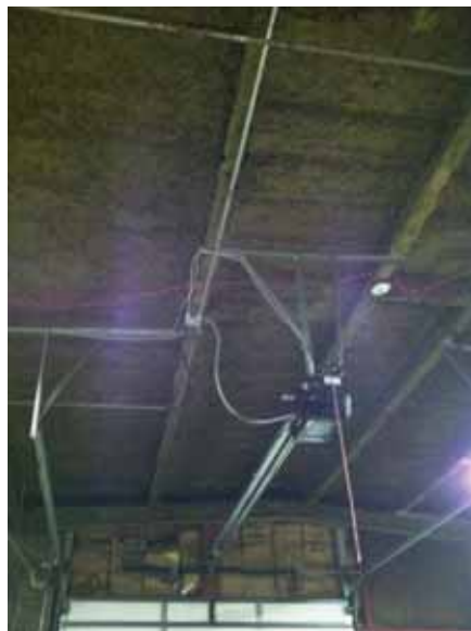
Fig. 3.0.C.10 Open ceiling observed with deteriorating spray-on insulation in the north loading dock and storage room.
