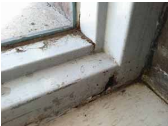
Fig. 2.1.A.37 Evidence of water damage observed on the interior side of the sidelight of the door and sidelight assembly on the south end of the east side of the building.
