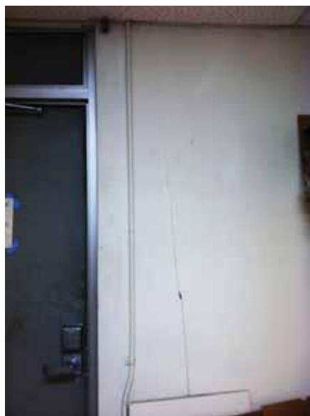
Fig. 3.0.C.14 A cracked section of the gypsum board wall observed near the Oil & Gas Lab exit door on the south side of the building.
