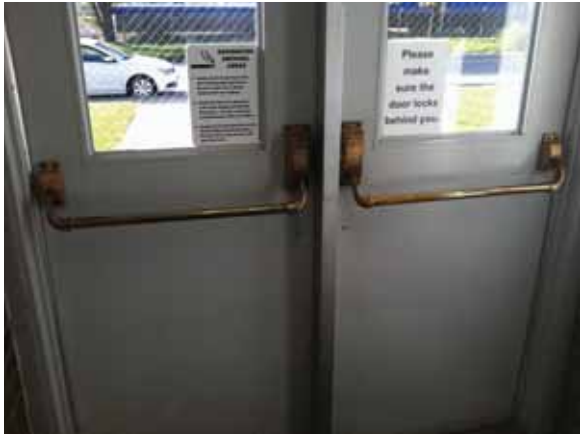
Fig. 2.1.B.17 Signs on the interior side of the emergency exits reminding employees to ensure that the doors lock upon exiting.
