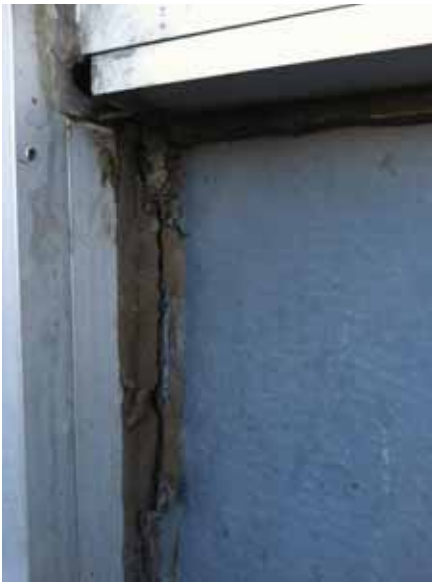
Fig. 2.1.A.13 Sealant observed to be deteriorating or missing entirely around the edges of the transite panels.
