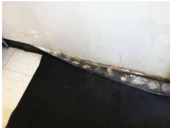
Fig. 3.0.C.20 Deteriorating vinyl baseboard observed in areas throughout the building.
