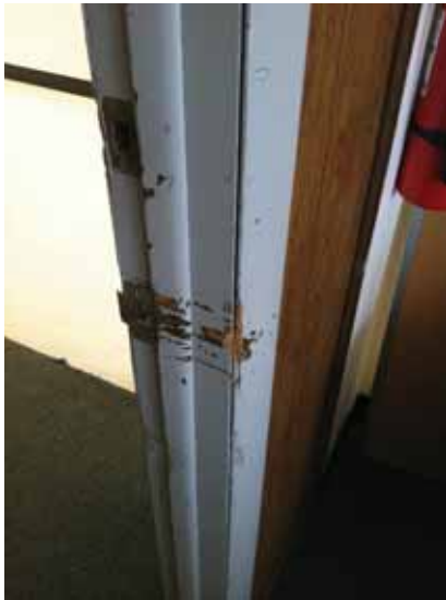
Fig. 3.0.C.32 Wear-and-tear observed at a door frame during the site survey visit.
