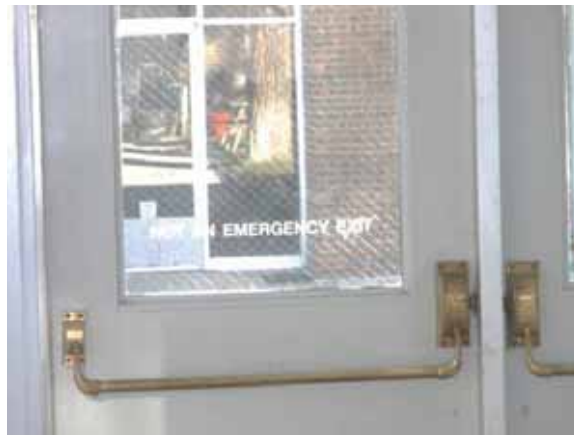
Fig. 2.4.B.3 – “Not an emergency exit” labeling
