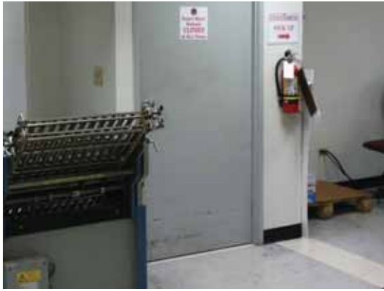
Fig. 3.0.C.31 General wear-and-tear observed at the doors throughout.
