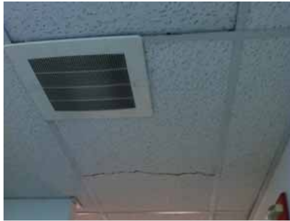
Fig. 3.0.C.5 Typical instance of a cracked 2x4 acoustic ceiling tile observed during the site survey visit.
