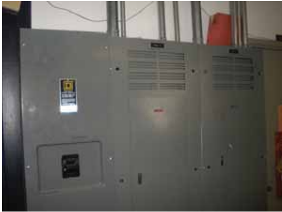
Fig. 2.4.A.4 – Secondary electrical room
