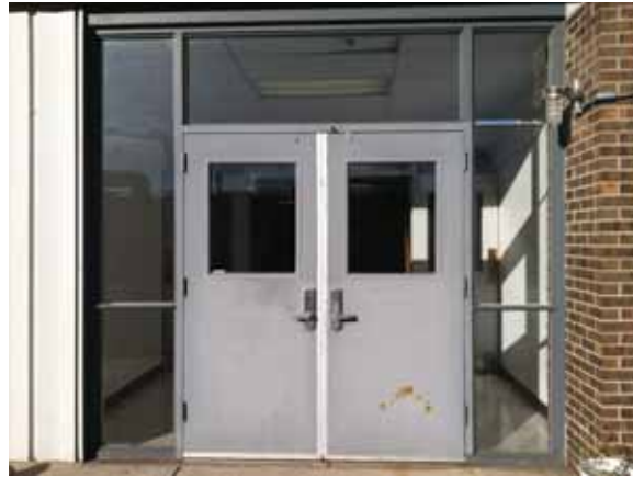
Fig. 2.1.A.38 Evidence of corrosion observed at the pair of doors on the north end of the east side of the building.
