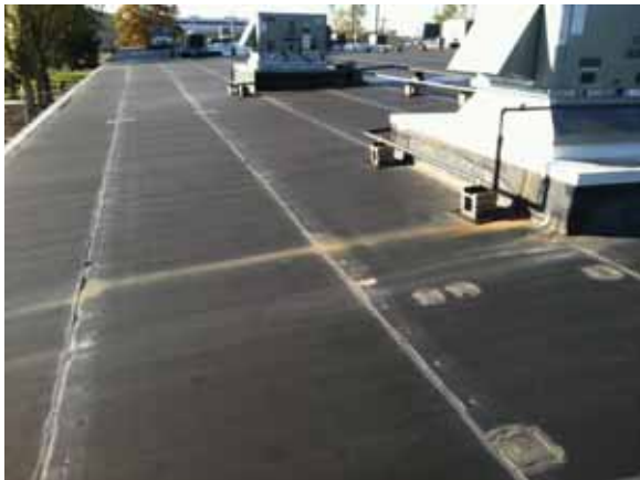
Fig. 2.1.A.40 Rubber membrane roof in fair to poor condition overall.
