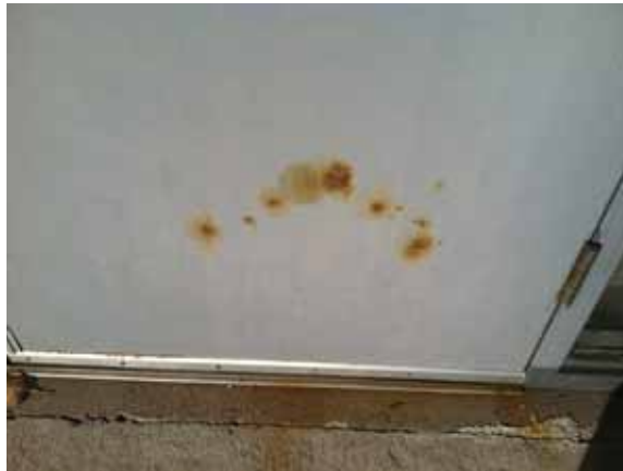
Fig. 2.1.A.51 Deterioration of the concrete paver observed along the base of the doors on the north end of the east side of the building.
