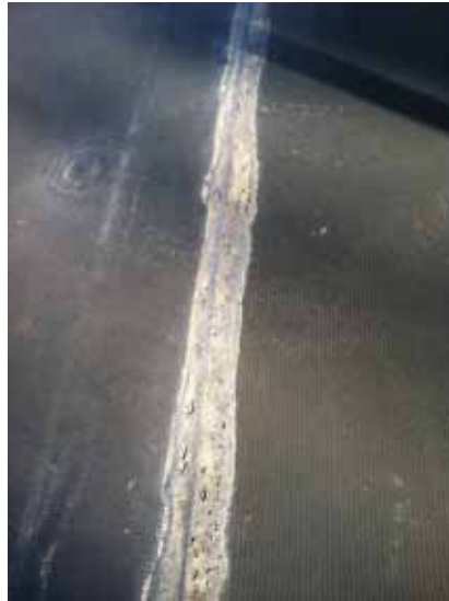
Fig. 2.1.A.41 Typical instance of deteriorating sealant along the seams of the rubber roofing membrane.
