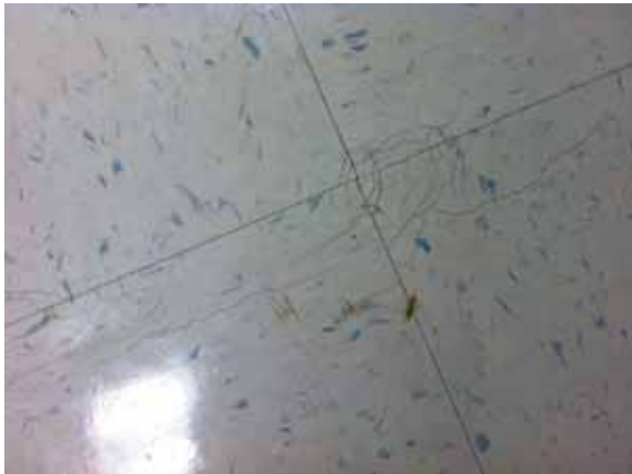
Fig. 3.0.C.21 Damaged vinyl tile flooring observed throughout the building.
