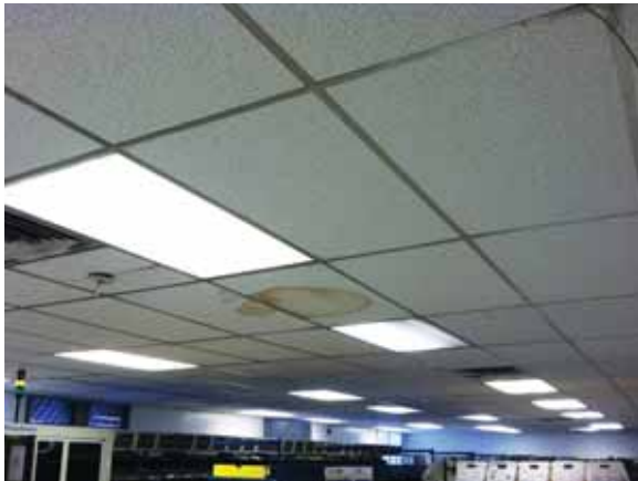
Fig. 3.0.C.8 Soiled and deteriorating 2x4 acoustic ceiling tiles with evidence of water damage observed in the IDS Print Shop.
