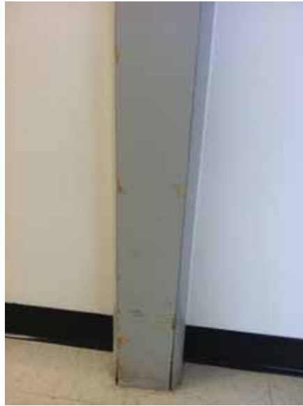
Fig. 3.0.C.19 General wear-and-tear to the wood trim observed in areas throughout the building.
