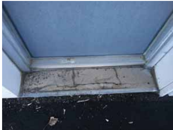
Fig. 2.1.A.22 Cracked and spalling concrete observed along the building's foundation.
