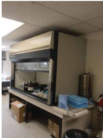
Fig. 2.4.A.21 – Fume hood in lab
