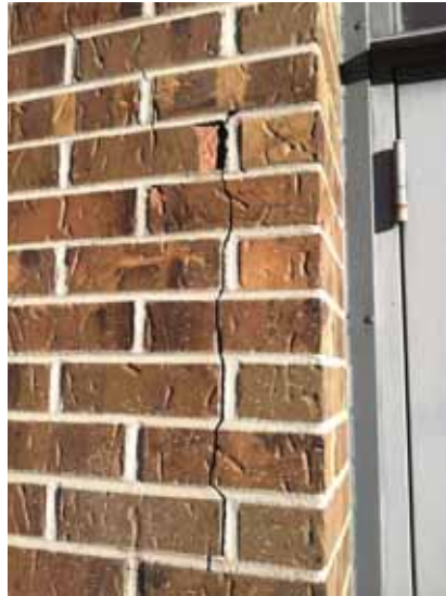
Fig. 2.1.A.15 Areas of damaged and deteriorating brick and mortar observed around the exterior of the building.
