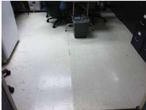
Fig. 3.0.C.24 An area of the vinyl tile flooring observed to be buckling during the site survey visit.
