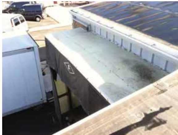
Fig. 2.1.A.48 The top of the canopy at the northeast corner of the building was observed to be generally soiled and to have deteriorating sealant along the wall of the building.
