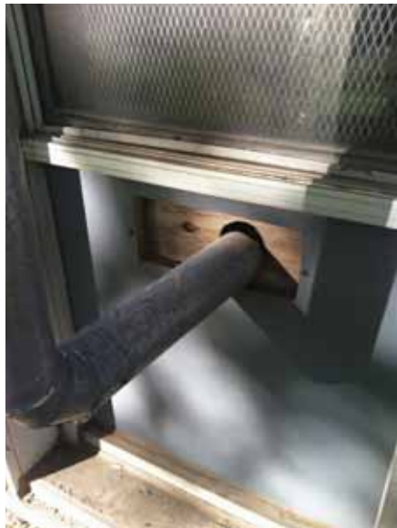
Fig. 2.1.A.14 An improperly waterproofed hole created through a transite panel which may be exposing the asbestos fibers within the panel.
