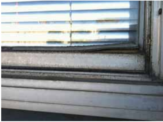
Fig. 2.1.A.25 General deterioration of the window frames noted around the exterior of the building.
