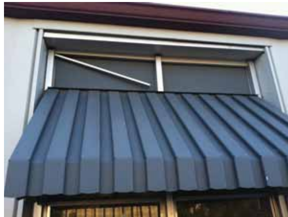
Fig. 2.1.A.5 Metal trim observed to be coming loose around the exterior of the building.
