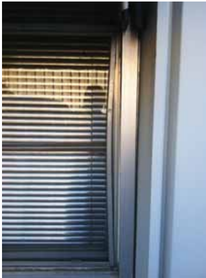
Fig. 2.1.A.26 General deterioration of the window frames noted around the exterior of the building.
