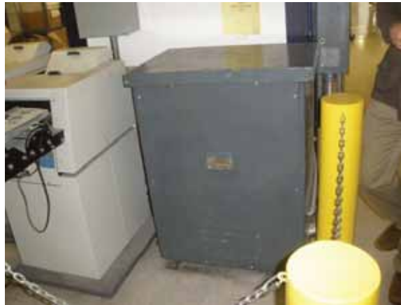
Fig. 2.4.A.17 – Transformer in printing area
