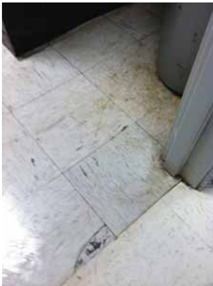
Fig. 3.0.C.22 Deteriorating and soiled vinyl tile flooring observed throughout the building.
