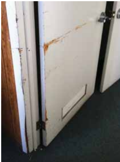
Fig. 3.0.C.33 Extensive damage observed at a wood door and frame during the site survey visit.
