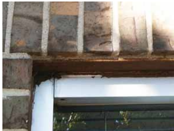
Fig. 2.1.A.29 Corrosion observed at a metal header above a window on the east side of the building.
