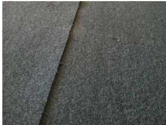
Fig. 3.0.C.29 Carpet seams that have come loose and are creating a potential tripping hazard.
