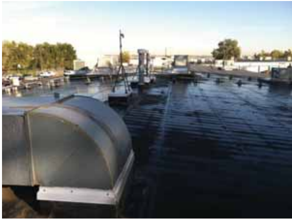
Fig. 2.1.A.44 Large areas of the roof observed to be wet at the time of the site survey visit.
