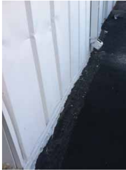
Fig. 2.1.A.10 Damaged metal panels observed along parking and loading dock areas around the exterior of the building.
