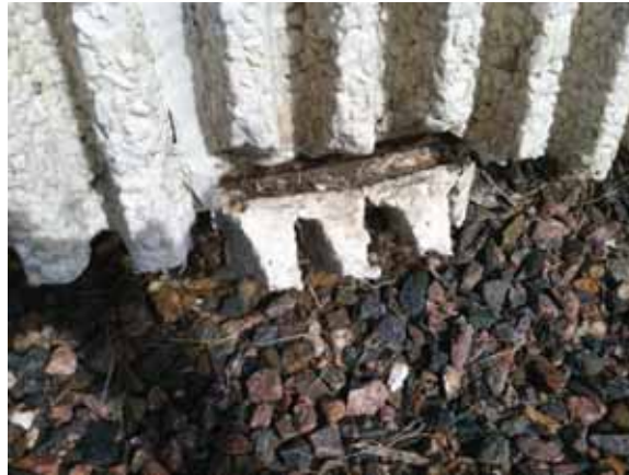
Fig. 2.1.A.2 Damaged areas of the precast aggregate panels noted around the building.
