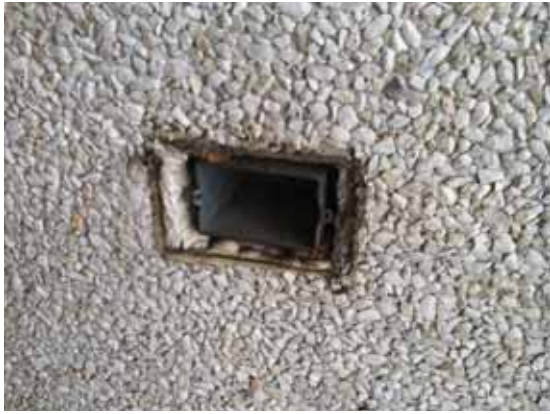
Fig. 2.1.A.16 Exposed empty electrical outlet box at the exterior porch on the east side of the building.
