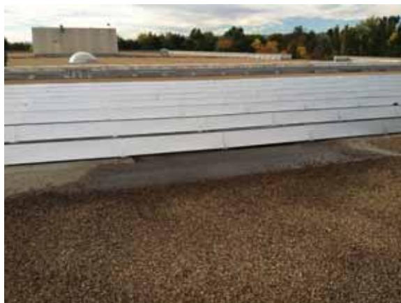
Fig. 2.1.A.43 Areas of pooling water noted around the roof.
