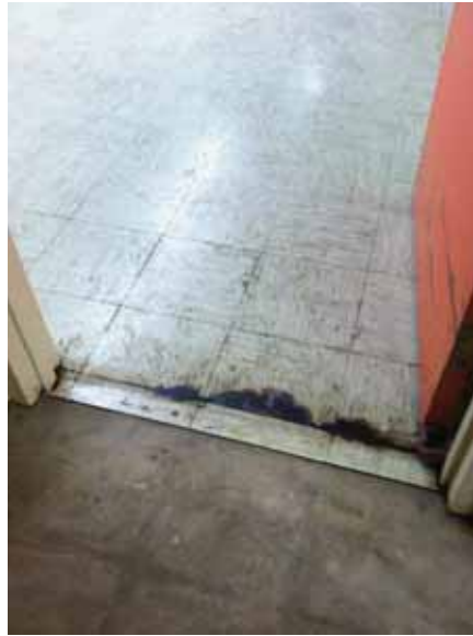
Fig. 3.0.C.30 Damaged and soiled linoleum flooring noted on the Basement Floor.
