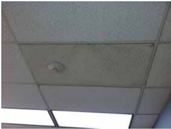
Fig. 3.0.C.5 Acoustic ceiling tiles do not appear to have been updated or replaced during the recent remodeling of Room 118 or in other remodeled spaces included in the site survey.
