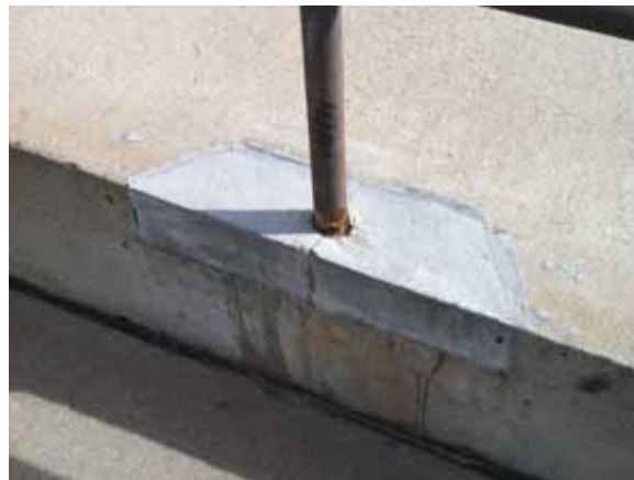
Fig. 2.1.A.67 Cracked concrete causing the corroding guardrail posts to become loose along the ramp to the South Employee Entrance.
