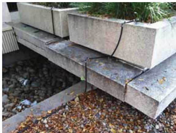
Fig. 2.1.A.56 Cracked aggregate beam and aggregate beams pulling away from the north side of the raised platform at Entrance B.
