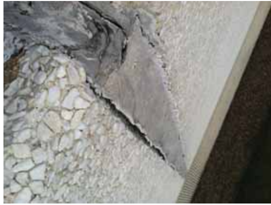
Fig. 2.1.A.19 Deterioration of the sealant between the precast panels.
