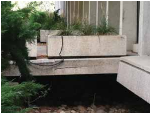
Fig. 2.1.A.58 Cracked aggregate beam and aggregate beams pulling away from the south side of the raised platform at Entrance B.
