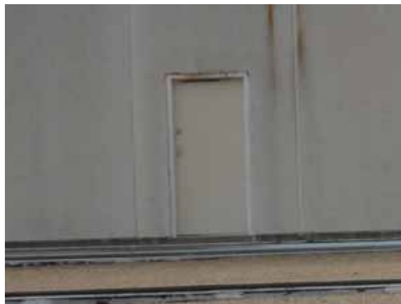
Fig. 2.1.A.40 Corroding frame around the door to the South Penthouse.
