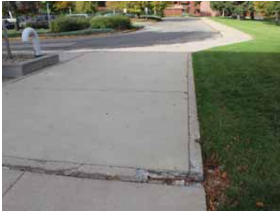
Figure 2.3.A.12 Broken Site Concrete, Recommended for Replacement
