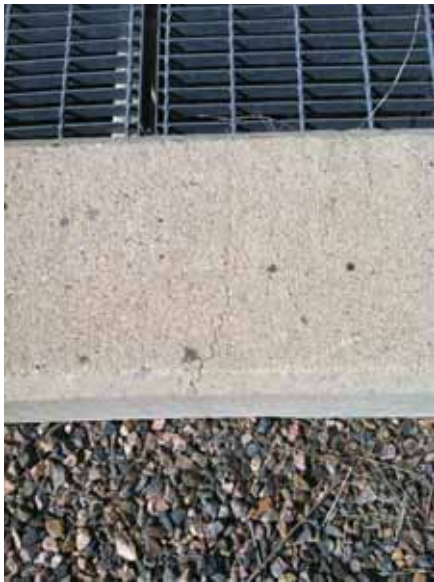
Fig. 2.1.A.76 Cracked concrete at a low window well wall.
