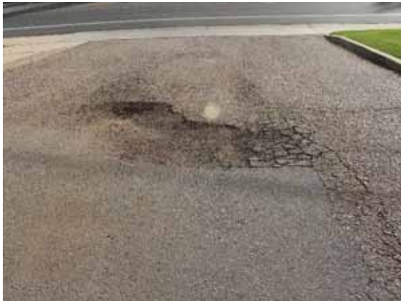
Figure 2.3.A.18 Poor Site Asphalt Condition
