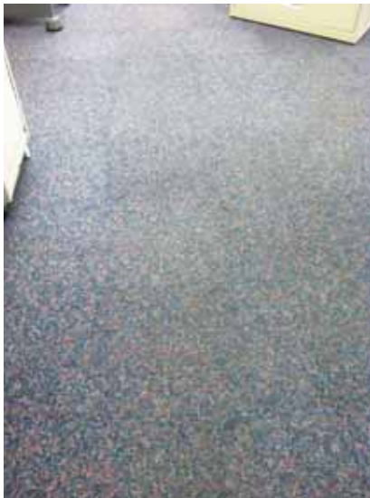
Fig. 3.0.C.23 Typical instance of worn and soiled carpet noted on the First Floor of the south wing.
