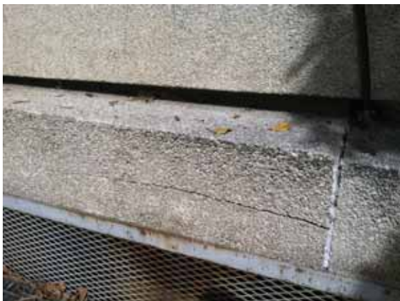
Fig. 2.1.A.59 Cracked aggregate beam at the raised platform at the East Employee Entrance.
