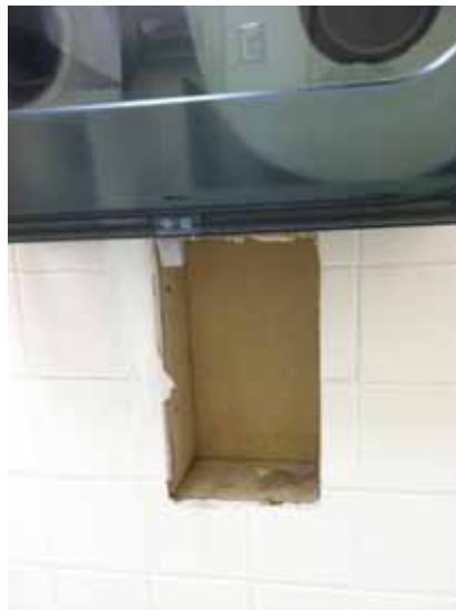
Fig. 3.0.C.17 Unrepaired hole from a former toilet paper dispenser in the Men's and Women's Restrooms at the northeast corner of the south wing.
