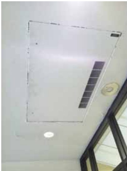
Fig. 3.0.C.6 Water damage at the gypsum board ceiling around the ceiling panel in the vestibule of Entrance B.
