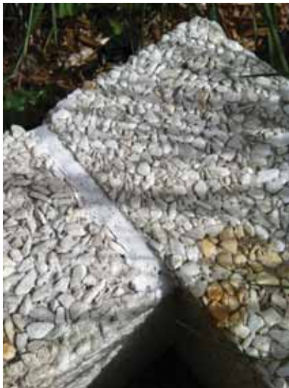
Fig. 2.1.A.18 Soiled precast aggregate wall with deteriorating sealant at the outside edge of the exterior porch.
