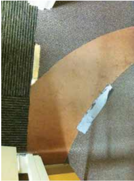
Fig. 3.0.C.28 Typical instance of tape placed over damaged portions of the original carpet in the north wing known to have asbestos in the mastic. This is also creating a potential tripping hazard.
