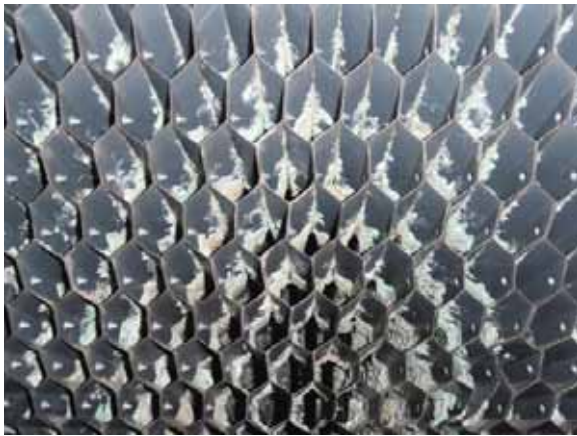
Fig. 2.4.A.22 – Cooling tower fill material
