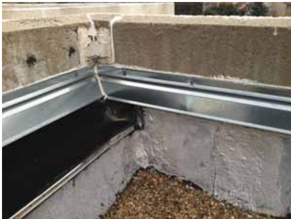
Fig. 2.1.A.28 Deterioration of the concrete parapet around a corroding metal corner connection.
