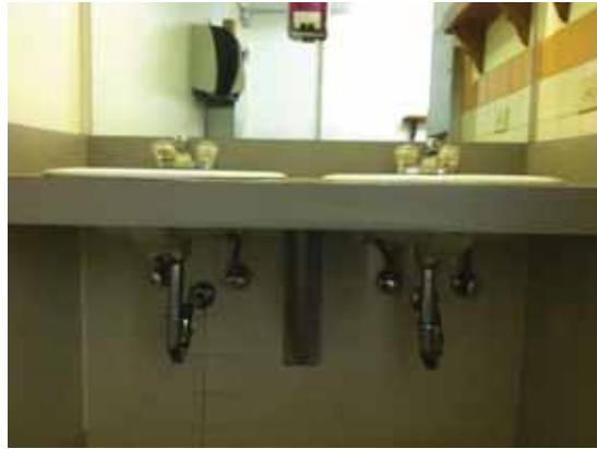
Fig. 2.1.C.3 Lavatories with knob-style faucet controls and without insulation wrapped around the pipes in the Women's Restroom on the Basement Floor.
