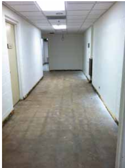
Fig. 3.0.C.31 Flooring mastic with asbestos throughout the basement corridors was abated as of the date of the site survey visit.
