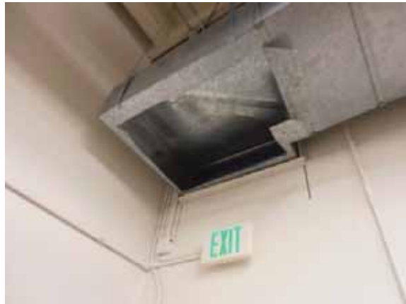
Fig. 2.4.A.31 - Exhaust duct cut open
