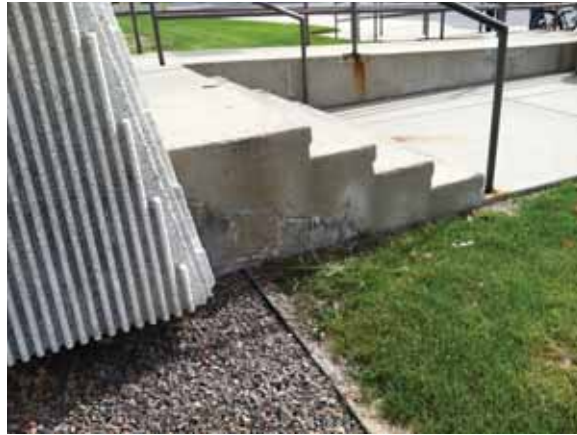
Fig. 2.1.A.66 Spalling and cracked concrete at the exterior stairway to the South Employee Entrance.
