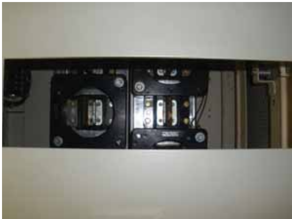
Fig. 2.4.B.6 – Open bus in main electrical gear
