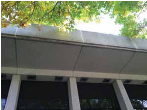
Fig. 2.1.A.11 Soiled precast aggregate panels along the drip edge.
