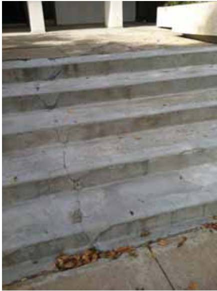
Fig. 2.1.A.63 Spalling and cracking of the concrete stairs at the East Employee Entrance.
