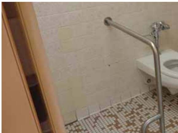
Fig. 3.0.C.15 Areas that were repaired with four-inch square wall tile that does not match the original wall tile.
