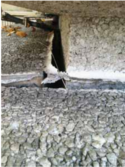
Fig. 2.1.A.57 Close up of the aggregate beams pulling away from the north side of the platform at Entrance B.
