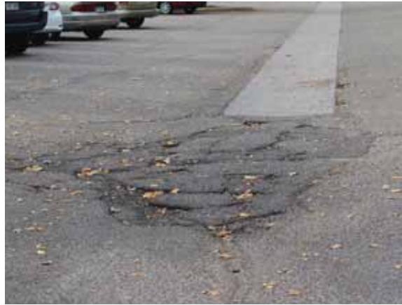
Figure 2.3.A.14 Poor Site Asphalt Condition
