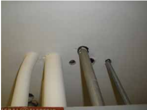
Fig. 2.4.B.5 – Openings in fire rated wall
