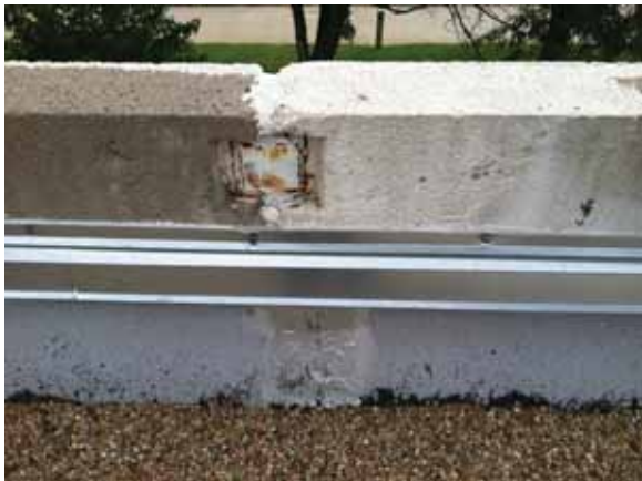
Fig. 2.1.A.29 Deterioration of the concrete parapet around a corroding metal plate.
