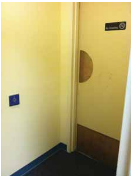
Fig. 3.0.C.33 Typical instance of minor wear and tear noted at a few of the doors throughout the building.
