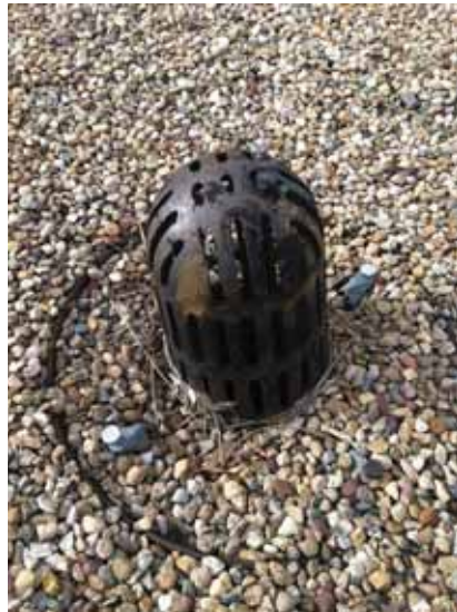
Fig. 2.1.A.48 Typical corroded drain cover, also filled in with ballast, noted at the roof.
