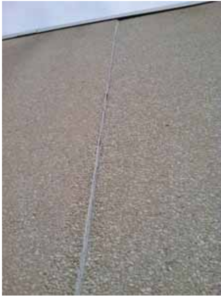
Fig. 2.1.A.4 Precast panel appears to be moving out of flush at the South Penthouse.
