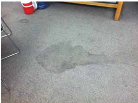
Fig. 3.0.C.24 Typical instance of worn and soiled carpet noted on the Basement Floor of the north wing.
