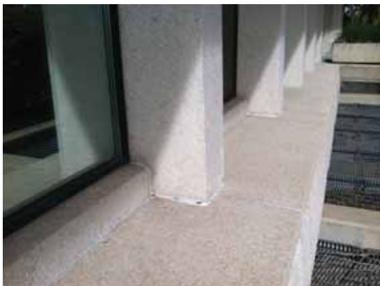
Fig. 2.1.A.24 Deterioration of the sealant around the base of the precast columns.
