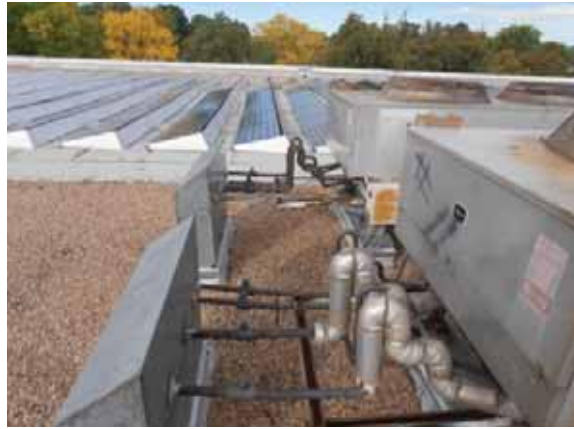
Fig. 2.4.A.18 – Missing insulation on refrigerant piping
