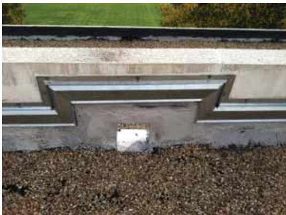
Fig. 2.1.A.46 Deteriorating waterproofing membrane at the roof.
