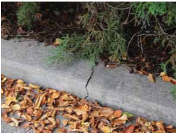
Figure 2.3.A.13 Broken Site Concrete, Recommended for Replacement
