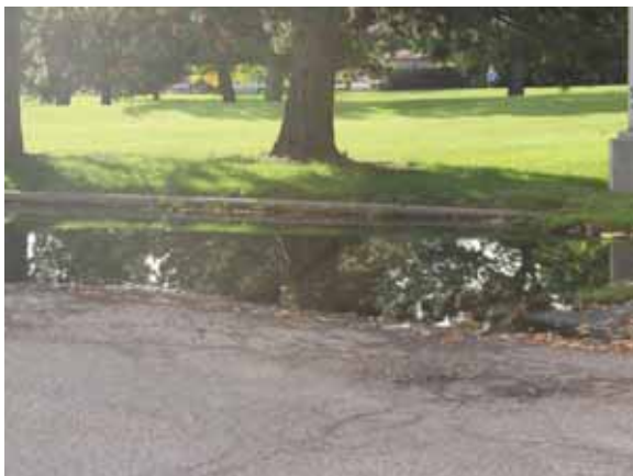
Figure 2.3.B.2 Ponding Water Depth
