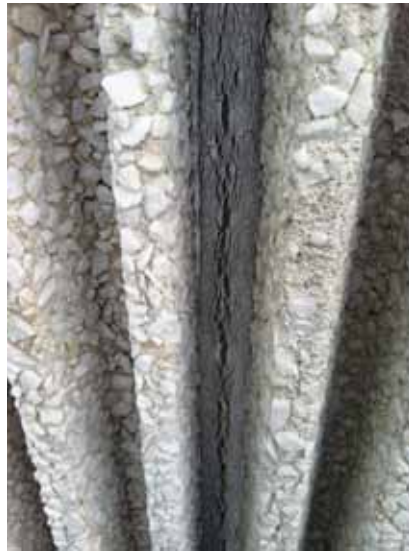
Fig. 2.1.A.20 Deterioration of the sealant between the precast panels.
