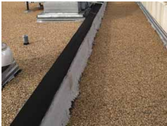
Fig. 2.1.A.45 Deteriorating waterproofing membrane at the roof.
