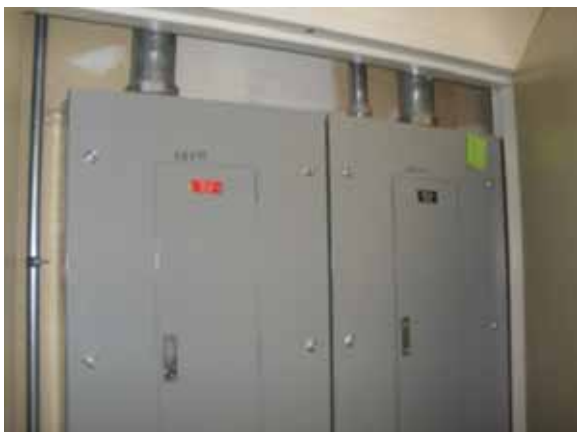
Fig. 2.4.A.4 – Panels in the electrical closets
