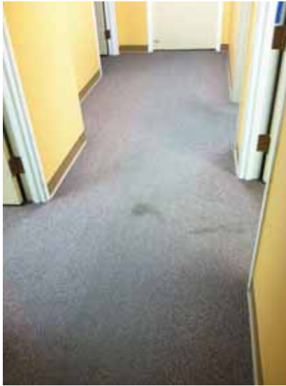
Fig. 3.0.C.22 Typical instance of worn and soiled carpet noted on the First Floor of the north wing.
