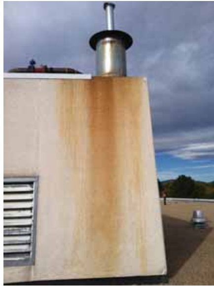
Fig. 2.1.A.13 Precast aggregate panels at the North Penthouse soiled due to corrosion and cracked and spalling at the top and bottom corners.
