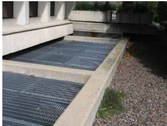
Fig. 2.1.A.78 Moss and/or mold growing on the low concrete window well wall south of the East Employee Entrance.
