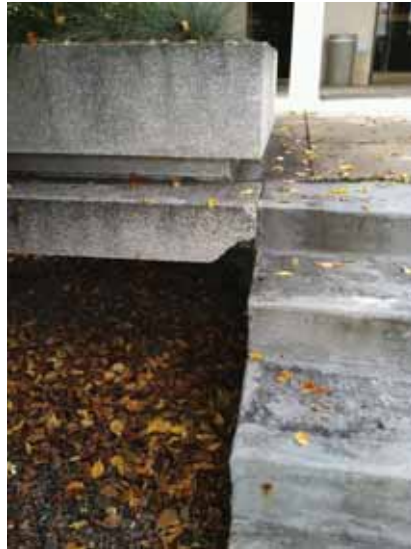
Fig. 2.1.A.60 Spalling aggregate beam at the raised platform at the East Employee Entrance.
