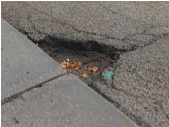
Figure 2.3.A.17 Poor Site Asphalt Condition
