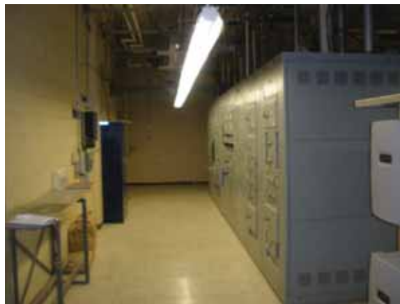
Fig. 2.4.A.1 – Main electrical gear
