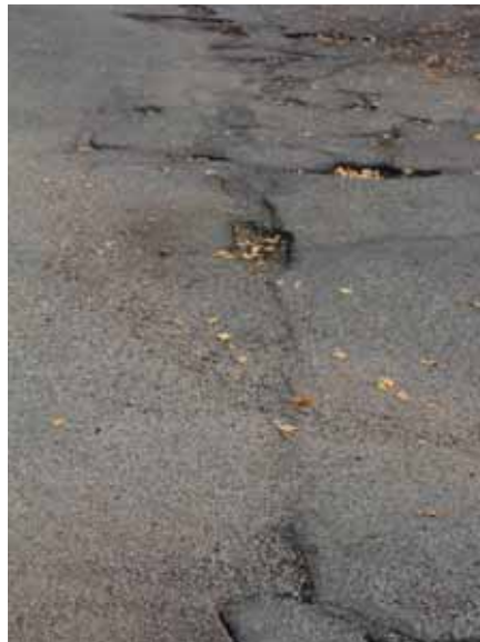
Figure 2.3.A.15 Poor Site Asphalt Condition
