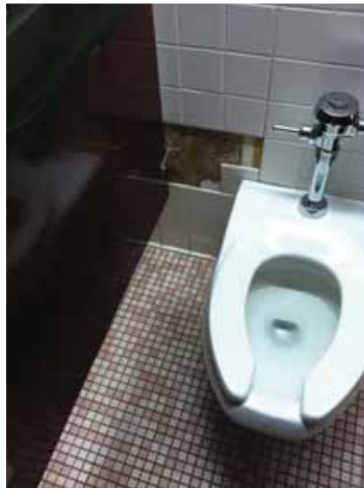
Fig. 3.0.C.16 Missing four-inch square wall tile from the Women's First Floor Restroom on the west side of the south wing.
