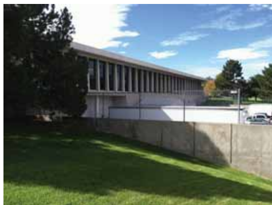
Fig. 2.1.A.72 Typical soiling of the concrete retaining wall on the north side of the building.
