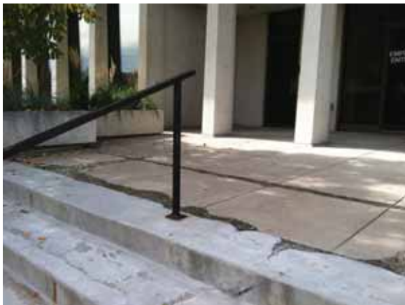
Fig. 2.1.A.64 Spalling and cracking of the concrete pavers at the East Employee Entrance.
