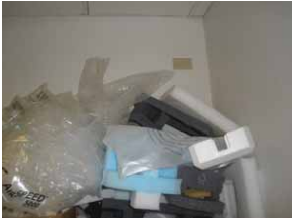
Fig. 2.4.A.27 – Material stored is a fire hazard
