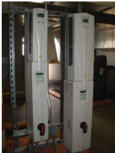
Fig. 2.4.A.17 – VFDs for motors
