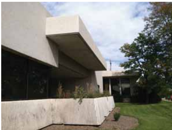
Fig. 2.1.A.6 Soiled precast aggregate panels noted around the building.
