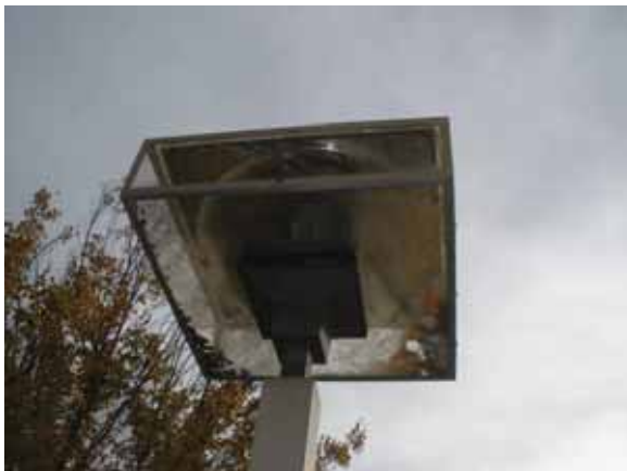
Fig 2.4.A.7 – Parking lot luminaires
