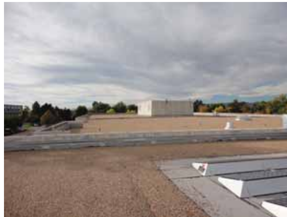
Fig. 2.1.A.26 Generally soiled and worn concrete parapets.
