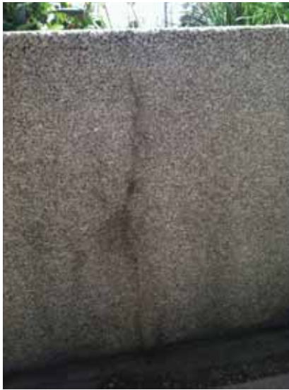
Fig. 2.1.A.17 Large cracking noted in the precast aggregate wall at the outside edge of the exterior porch.
