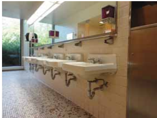
Fig. 2.1.C.4 Typical instance of an accessible lavatory without insulation wrapped around the pipes.
