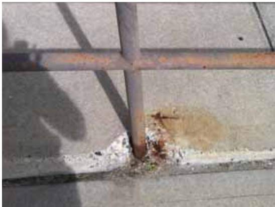
Fig. 2.1.A.70 Spalling concrete causing the corroding guardrail posts to become loose along the ramp to the South Employee Entrance.
