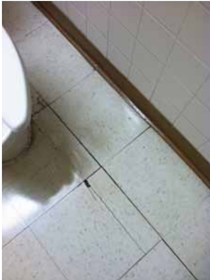
Fig. 3.0.C.29 Damaged linoleum flooring noted in the Women's First Floor Restroom at the northeast corner of the south wing.
