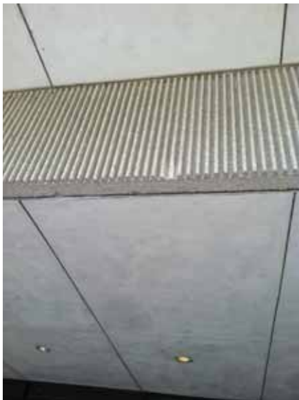
Fig. 2.1.A.55 Areas of minor spalling noted at the precast panels covering the front edges of the entrance canopies.
