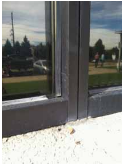
Fig. 2.1.A.34 General deterioration of the weatherstripping surrounding the windows.
