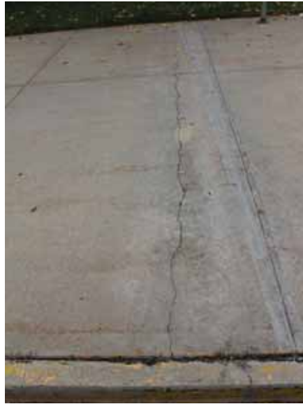
Figure 2.3.A.8 Site Concrete Crack, Recommended for Replacement
