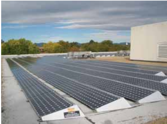
Fig. 2.4.A.2 – PV on the roof
