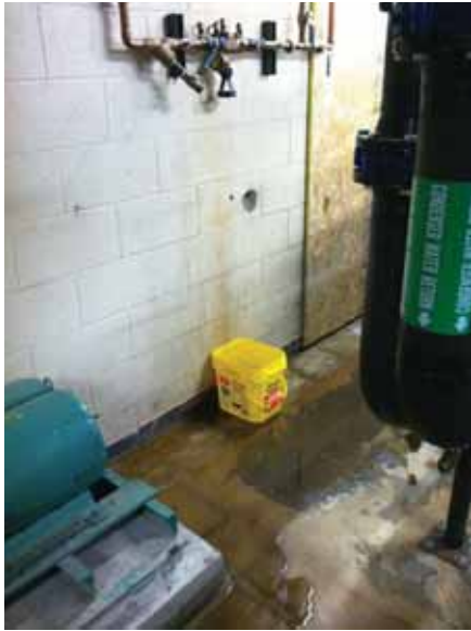
Fig. 3.0.C.32 Water pooling on the concrete floor in the equipment room on the east side of the Basement Floor.
