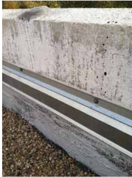
Fig. 2.1.A.30 Areas where the protective coating sealing the concrete parapet is wearing off.
