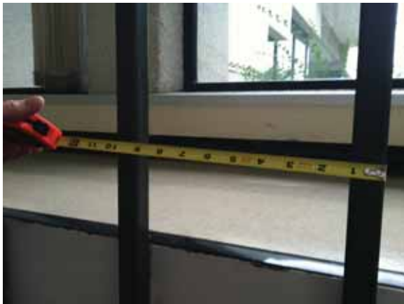
Fig. 2.1.B.4 The spacing between the guardrails along the walkway in the east stairway exceeds the code-maximum of four inches.
