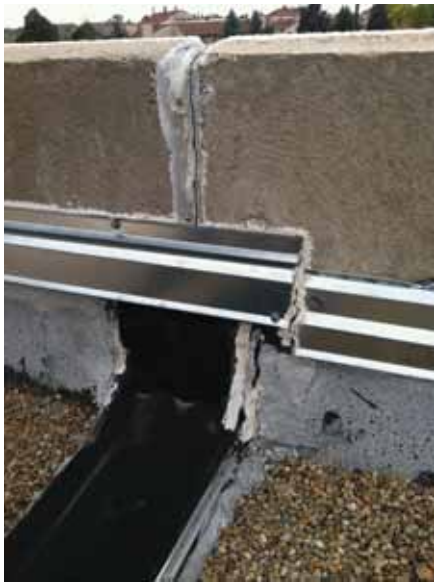
Fig. 2.1.A.50 Flashing incorrectly installed across a control joint.
