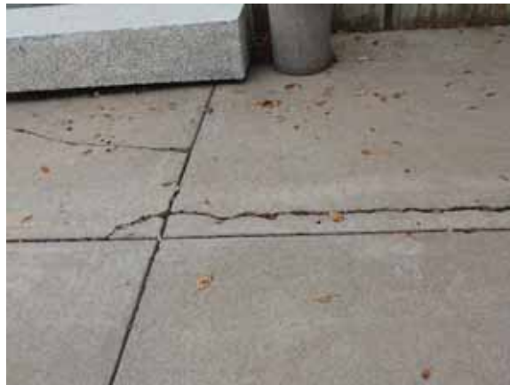
Figure 2.3.A.9 Site Concrete Crack, Recommended for Replacement
