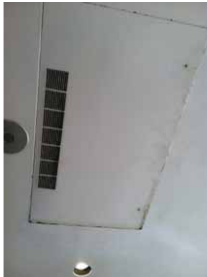
Fig. 3.0.C.7 Water damage at the gypsum board ceiling around the ceiling panel in the vestibule of the East Employee Entrance.
