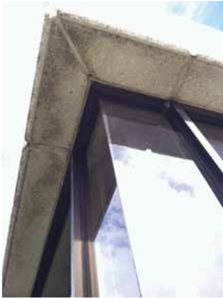
Fig. 2.1.A.10 Soiled precast aggregate panels along the bottom edge located above the windows.
