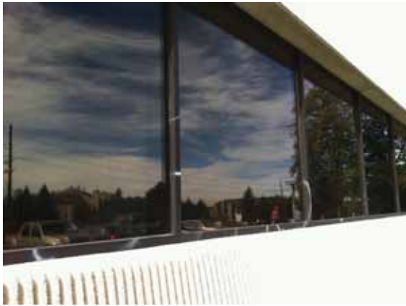
Fig. 2.1.A.37 Window frames that appear to have spots that were spray painted with white paint.
