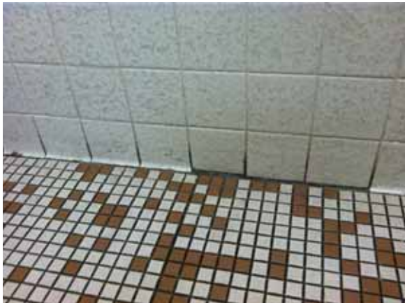
Fig. 3.0.C.14 Typical instance of soiled four-inch square wall tile observed in the restrooms.
