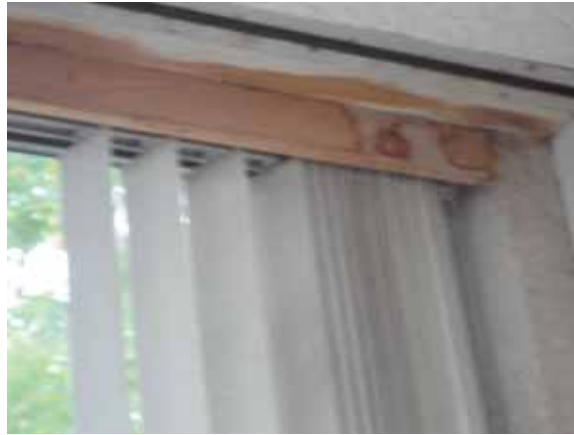
Fig. 2.1.A.39 Water damage noted along the top of a window from the interior side of the building.
