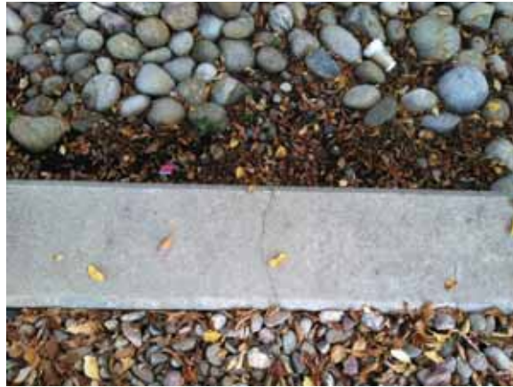
Fig. 2.1.A.77 Cracked concrete at a low landscaping wall.
