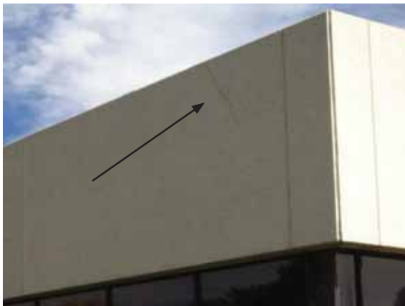
Fig. 2.1.A.5 Cracked areas of the precast aggregate panels noted around the building.
