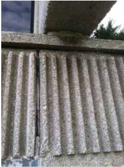
Fig. 2.1.A.22 Deterioration of the sealant between the precast panels.
