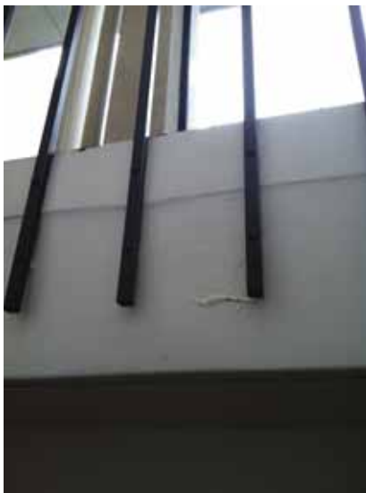
Fig. 3.0.C.21 Water damage noted at the gypsum board in the west stairway.
