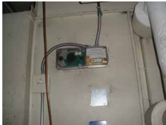
Fig. 2.4.A.13 – Duct smoke detector
