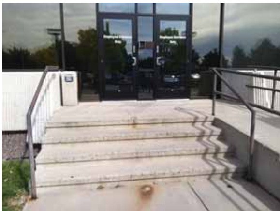
Fig. 2.1.A.65 Minor spalling of the concrete stairs and holes left in the concrete surface where guardrail posts were previously removed at the South Employee Entrance.
