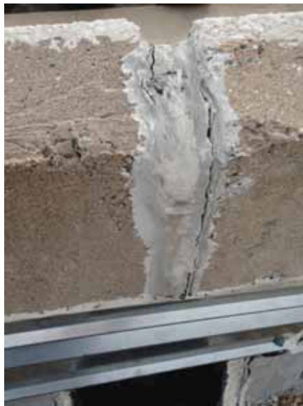
Fig. 2.1.A.31 Deteriorating sealant typical around the concrete parapets.
