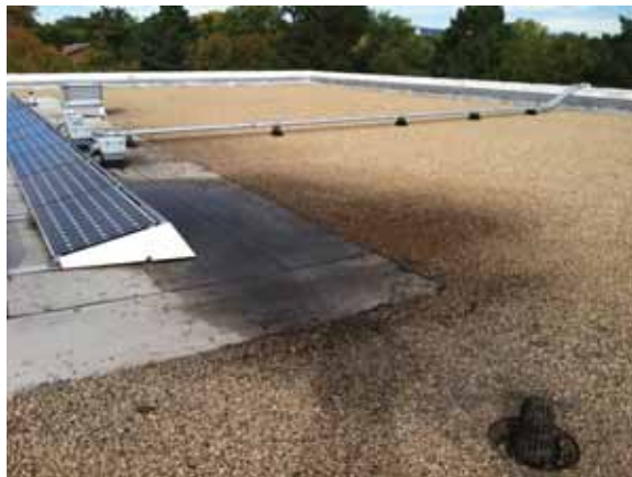
Fig. 2.1.A.42 Areas of pooling water noted around the roof.
