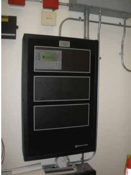
Fig. 2.4.A.11 – Fire alarm control panel
