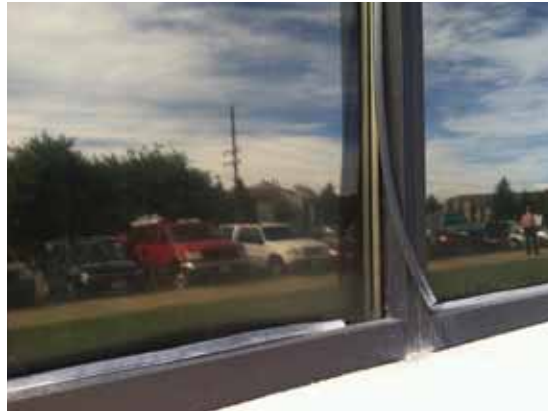
Fig. 2.1.A.33 General deterioration of the weatherstripping surrounding the windows.
