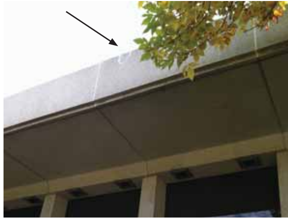
Fig. 2.1.A.1 Areas of spalling noted at the precast aggregate panels.
