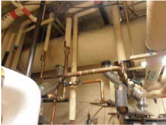
Fig. 2.4.A.33 – Missing insulation on hot water piping
