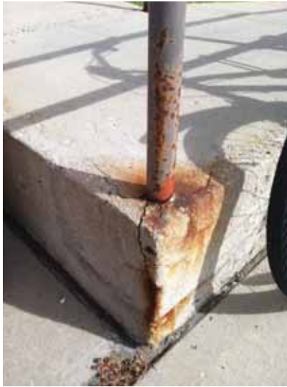
Fig. 2.1.A.69 Cracked concrete causing the corroding guardrail posts to become loose along the ramp to the South Employee Entrance.
