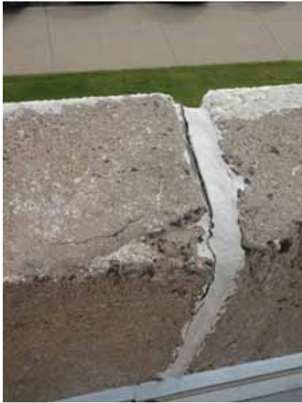
Fig. 2.1.A.27 Spalling and cracking areas of the parapet noted during the site visit.
