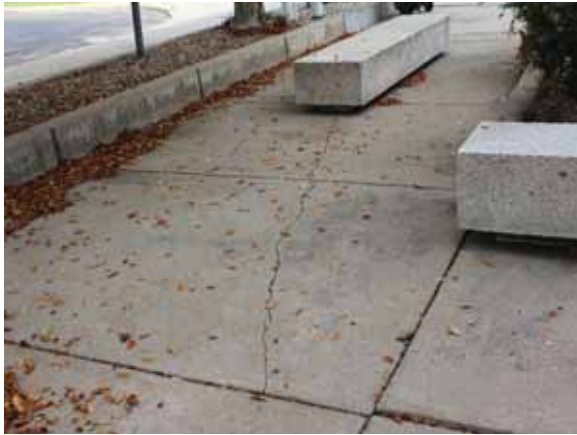
Figure 2.3.A.11 Site Concrete Crack, Recommended for Replacement
