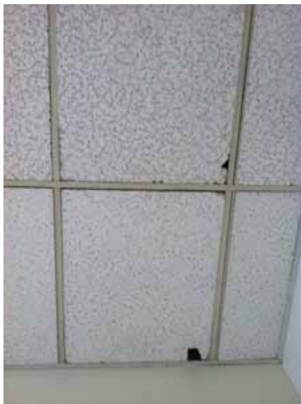
Fig. 3.0.C.2 Typical instance of deterioration of the acoustic ceiling tiles.
