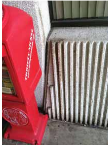
Fig. 2.1.A.7 Soiled precast aggregate panels noted around the building.
