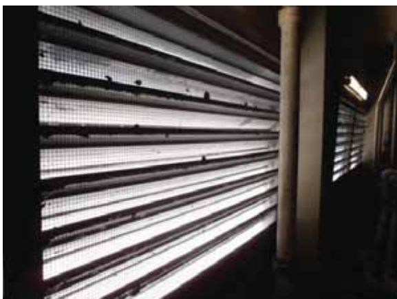
Fig. 2.4.A.23 – Outside air dampers for cooling tower
