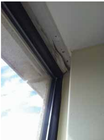
Fig. 2.1.A.38 Water damage noted along the top of a window from the interior side of the building.
