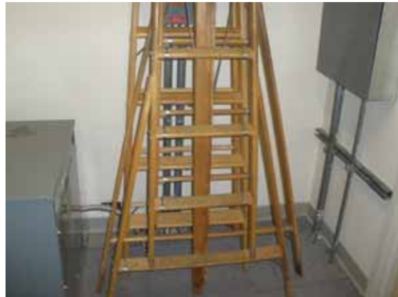
Fig. 2.4.B.3 – Ladders within panelboard and transformer clearance
