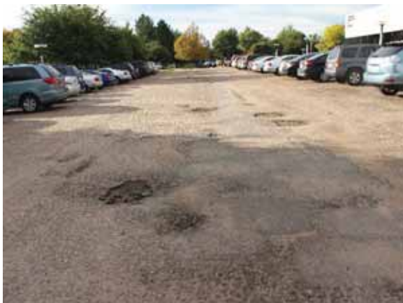
Figure 2.3.A.19 Poor Site Asphalt Condition
