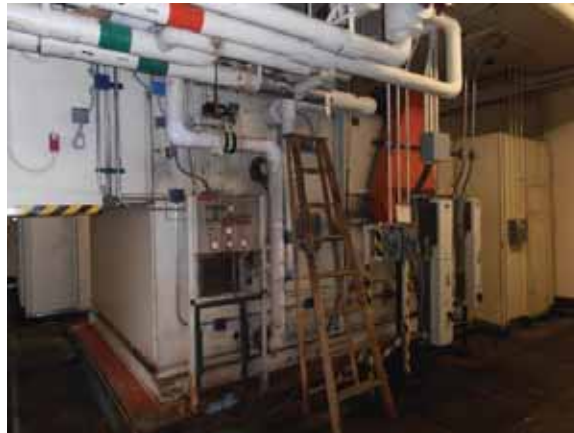
Fig. 2.4.A.19 – North building Trane units
