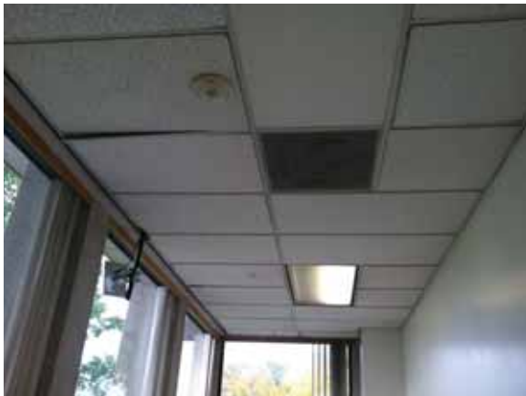
Fig. 3.0.C.1 General deterioration and poor condition of the acoustic ceilings throughout.
