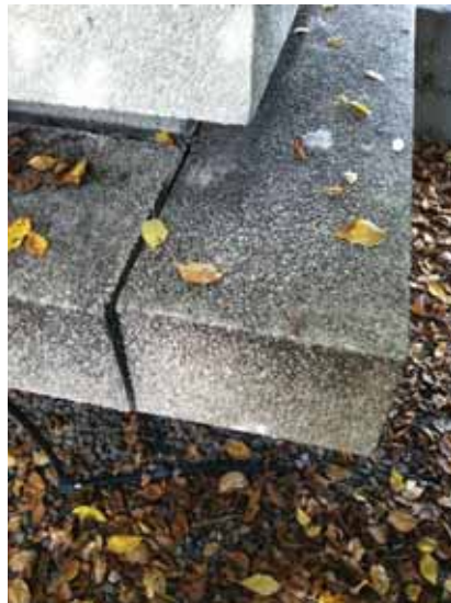
Fig. 2.1.A.61 Aggregate beam that appears to be pulling away from the platform at the East Employee Entrance.
