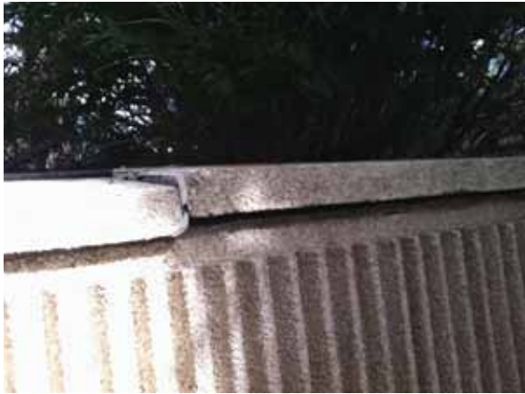
Fig. 2.1.A.75 Capping piece of the north retaining wall on the east side of the building moving out of place and with deteriorating sealant.
