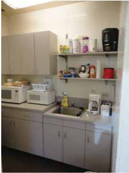
Fig. 2.1.C.6 Typical non-accessible sink found in the Break Rooms throughout.
