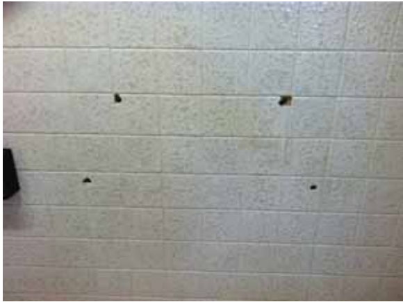
Fig. 3.0.C.13 Typical instance of discolored, soiled, and damaged four-inch square wall tile observed in the restrooms throughout the north wing.
