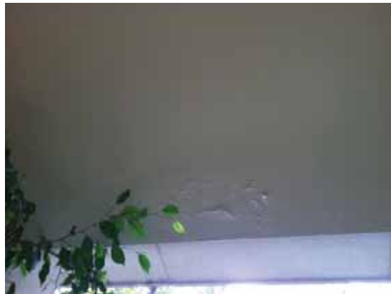
Fig. 3.0.C.8 Water damage at the gypsum board ceiling in the Women's First Floor Restroom on the west side of the north wing.
