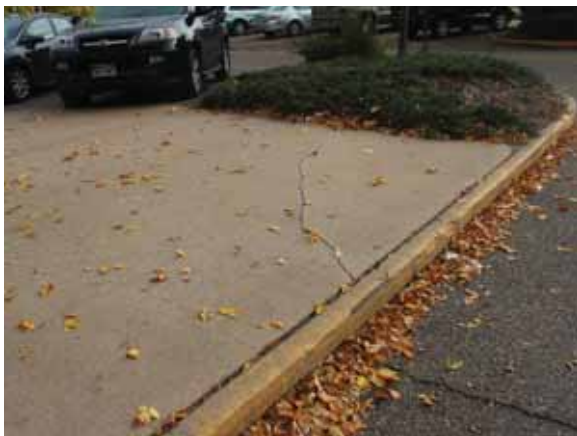
Figure 2.3.A.7 Site Concrete Crack, Recommended for Replacement
