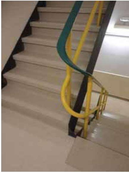
Fig. 2.1.B.3 The spacing between the guardrails in the west stairway exceeds the code-maximum of four inches.
