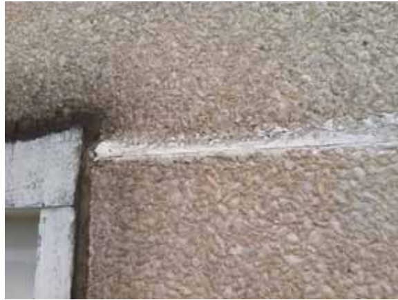
Fig. 2.1.A.25 Typical deterioration of the sealant at the two Penthouses on the roof.
