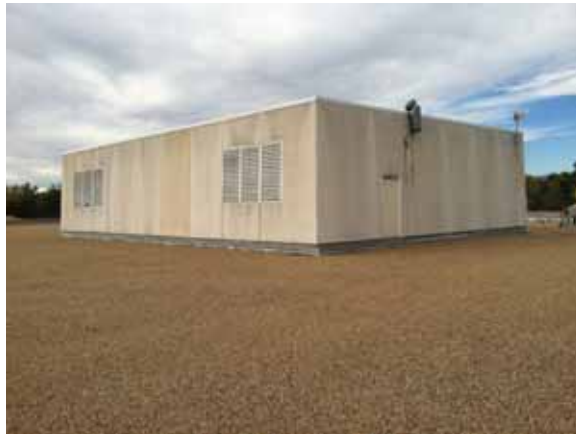
Fig. 2.1.A.14 Generally soiled precast aggregate panels at the South Penthouse.
