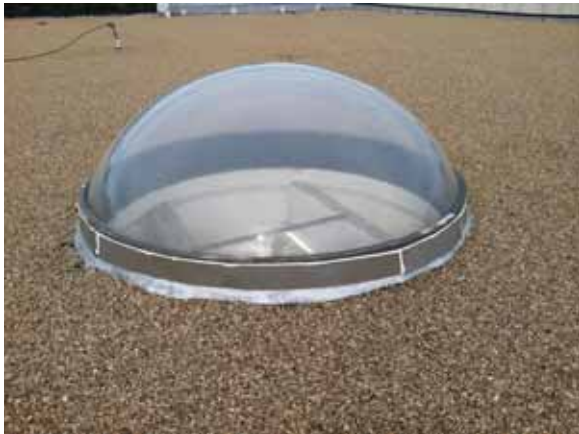
Fig. 2.1.A.51 Deteriorating sealant at the skylight near the middle of the roof.
