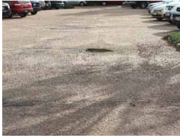
Figure 2.3.A.20 Poor Site Asphalt Condition
