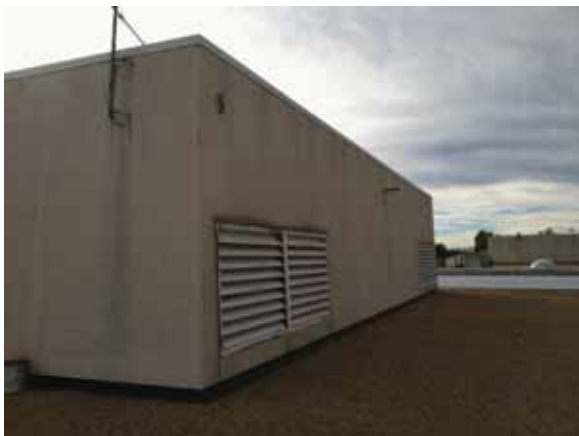
Fig. 2.1.A.12 Generally soiled precast aggregate panels at the North Penthouse.
