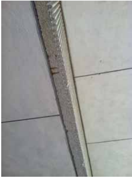
Fig. 2.1.A.54 Brown substance leaking out from behind a precast panel covering the front edge of the canopy at Entrance A.
