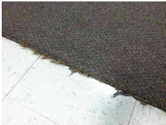
Fig. 3.0.C.26 Instance of worn and deteriorating carpet noted during the site survey visit.
