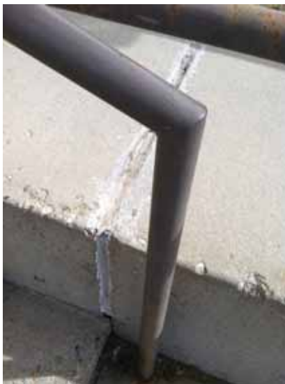
Fig. 2.1.A.71 Deteriorating sealant between the concrete slabs at the ramp to the South Employee Entrance.
