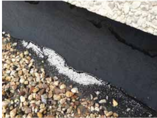
Fig. 2.1.A.47 Deteriorating waterproofing membrane at the roof.
