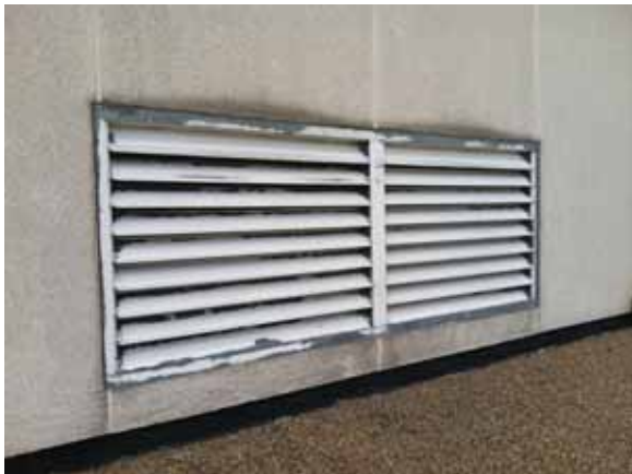
Fig. 2.1.A.52 Paint deteriorating and peeling off the louvers at the North Penthouse.
