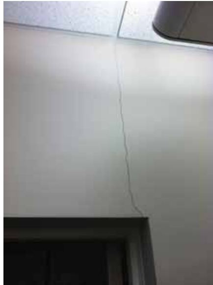
Fig. 3.0.C.10 Cracking in the gypsum board walls noted throughout the north wing.
