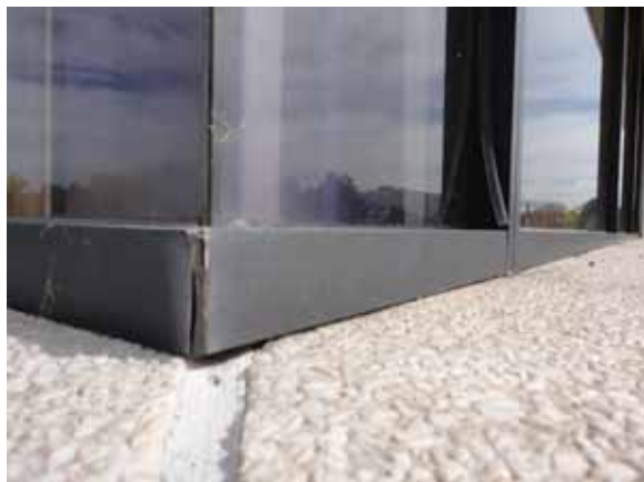
Fig. 2.1.A.32 General deterioration of the sealant and weatherstripping surrounding the windows.
