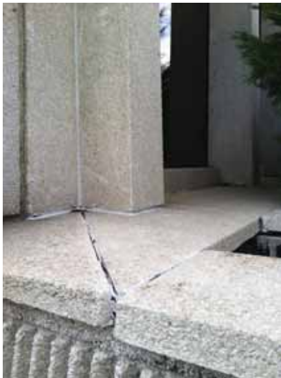
Fig. 2.1.A.23 Deterioration of the sealant along the window ledge.
