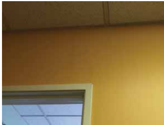
Fig. 3.0.C.11 Cracking in the gypsum board walls noted throughout the north wing.
