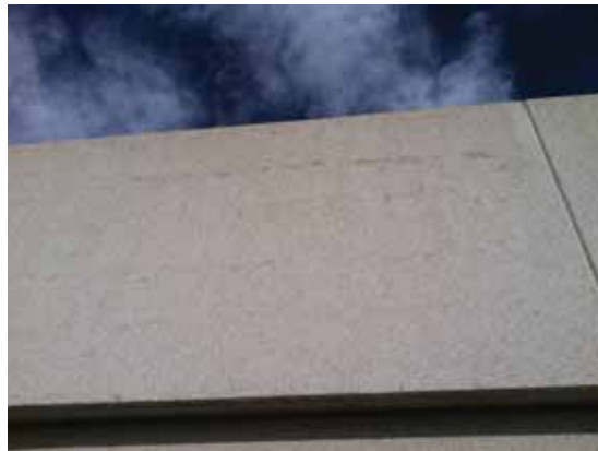
Fig. 2.1.A.8 Soiled precast aggregate panels noted around the building.
