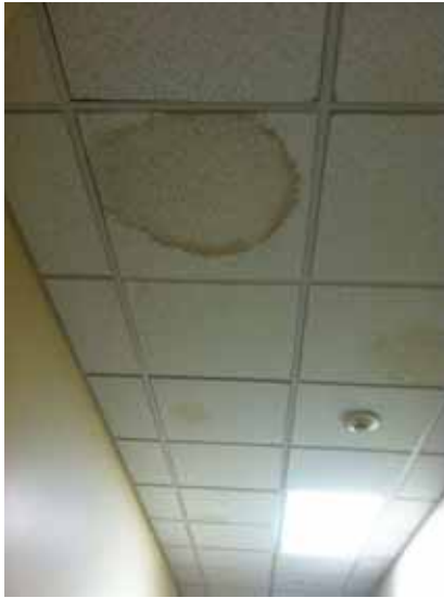
Fig. 3.0.C.4 Typical instance of soiled acoustic ceiling tiles.
