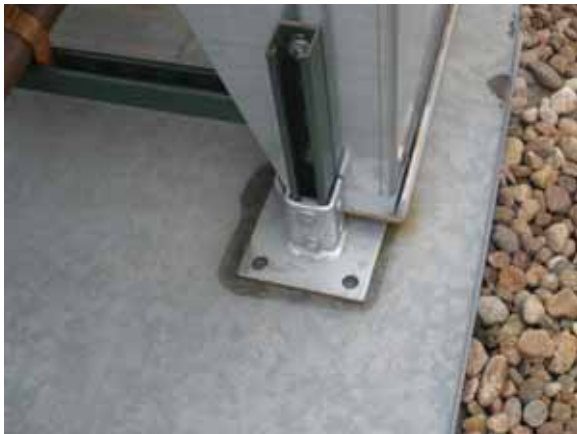
Fig 2.4.B.4 – Unit not bolted to structure
