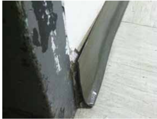
Fig. 3.1.C.20 Damage to vinyl baseboard observed in the main corridors throughout the Basement Floor.
