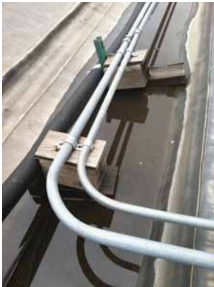
Fig. 2.1.A.36 Issues with ponding on the roof.
