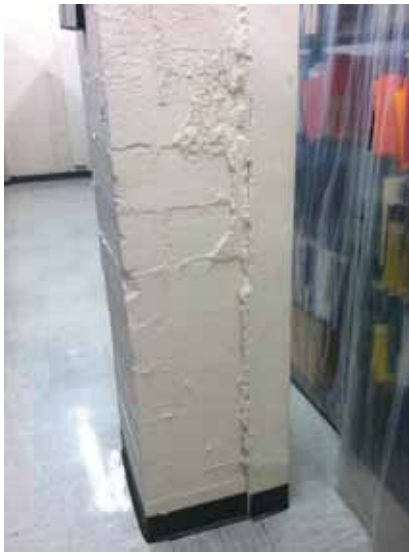
Fig. 3.1.C.24 Typical spalling noted at the columns in Room B-13 Library Stacks.
