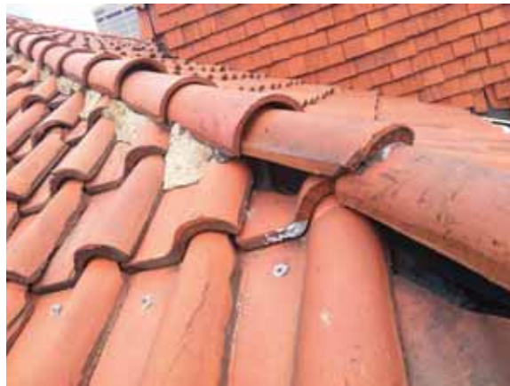
Fig. 2.1.A.44 Missing grout at openings between terra cotta tiles.
