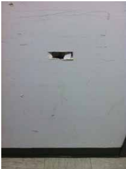
Fig. 3.1.C.19 Damage to gypsum board walls observed in the main corridors throughout the Basement Floor.
