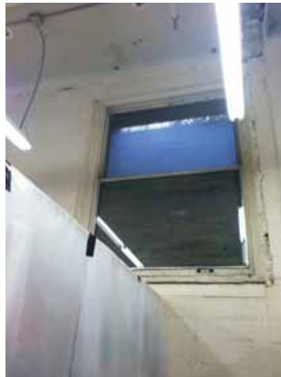
Fig. 3.1.C.21 Spalling and cracking around the windows along the exterior wall in Room B-13 Library Stacks.
