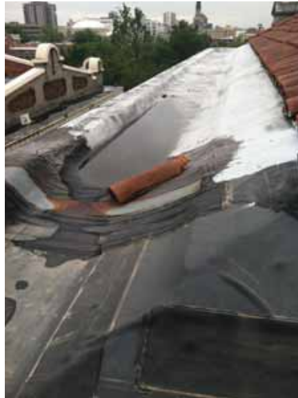
Fig. 2.1.A.39 Sharp debris collecting on the roof membrane.
