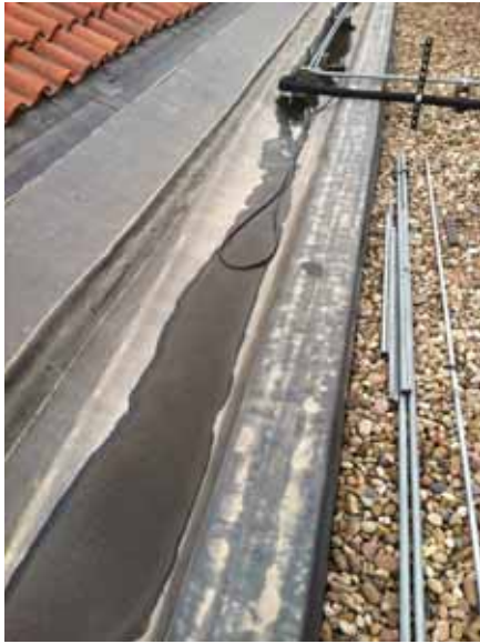
Fig. 2.1.A.35 Issues with ponding on the roof.
