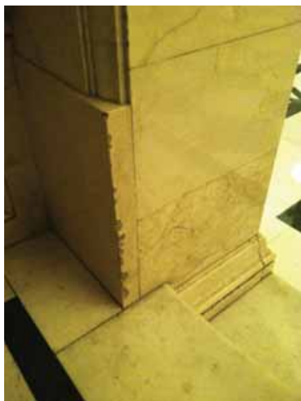
Fig. 3.1.C.7 Damaged stone at the base of the northwest stairway on the First Floor.
