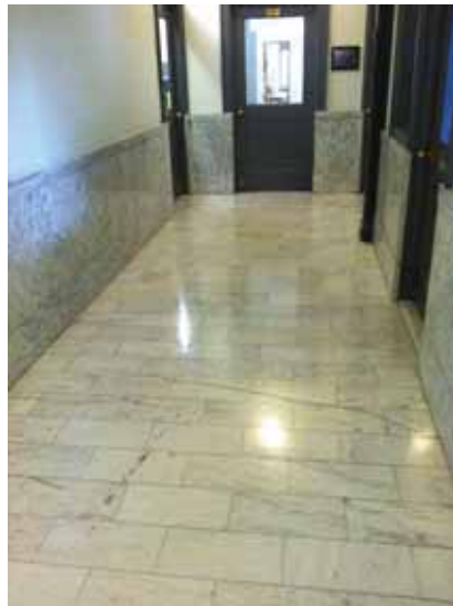
Fig. 3.1.C.29 Typical cracked and soiled stone flooring observed in the main corridors.
