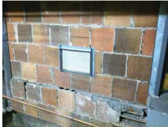
Fig. 2.1.A.21 Deteriorating masonry wall observed from the inside of the attic space.
