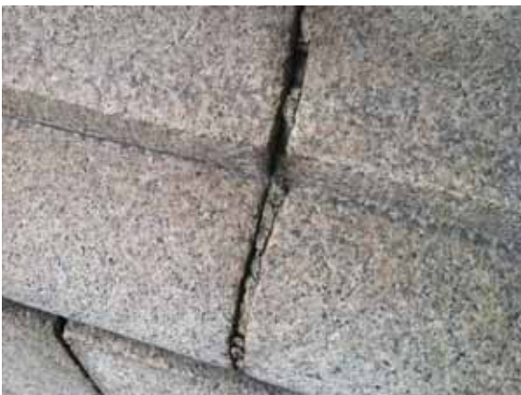
Fig. 2.1.A.15 Deteriorated grout between granite blocks.
