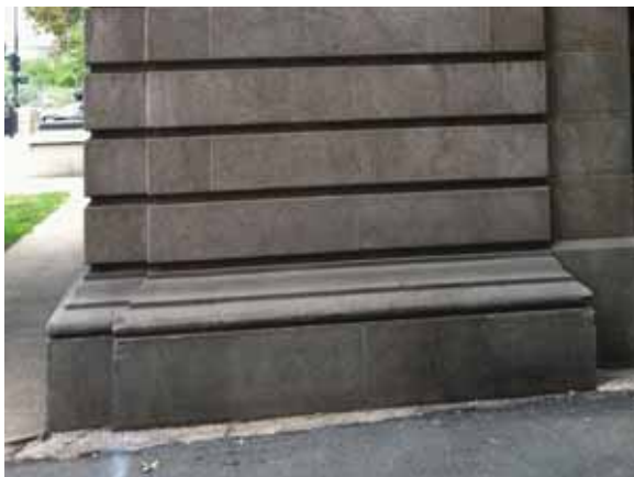
Fig. 2.1.A.5 Spalling of the granite along the base of the building.
