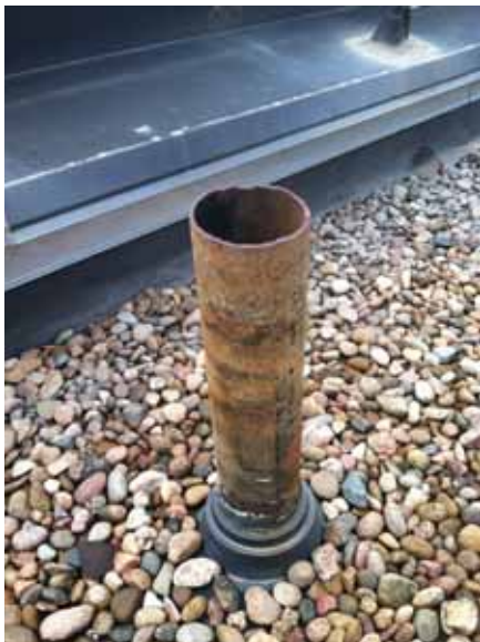
Fig. 2.1.A.47 Exhaust pipe with signs of corrosion.
