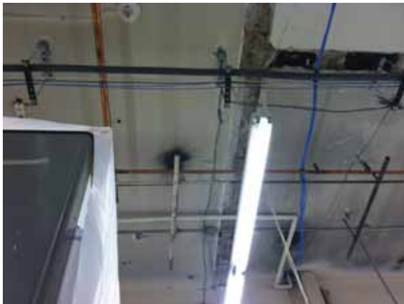
Fig. 3.1.C.4 Damaged ceiling in Room B-13 Library Stacks.
