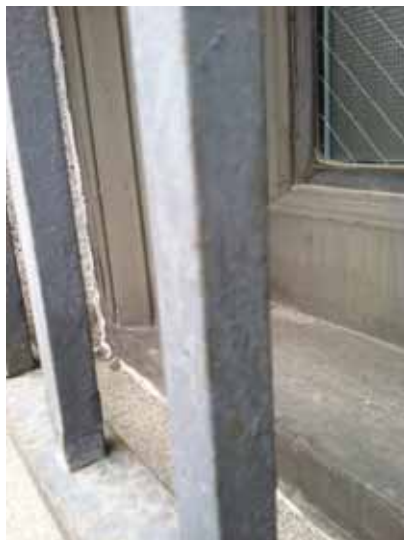
Fig. 2.1.A.23 Corroding metal window frame.
