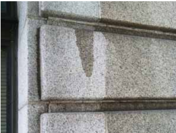
Fig. 2.1.A.14 Deteriorated grout between granite blocks.
