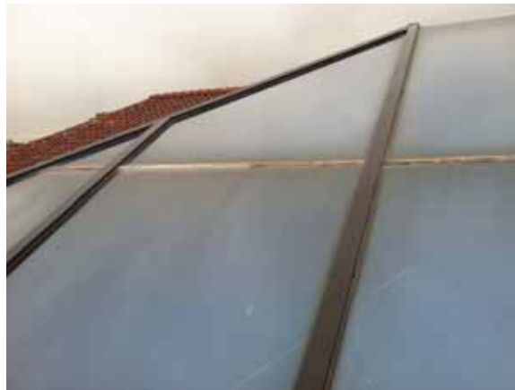
Fig. 2.1.A.49 Deteriorated sealant at the skylight.
