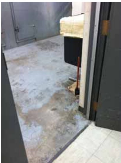
Fig. 3.1.C.39 Worn and cracked paint on the concrete flooring in the Fire Pump Room in the basement.
