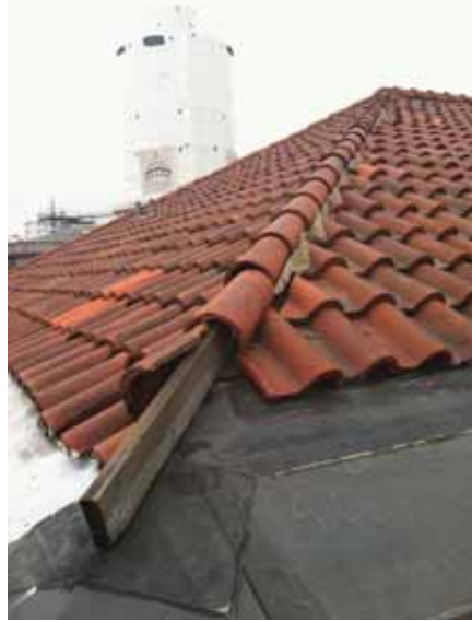
Fig. 2.1.A.43 Missing terra cotta tiles.
