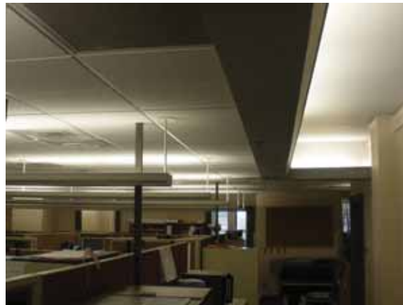
Fig 2.4.A.3 – Indirect office lighting
