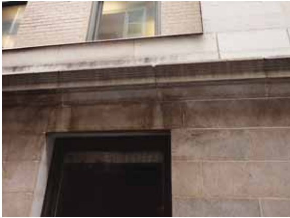
Fig. 2.1.A.8 Soiled granite blocks typical under a building ledge.
