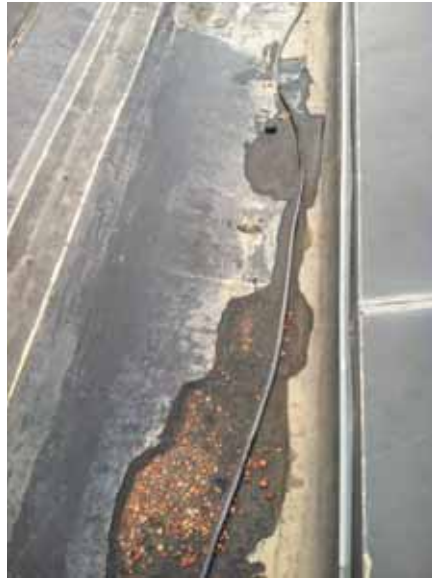
Fig. 2.1.A.38 Sharp debris collecting on the roof membrane.
