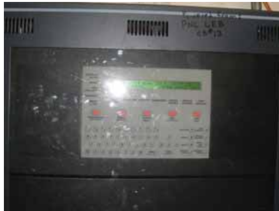
Fig 2.4.A.7 – Fire alarm control panel
