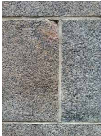
Fig. 2.1.A.1 Spalling of the granite.
