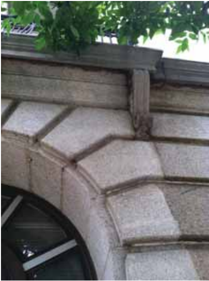
Fig. 2.1.A.13 Deteriorated grout between granite blocks.
