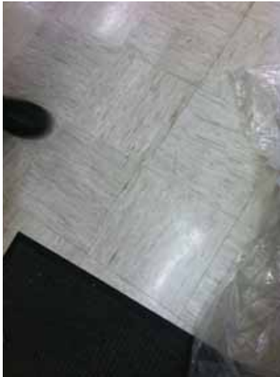
Fig. 3.1.C.37 Cracked one-foot square linoleum tile flooring in Room B-13 Library Stacks in the basement.
