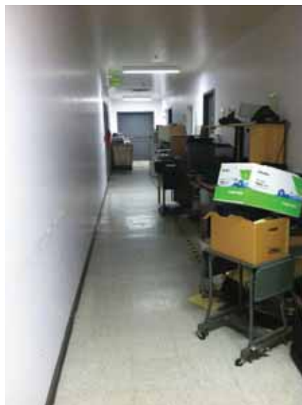
Fig. 2.1.B.5 Furniture intruding into the exit corridor, beyond the marked storage areas, leading to the northeast stair at the Basement Floor.
