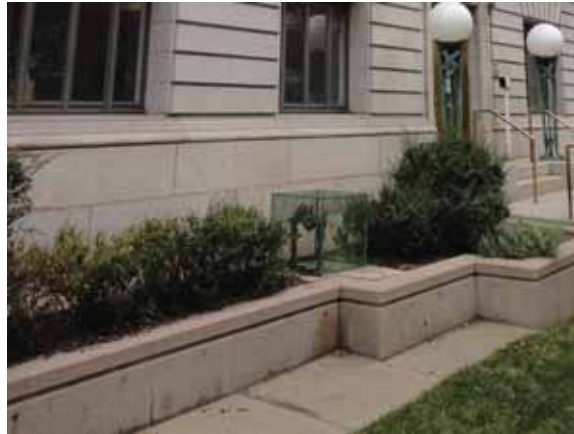
Fig. 2.1.A.11 Cracked and soiled granite along the low landscaping retaining wall.
