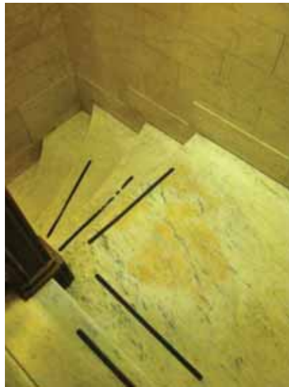
Fig. 3.1.C.28 Soiled areas of polished stone cladding the northwest stairway connecting the First and Second Floor.
