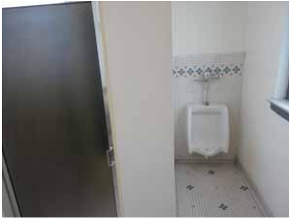
Fig. 2.1.C.4 Fifth Floor urinal alcove is too narrow per accessibility standards.
