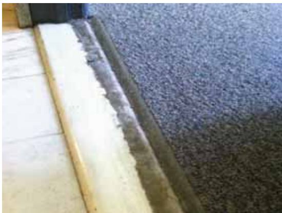
Fig. 3.1.C.33 General wear-and-tear and soiling noted at thresholds.
