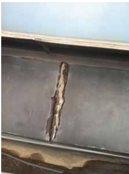
Fig. 2.1.A.52 Deteriorated sealant at membrane surrounding base of skylight.
