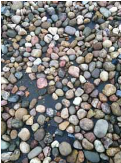
Fig. 2.1.A.32 Typical area of thin ballast and accumulation of dirt.
