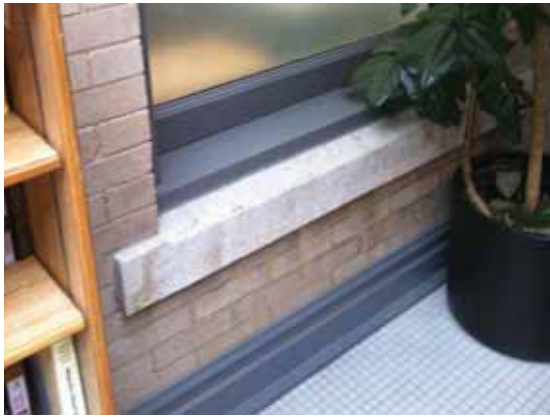
Fig. 3.1.C.18 Deteriorating grout and minor soiling of the brick and stone window sills within the Fourth Floor atrium space.
