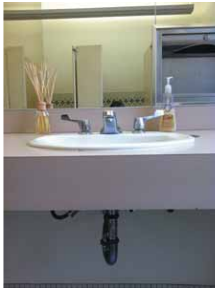
Fig. 2.1.C.1 Insulation missing from around the lavatory pipes in the Women's Restroom on the First Floor.
