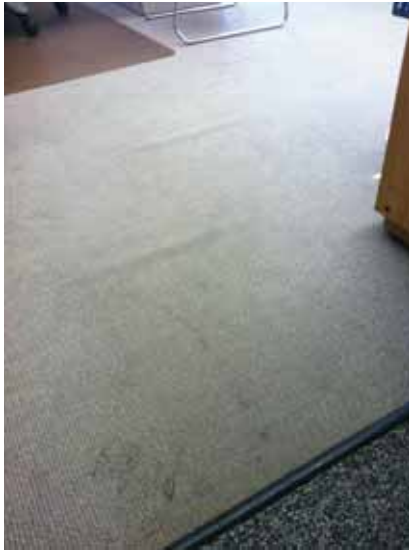
Fig. 3.1.C.31 Typical soiled and worn carpet pulling loose and creating a potential tripping hazard.
