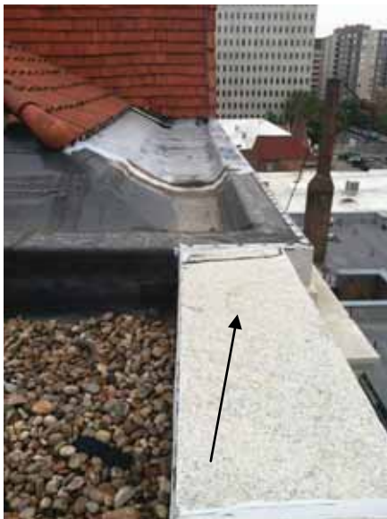
Fig. 2.1.A.20 Evidence of water pooling on the granite stone blocks along the top edge of the parapet.
