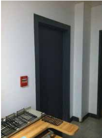
Fig. 2.1.B.1 Unlabeled exit stairway door to the southwest stair from the Basement Floor.
