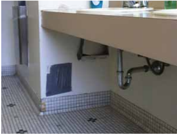
Fig. 3.1.C.11 Holes in the plaster wall under the counter in the Women's Restroom on the First Floor that have not been repaired correctly.
