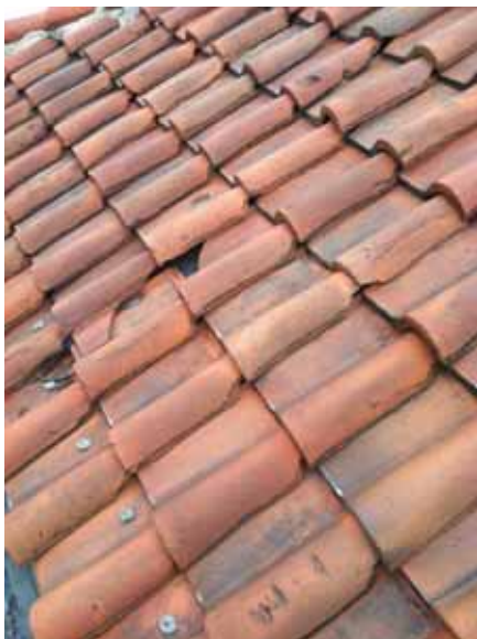
Fig. 2.1.A.42 Cracked terra cotta tiles.
