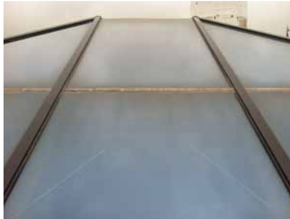
Fig. 2.1.A.48 Deteriorated sealant at the skylight.
