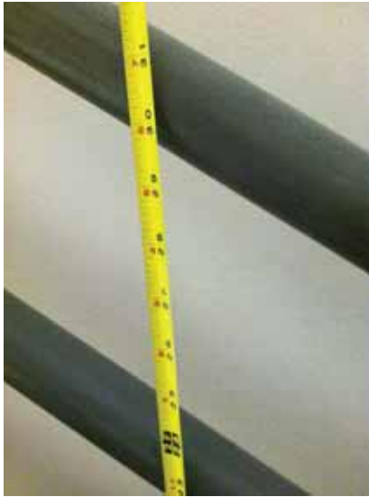
Fig. 2.1.B.8 The distance between the guardrail openings exceeds 4 inches in diameter.
