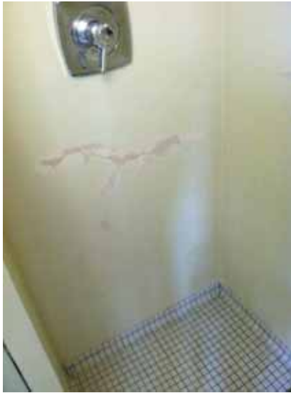
Fig. 3.1.C.17 Damaged shower walls in the Women's Restroom on the Fifth Floor.
