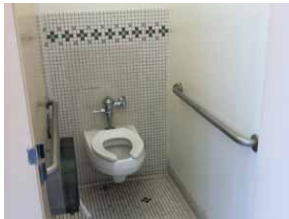
Fig. 3.1.C.15 Areas of discolored one-inch square tile wainscoting noted in the restrooms.
