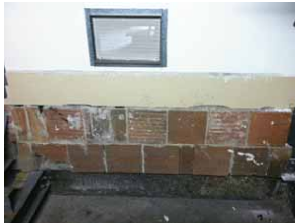
Fig. 2.1.A.22 Deteriorating masonry wall observed from the inside of the attic space.
