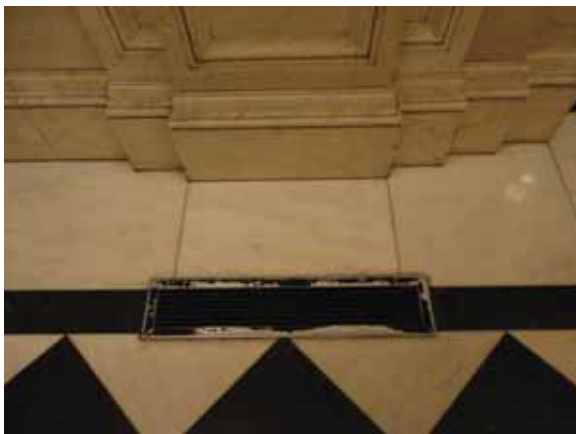
Fig. 3.1.C.27 Floor vent cover missing paint and showing general signs of wear-and-tear in the vaulted atrium space on the First Floor.
