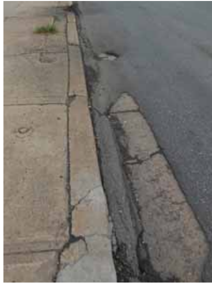
Figure 2.3.A.9 – Broken Curb, Recommended for Replacement
