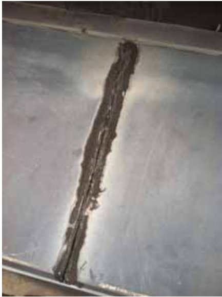
Fig. 2.1.A.51 Deteriorated sealant at membrane surrounding base of skylight.
