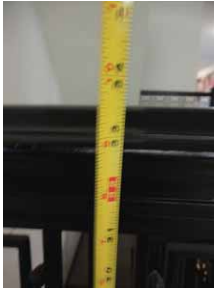
Fig. 2.1.B.11 The height to the top of the guardrail along the edge of the unenclosed northwest stairway.
