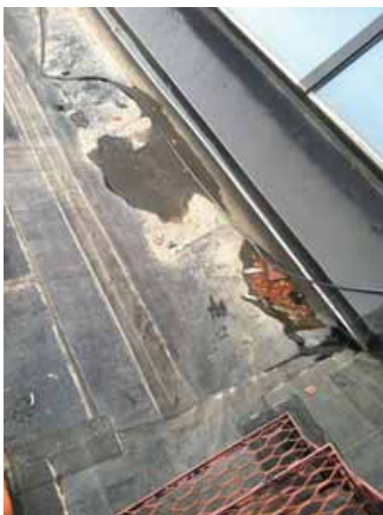
Fig. 2.1.A.37 Sharp debris collecting on the roof membrane.
