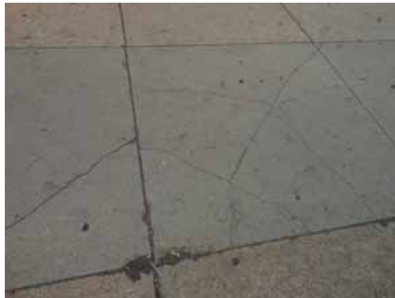
Figure 2.3.A.10 – Broken Site Concrete, Recommended for Replacement
