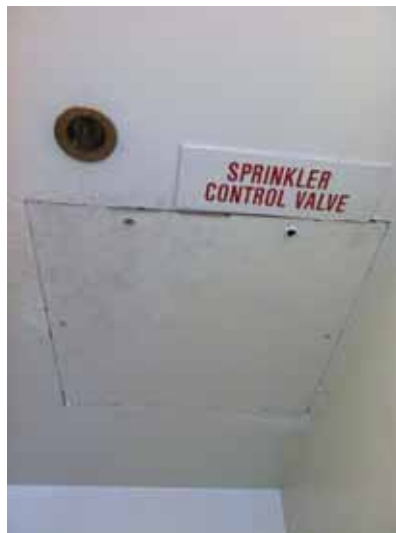
Fig. 3.1.C.1 Soiled access panel observed in the Women's Restroom on the Fourth Floor.
