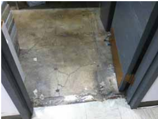
Fig. 3.1.C.38 Cracked and spalling concrete flooring in the CDE Mailroom in the basement.
