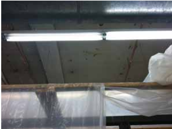
Fig. 3.1.C.3 Damaged ceiling and plastic sheeting covering the storage shelves in Room B-13 Library Stacks.
