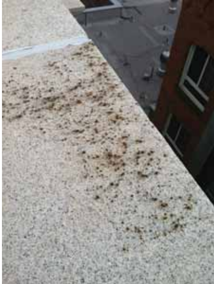
Fig. 2.1.A.19 Pitting of the granite stone blocks along the top edge of the parapet.
