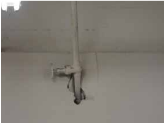
Fig. 3.1.C.23 Unsealed opening around a pipe passing through the wall in Room B-13 Library Stacks.
