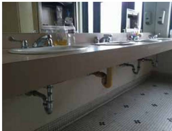
Fig. 2.1.C.2 Insulation is wrapped around the pipes of the non-accessible lavatory with knob-style faucet controls in the Women's Restroom on the Third Floor.
