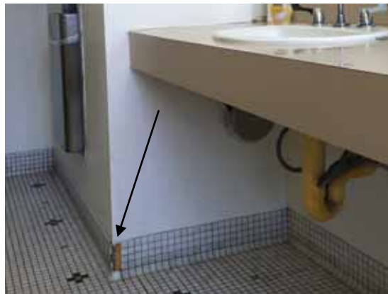
Fig. 3.1.C.35 Typical area of damaged one-inch square tile in the Women's Restroom on the First, Second, and Fourth Floors.
