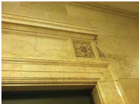
Fig. 3.1.C.6 Cracked stone observed in the central atrium space on the First Floor.
