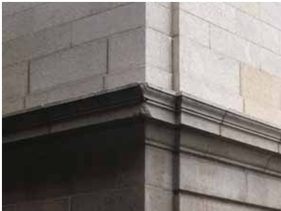
Fig. 2.1.A.4 Spalling of the granite at a corner ledge.
