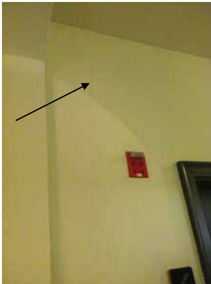
Fig. 3.1.C.12 Large crack in the plaster wall noted in the main corridor area on the Second Floor.
