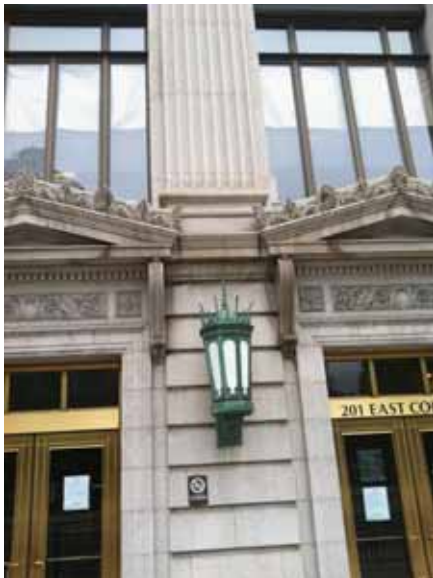
Fig. 2.1.A.9 Soiled stone architrave surrounds above the East Colfax Entrance doors.
