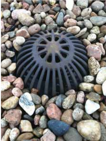
Fig. 2.1.A.46 Drain cover with signs of corrosion.
