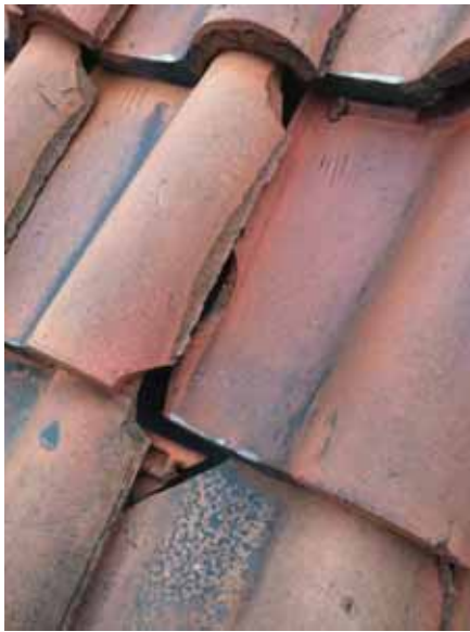
Fig. 2.1.A.41 Cracked terra cotta tiles.
