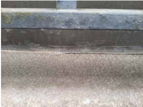
Fig. 2.1.A.27 Deteriorating sealant surrounding window frames.
