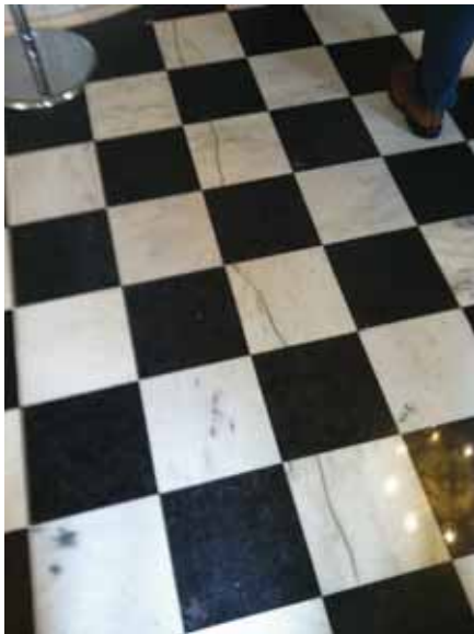
Fig. 3.1.C.26 Large crack across the marble flooring in the East Colfax Entrance Vestibule on the First Floor.
