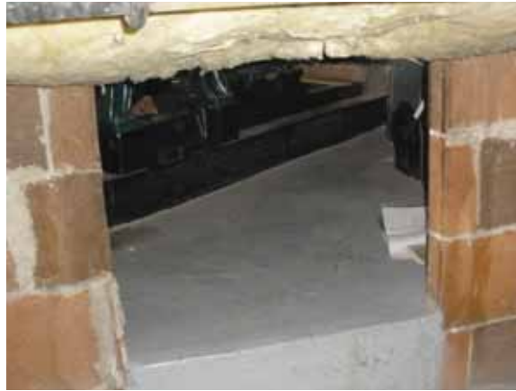
Fig 2.4.B.1 - 3' x 3' opening for elevator motor
