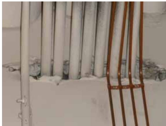
Fig 2.4.B.2 – Penetrations not sealed
