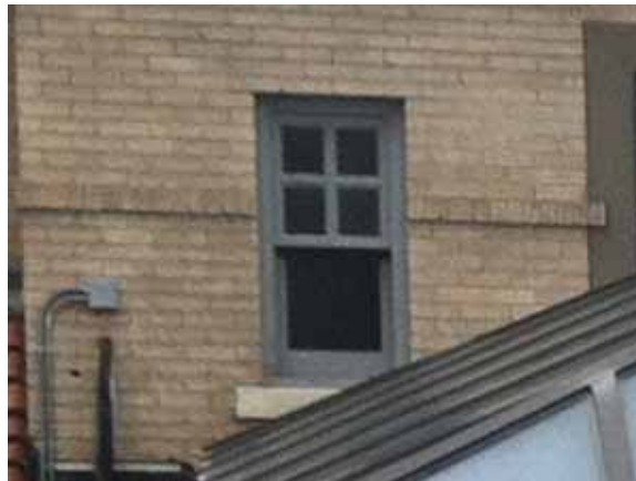
Fig. 2.1.A.25 Corroding metal window frame at the Penthouse.
