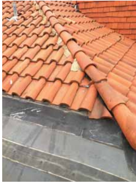
Fig. 2.1.A.33 Area where the membrane is beginning to tear.
