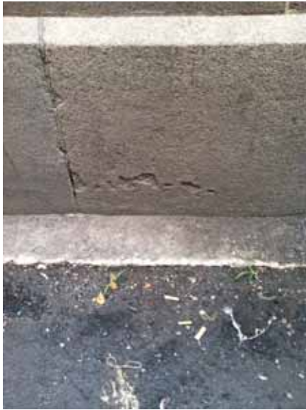
Fig. 2.1.A.3 Spalling of the granite at the base of the building.
