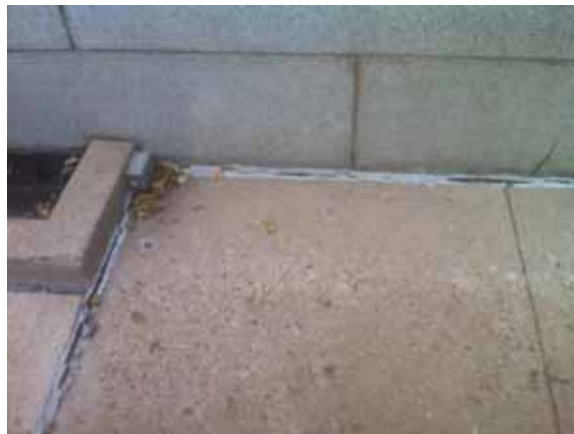
Fig. 2.1.A.17 Deteriorated sealant along the base of the building.
