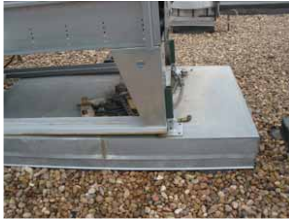
Fig 2.4.B.5 - Condenser unit on the roof not bolted
