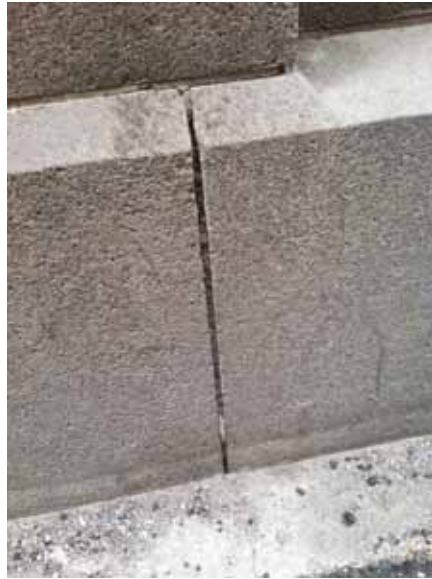
Fig. 2.1.A.16 Deteriorated grout between granite blocks.
