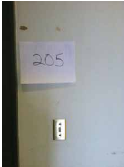
Fig. 3.1.C.9 General wear-and-tear and minor damage to plaster walls.
