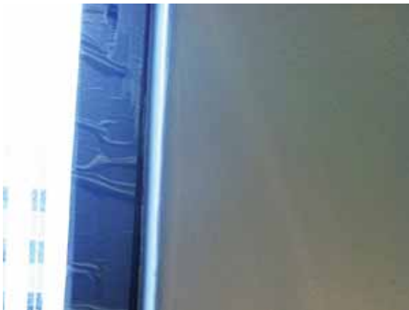
Fig. 2.1.A.28 Duct tape placed around the interior-side of the windows to prevent air leakage.
