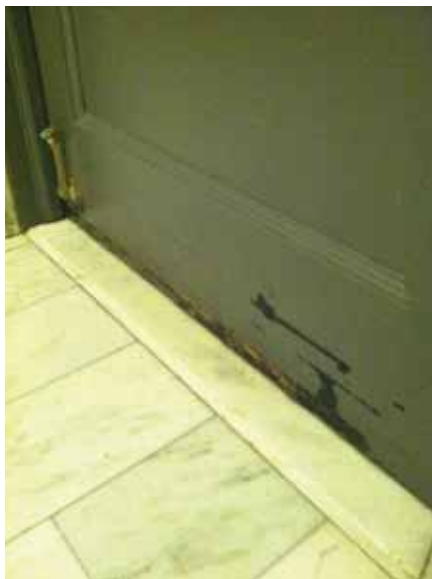
Fig. 3.1.C.40 General wear-and-tear noted at the doors.
