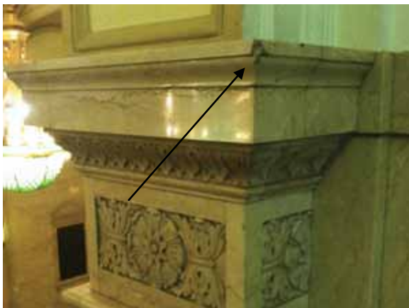
Fig. 3.1.C.13 Typical minor damage to polished stone wainscoting.
