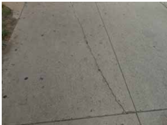
Figure 2.3.A.8 – Site Concrete Crack
