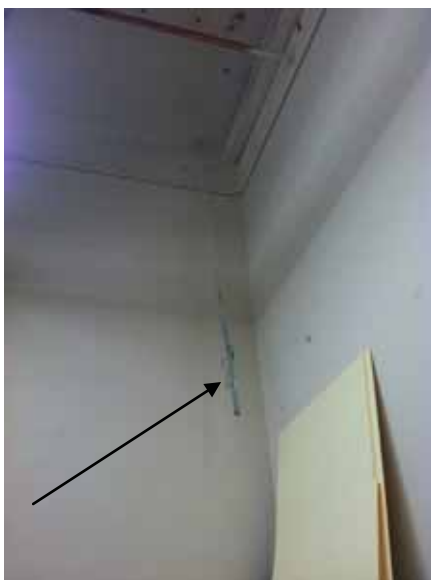
Fig. 3.1.C.5 Metal strapping hanging from the ceiling in Room B-13 Library Stacks.
