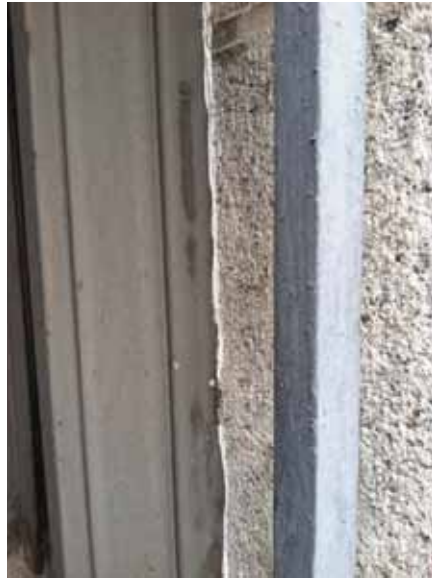
Fig. 2.1.A.24 Corroding metal window frame.
