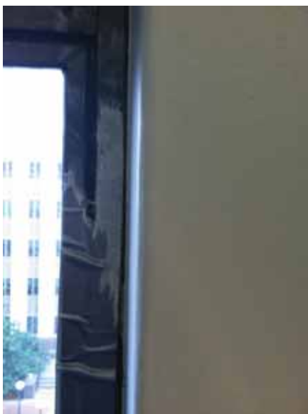
Fig. 2.1.A.29 Duct tape placed around the interior-side of the windows to prevent air leakage.
