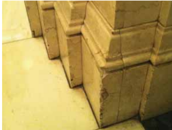
Fig. 3.1.C.8 Damaged stone observed in the central atrium space on the First Floor.
