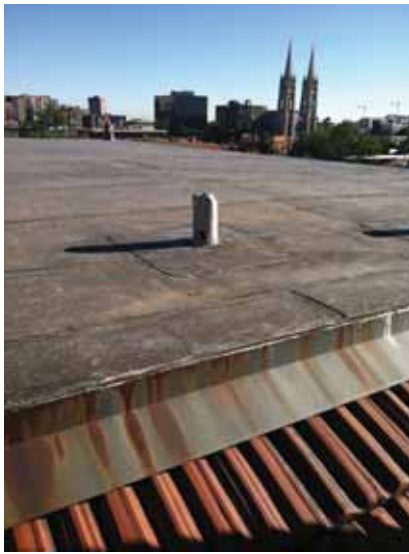
Fig. 2.1.A.23 General deterioration of the roofing materials at the flat central portion of the roof.
