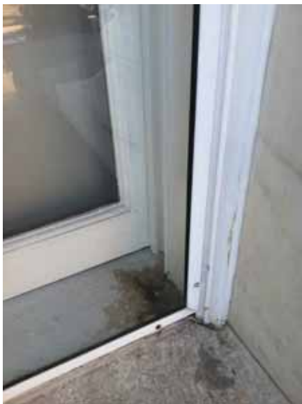
Fig. 2.1.A.11 Deterioration noted at a window sill and wear-and tear of a window frame.
