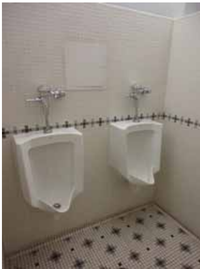
Fig. 2.1.C.2 Urinals mounted higher on the wall than allowed per accessibility requirements.
