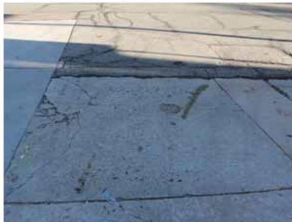
Figure 2.3.A.7 Broken Site Concrete, Recommended for Replacement
