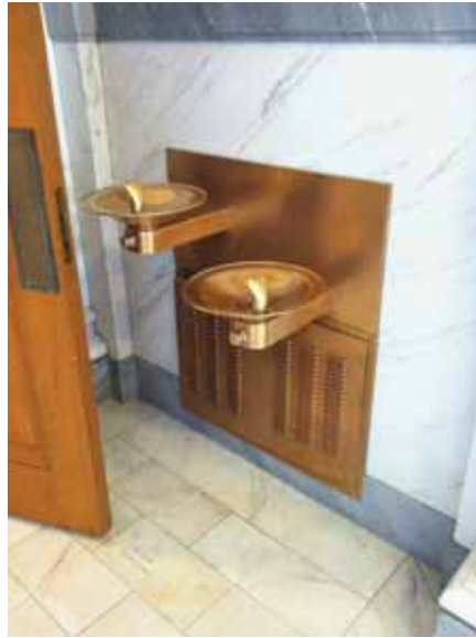
Fig. 2.1.C.9 A door appears to swing into the clear floor space of the drinking fountains on the Second Floor.
