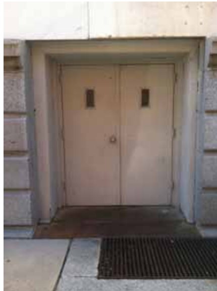
Fig. 2.1.A.18 Corroding metal sill plate noted at the pair of double doors leading to the freight elevator at the south end of the east side of the building.
