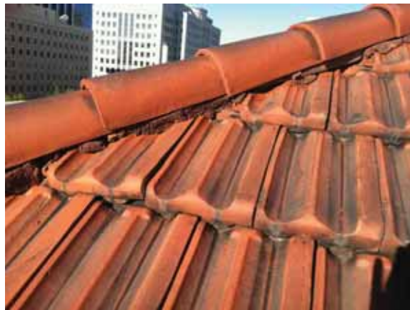
Fig. 2.1.A.26 Deterioration of the masonry along the corners of the roof is providing points by which water can penetrate the roofing membrane.
