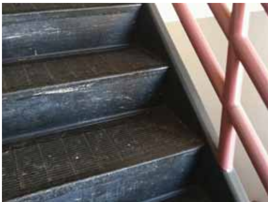
Fig. 3.1.C.26 The rubber flooring covering the stairs in the interior exit stairways has signs of general wear-and-tear throughout.
