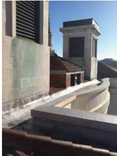
Fig. 2.1.A.19 Parapets surrounding the perimeter of the roof are lower than required by code.
