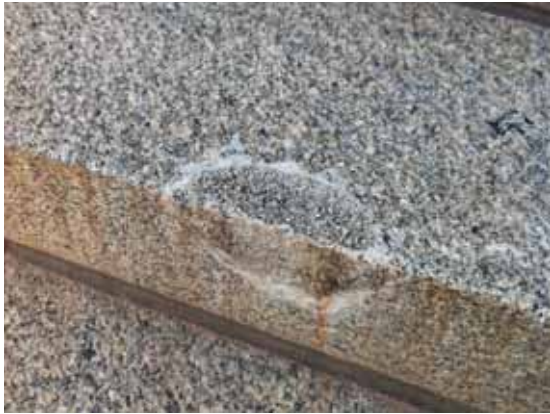
Fig. 2.1.A.32 Previously repaired damage to the granite staircase at the main East 14th Avenue Entrance.
