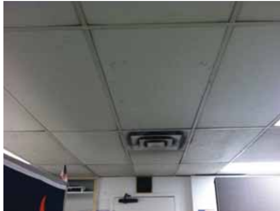
Fig. 3.1.C.1 Damaged and soiled 2x4 acoustic ceiling tiles noted throughout the Basement Floor.
