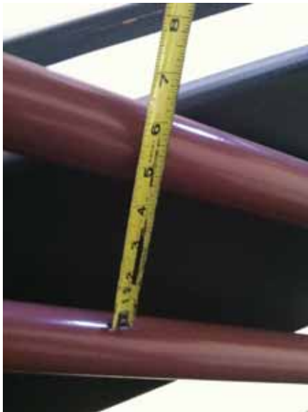
Fig. 2.1.B.2 The distance between the guardrail openings exceeds 4 inches in diameter.
