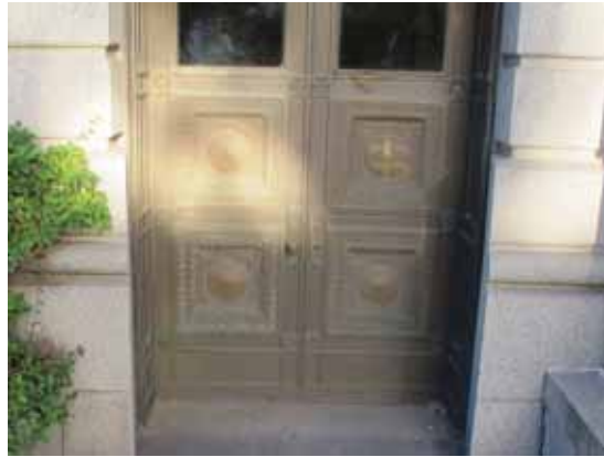
Fig. 2.1.A.17 Pair of doors on the north end of the west side of the building missing a door handle and spray-painted with graffiti.
