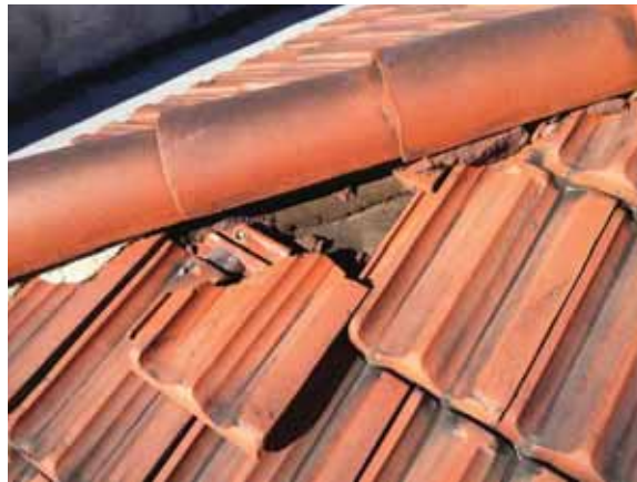
Fig. 2.1.A.25 Broken and loose clay tiles sliding down the side of the roof.
