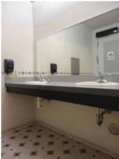
Fig. 2.1.C.3 The heights of the lavatory rims above the floor are greater than the maximum 34 inches allowed per code.
