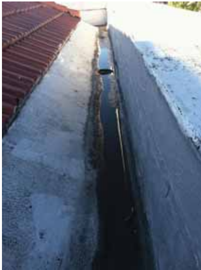
Fig. 2.1.A.29 Ponding water in the areas of the roof adjacent to the parapets.
