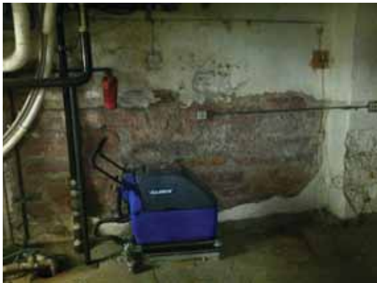
Fig. 3.1.C.15 Deterioration and damage noted to the protective brick coating in areas of the Basement Floor included in the site survey visit.
