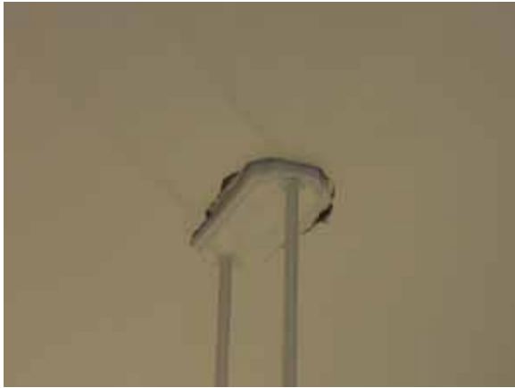
Fig. 2.4.B.3 – Cracked sheetrock around light fixture base
