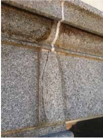
Fig. 2.1.A.6 Cracked granite observed on the east end of the north side of the building.
