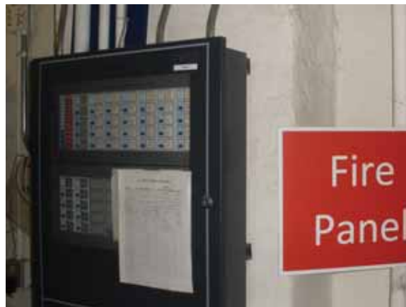
Fig. 2.4.A.8 – Fire panel in sub-basement
