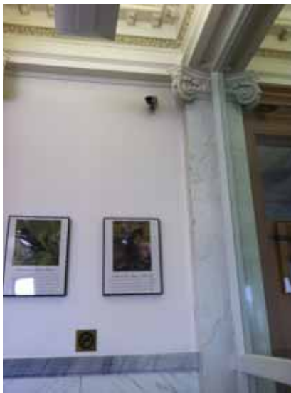
Fig. 2.1.B.9 Typical security cameras noted during the site survey visit.
