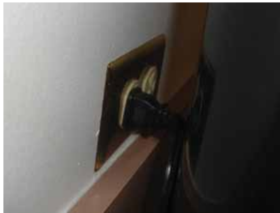
Fig. 2.4.B.6 – No GFI protection by sink
