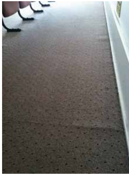
Fig. 3.1.C.21 Carpet flooring pulling loose at the seams and creating a potential tripping hazard.
