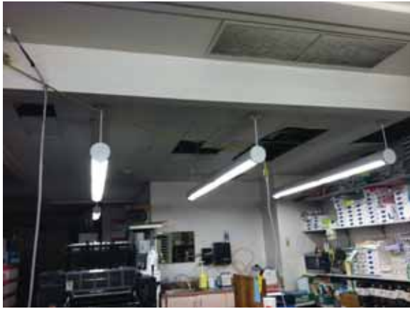
Fig. 3.1.C.4 Deteriorating, damaged, and missing 1x1 square acoustic ceiling tiles noted in the Print Shop on the Ground Floor.
