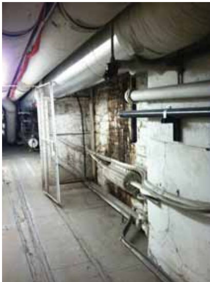
Fig. 3.1.C.16 A brown substance was noted to be dripping down a wall of the Basement Floor near the old coal tracks.
