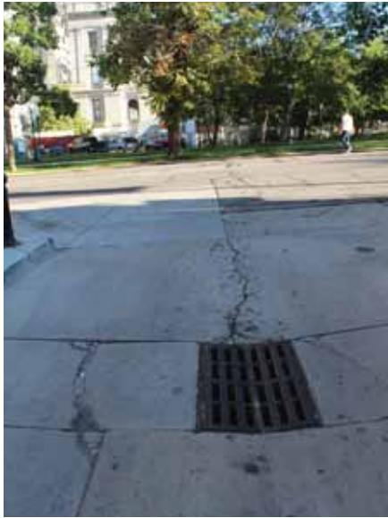
Figure 2.3.A.9 Broken Site Concrete, Recommended for Replacement
