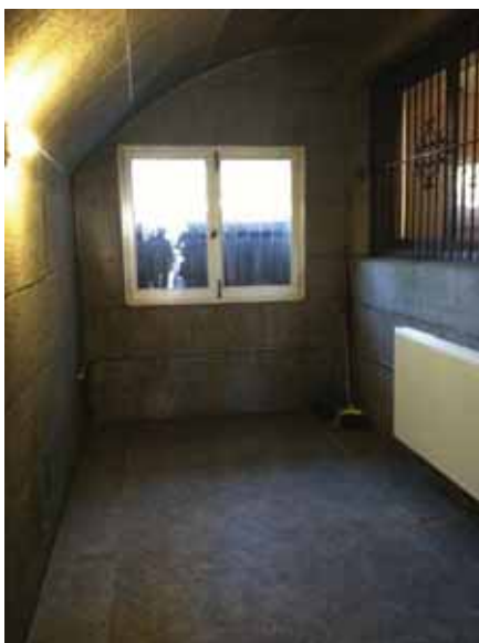
Fig. 3.1.C.6 Signs of water damage note to the granite cladding on the ceilings and walls in the Ground Floor accessible entrance vestibule on the north side of the building.
