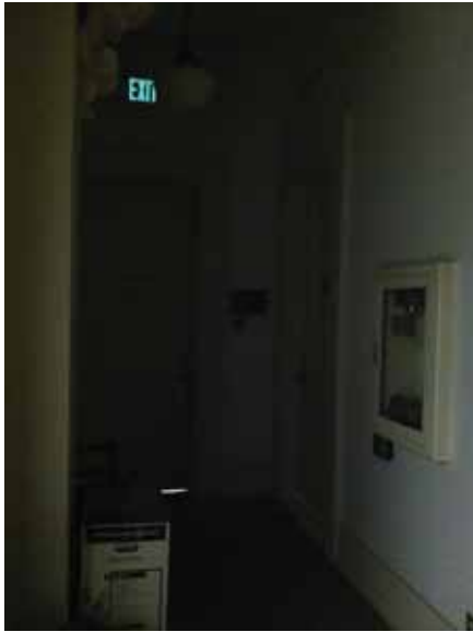
Fig. 2.1.B.1 Exit access corridor at the southwest corner of the building on the Grade Floor with inadequate illumination and with items blocking the corridor space.
