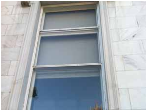
Fig. 2.1.A.10 Storm windows placed over the existing windows around the exterior of the building.
