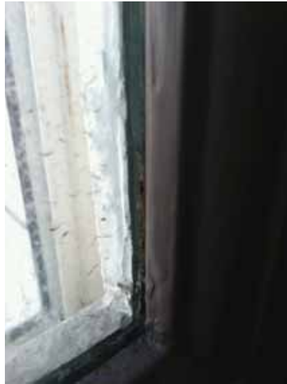
Fig. 2.1.A.12 Deteriorating original window observed during the site survey visit.
