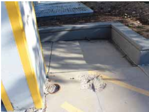
Figure 2.3.A.10 Broken Site Concrete, Recommended for Replacement
