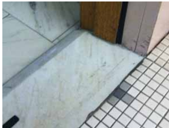
Fig. 2.1.C.5 Thresholds at the restrooms create a change in level of floor surfaces of greater than 1/2 inch high and do not comply with code requirements.
