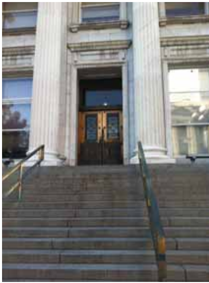
Fig. 2.1.A.33 Soiling of the granite staircase at the main East 14th Avenue Entrance.
