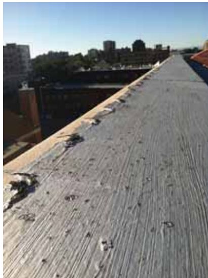
Fig. 2.1.A.20 Deterioration of the painted roofing membrane noted along the outer edge of the parapet.
