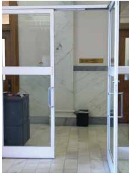
Fig. 2.1.B.7 Pull-style door handles between the lobby and office spaces found at the Second and Third Floors.
