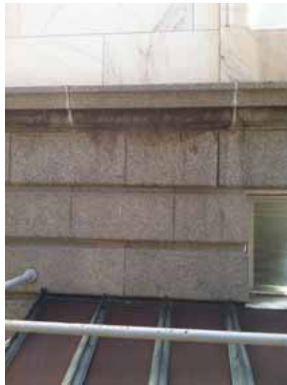
Fig. 2.1.A.3 Generally soiled granite veneer panels.
