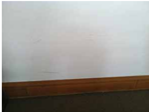
Fig. 3.1.C.11 Minor wear-and-tear noted to the plaster and gypsum board walls throughout the offices, hearing rooms, and corridors included in the site survey visit.
