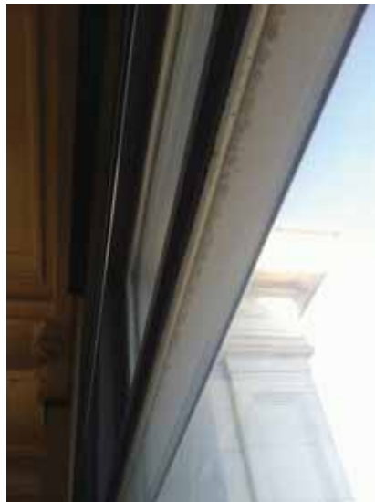
Fig. 2.1.A.13 Water damage and deterioration of the existing windows does not appear to have been addressed as part of the storm window installation project.
