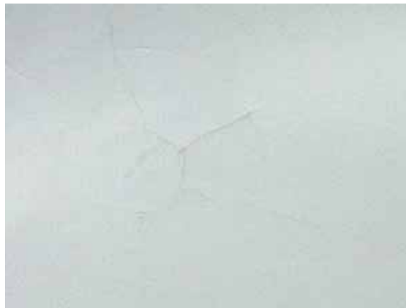
Fig. 3.1.C.12 Area of damaged plaster or gypsum board wall noted in a corridor on the Third Floor.
