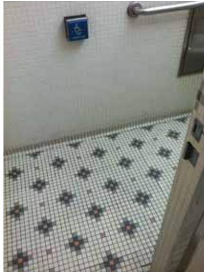
Fig. 3.1.C.27 Soiled one-inch square tile flooring noted in the restrooms throughout.
