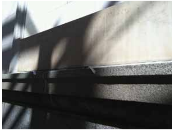
Fig. 2.1.A.9 Newer-looking sealant observed to be peeling away from the building.
