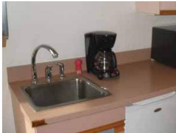
Fig. 2.4.B.5 – No GFI protection by sink
