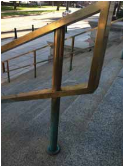
Fig. 2.1.A.34 Corroding metal railings at the East 14th Avenue exterior stairway.
