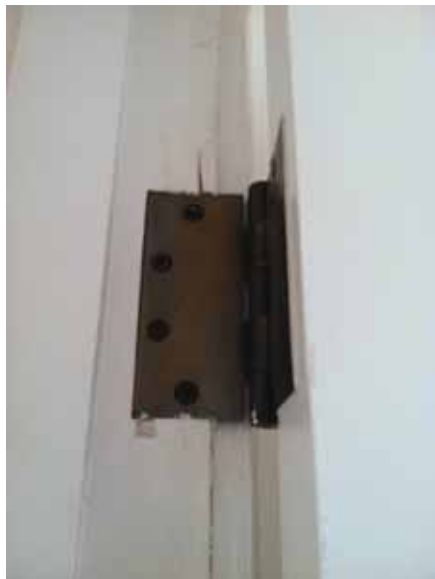
Fig. 3.1.C.30 Cracking door frame at the hinge noted during the site survey visit.
