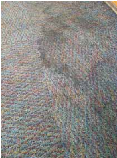
Fig. 3.1.C.20 Soiled and deteriorating carpet noted in areas throughout the building.
