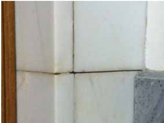
Fig. 3.1.C.9 Areas of deteriorating or missing grout at the marble wainscoting throughout.
