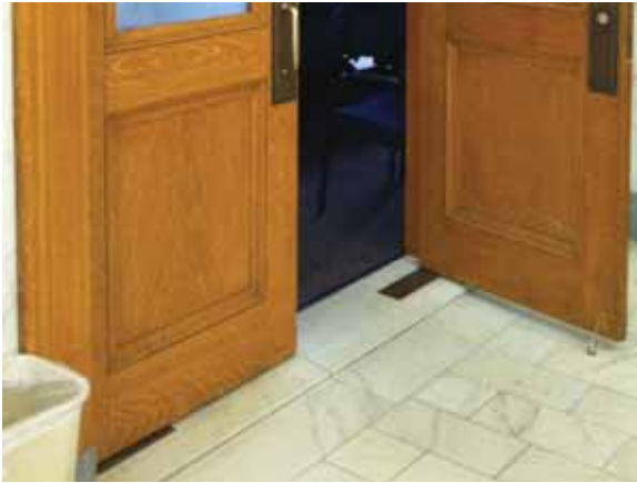
Fig. 2.1.C.7 Thresholds between the lobby spaces and surrounding spaces create a change in level of floor surfaces of greater than 1/2 inch high and do not comply with code requirements.
