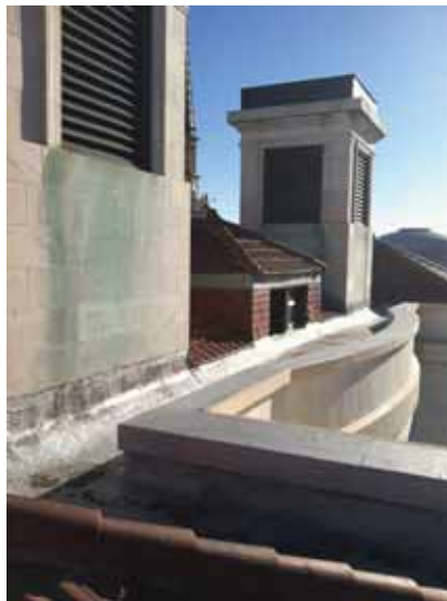
Fig. 2.1.A.4 Soiled marble veneer panels observed at the roof level.
