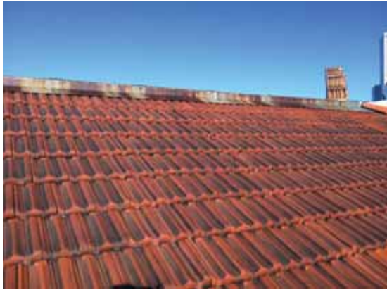
Fig. 2.1.A.28 Widespread corrosion of the flashing was observed around the roof.
