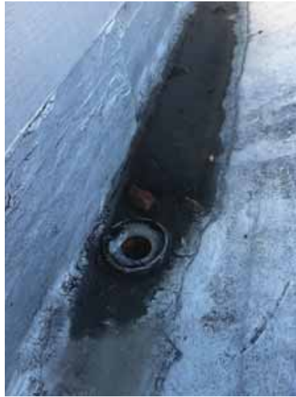
Fig. 2.1.A.31 Missing roof drain covers noted in spots around the perimeter of the roof.
