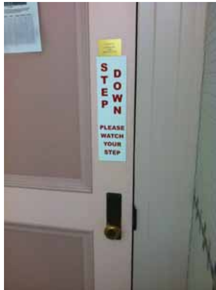
Fig. 2.1.C.4 Thresholds at the restrooms create a change in level of floor surfaces of greater than 1/2 inch high and do not comply with code requirements.
