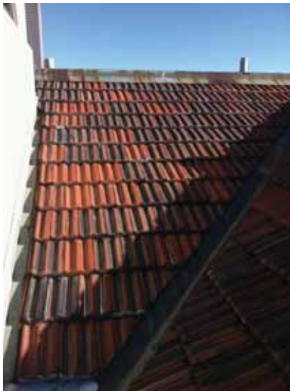
Fig. 2.1.A.24 Typical soiling noted of the clay tiles covering the shallow hipped sections of the roof.
