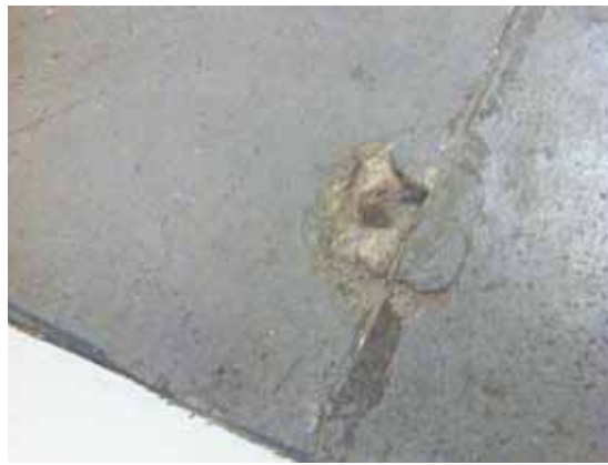
Fig. 3.1.C.28 Spalling concrete flooring noted in the basement.
