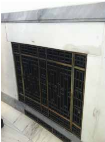
Fig. 3.1.C.10 Damage and wear-and-tear noted to the marble wainscoting around a metal grill at the grand central stairway.
