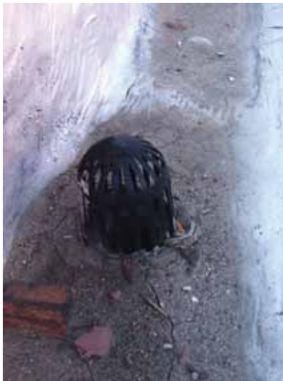
Fig. 2.1.A.30 Dirt and debris accumulating in the areas of the roof adjacent to the parapets.
