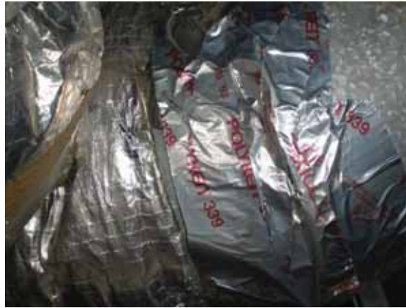
Fig. 2.4.A.12 – Air leakage from duct joint
