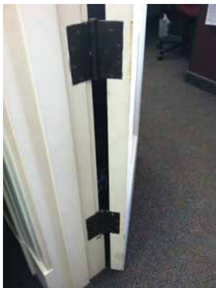
Fig. 3.1.C.31 General wear-and-tear noted at a door during the site survey visit.
