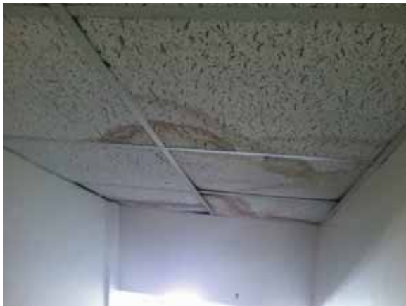
Fig. 3.1.C.5 2x4 acoustic ceiling tiles in poor condition within the interior exit stairway at the attic landing.
