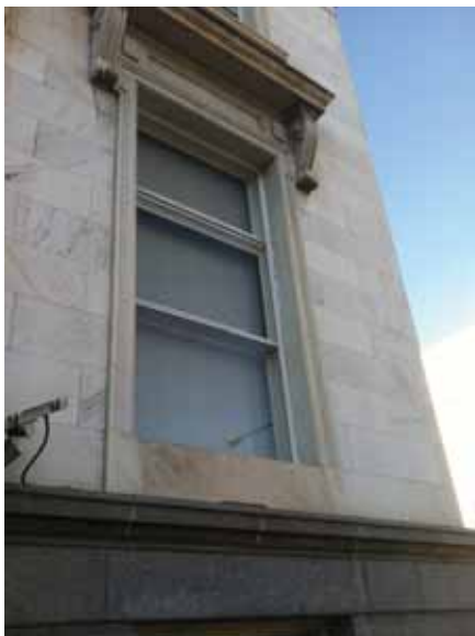
Fig. 2.1.A.2 Typical instance of soiled marble around the windows.
