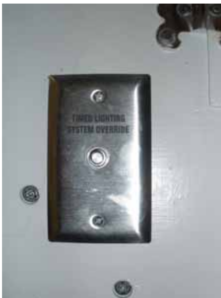
Fig. 2.4.A.6 – Lighting override button
