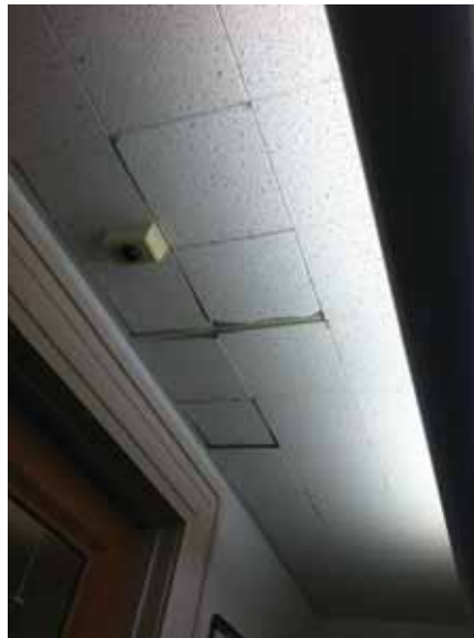
Fig. 3.1.C.2 Deteriorating and damaged 1x1 square acoustic ceiling tiles.
