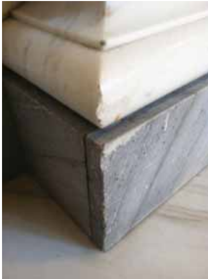
Fig. 3.1.C.8 Areas of damaged marble wainscoting and cladding noted throughout the building.
