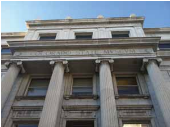
Fig. 2.1.A.1 Generally soiled marble cladding around the building's exterior.
