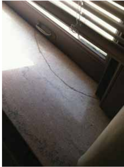
Fig. 3.1.C.32 Cracked stone window sill noted during the site survey visit.
