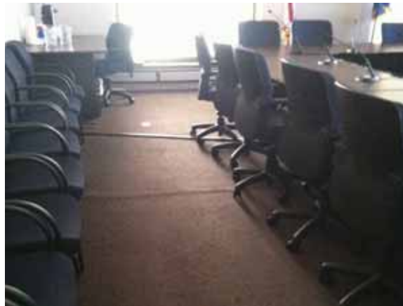
Fig. 3.1.C.22 Carpet flooring pulling loose and bunching together, creating a potential tripping hazard.
