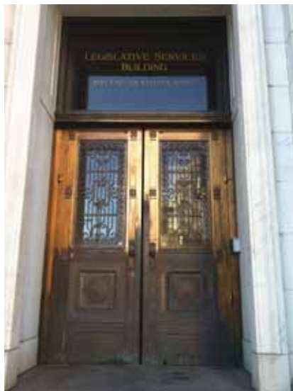
Fig. 2.1.A.16 The bottom half of the main East 14th Avenue Entrance doors have become tarnished over the years.
