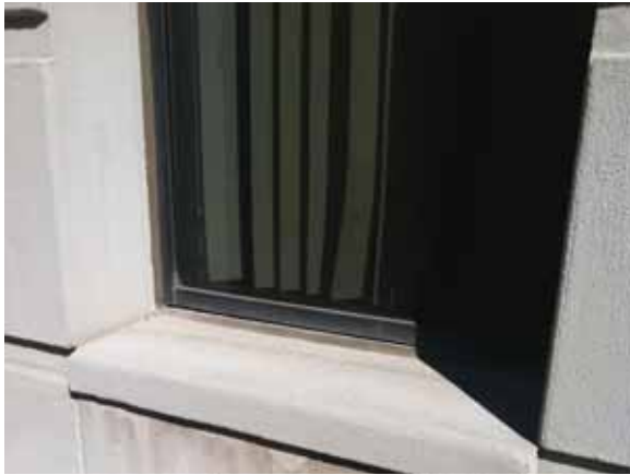
Fig. 2.1.A.11 Typical gaps observed at the bottom of a window frame, exposing the building envelope to the elements.
