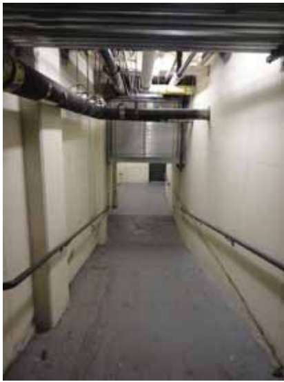
Fig. 3.0.C.27 Generally worn, cracking, and spalling concrete flooring with signs of water damage on the Basement Floor.
