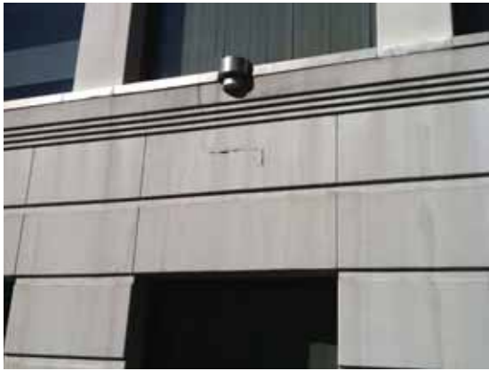
Fig. 2.1.A.3 Damaged, cracked, and soiled stucco noted around the exterior of the building.
