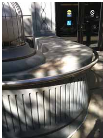
Fig. 2.1.A.31 Typical instance of deteriorating coating noted at the low concrete retaining walls.
