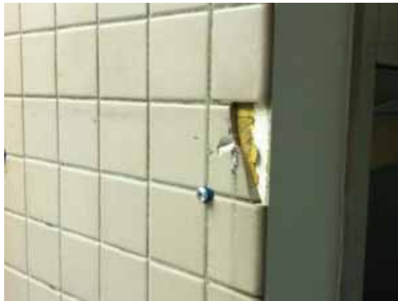
Fig. 3.0.C.14 Damaged and missing two-inch square wall tile noted throughout the restrooms during the site survey visit.
