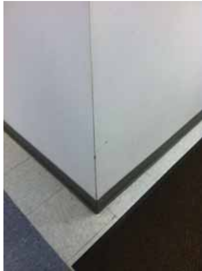
Fig. 3.0.C.7 Typical instance of minor wear-and-tear noted to the gypsum board walls.
