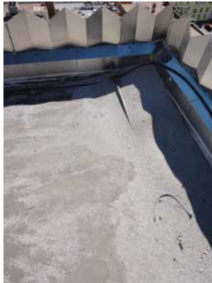
Fig. 2.1.A.17 Piles of aggregate separating from the roofing membrane are collecting at the corners of the roof.
