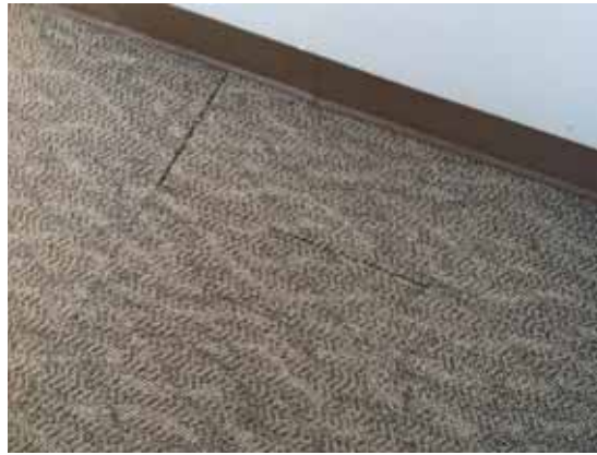
Fig. 3.0.C.18 Worn carpet with seams pulling loose and creating a potential tripping hazard.
