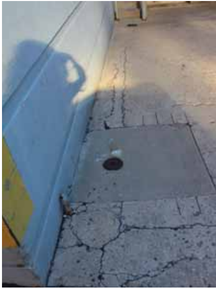
Figure 2.3.A.9 Broken Site Concrete, Recommended for Replacement
