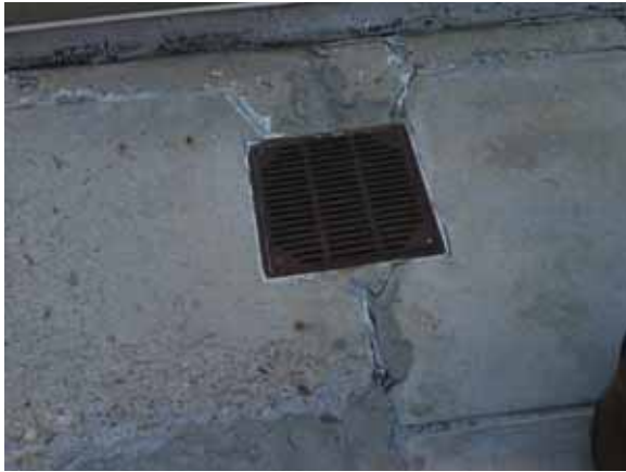
Fig. 2.1.A.8 Spalling concrete pavers located at the Ninth Floor patio and creating a potential tripping hazard.
