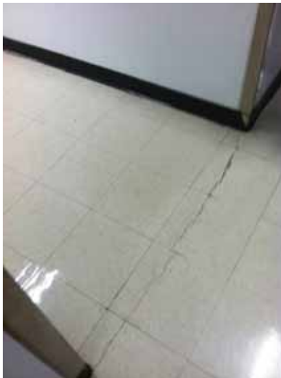
Fig. 3.0.C.22 An instance of cracked linoleum tile observed during the site survey visit.
