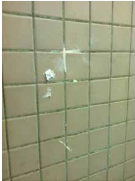
Fig. 3.0.C.13 Generally soiled areas of the two-inch square wall tile noted throughout the restrooms during the site survey visit.
