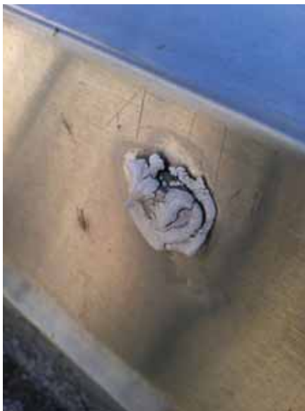
Fig. 2.1.A.27 Typical deterioration of the sealant over the fasteners anchoring the perimeter flashing at the roof parapets.
