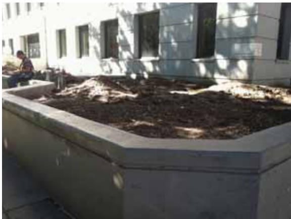
Fig. 2.1.A.29 Typical wear-and-tear and deterioration of the low concrete retaining walls around the exterior of the building.
