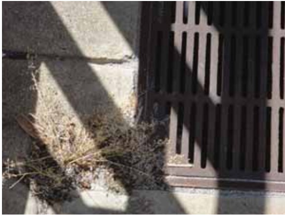
Fig. 2.1.A.25 Corroding drain cover located at the Ninth Floor patio with soil collecting nearby and allowing the growth of weeds.
