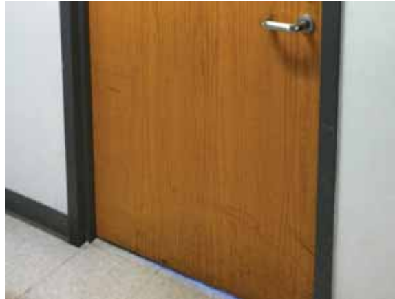
Fig. 3.0.C.29 Minor wear-and-tear observed to some of the doors throughout the building.
