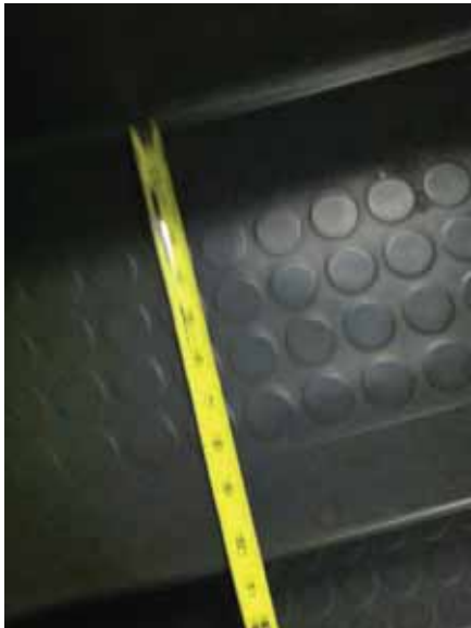
Fig. 2.1.B.4 Existing stair tread depths do not meet current code requirements.
