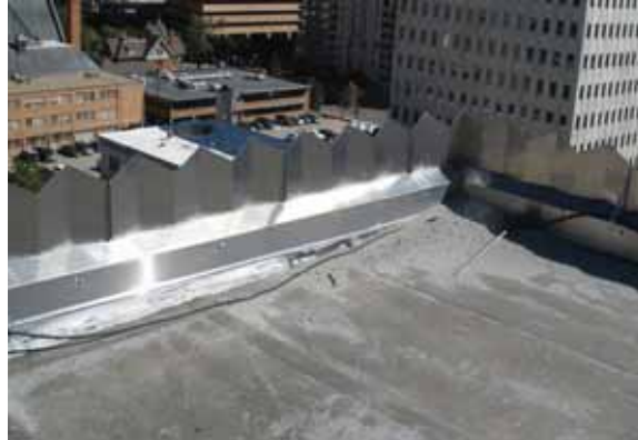
Fig. 2.4.B.1 – Broken air terminals and wire hanging
