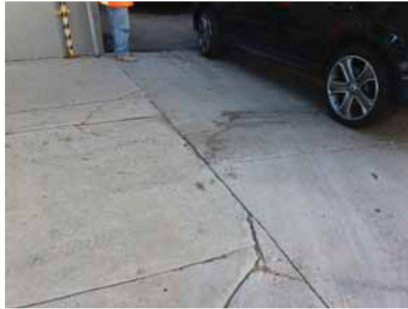
Figure 2.3.A.6 Site Concrete Crack
