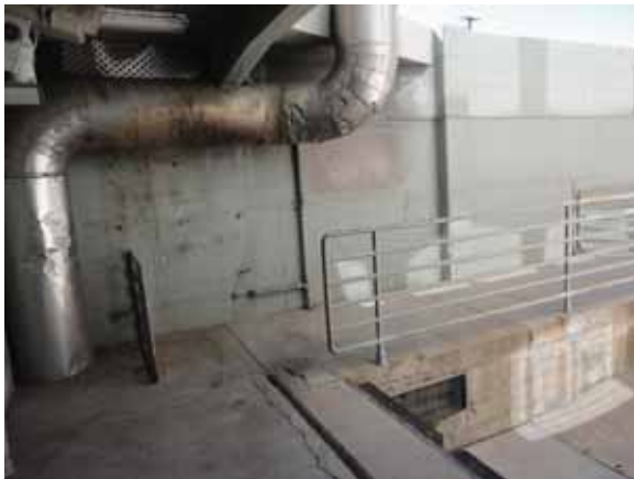
Fig. 2.1.A.34 Spalling and cracking concrete and corroding guardrail noted at the south loading dock.
