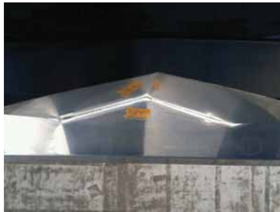
Fig. 2.1.A.23 Spots of corrosion and deteriorating sealant observed around the triangular, folded, decorative metal piece installed around the top perimeter of the Penthouse parapet.
