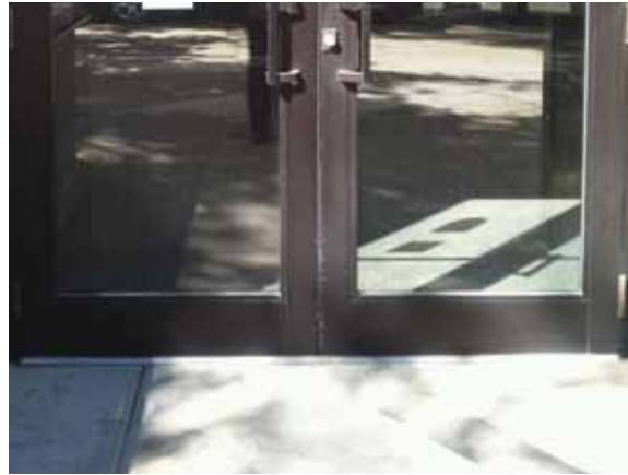
Fig. 2.1.A.14 The weatherstripping at the exterior doors is starting to deteriorate around the building.
