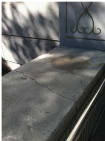
Fig. 2.1.A.30 Cracked concrete coping noted in a few spots along the low retaining walls during the site survey visit.
