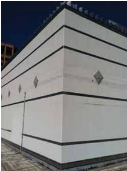
Fig. 2.1.A.4 Cracked and worn stucco noted at the Penthouse on the roof.
