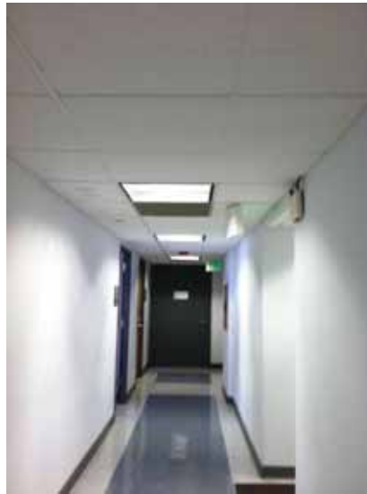
Fig. 3.0.C.4 Sagging ceiling tiles noted during the site survey visit.
