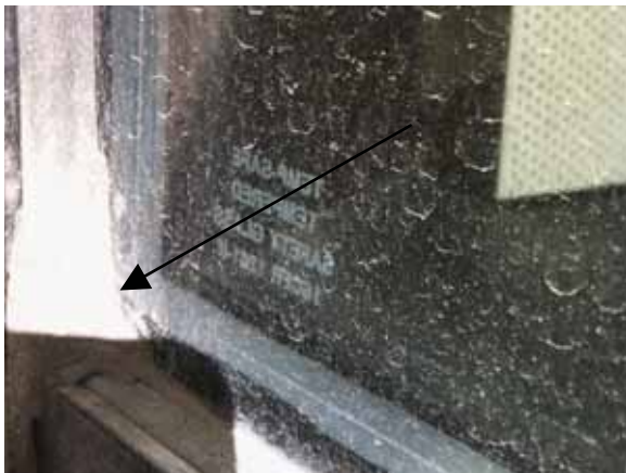
Fig. 2.1.A.12 The material used for previous repairs to the corner joints of the metal window frames appears to be deteriorating.
