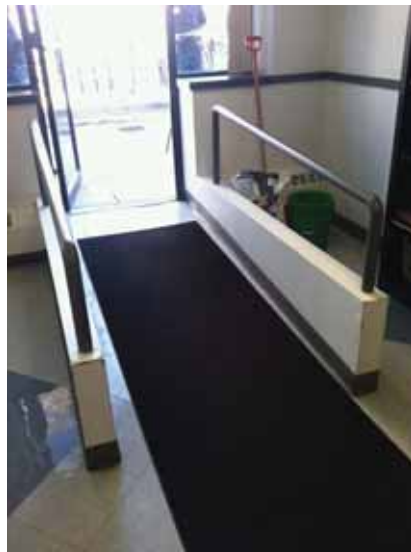
Fig. 3.0.C.8 Wear-and-tear noted to the low gypsum board walls on either side of the ramp to the Ninth Floor patio.
