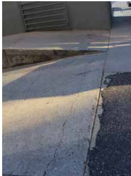
Figure 2.3.A.7 Site Concrete Crack
