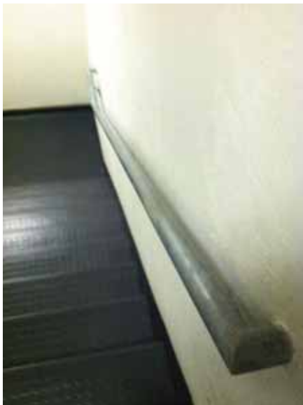
Fig. 3.0.C.32 Minor corrosion noted to the railings throughout the stairways.
