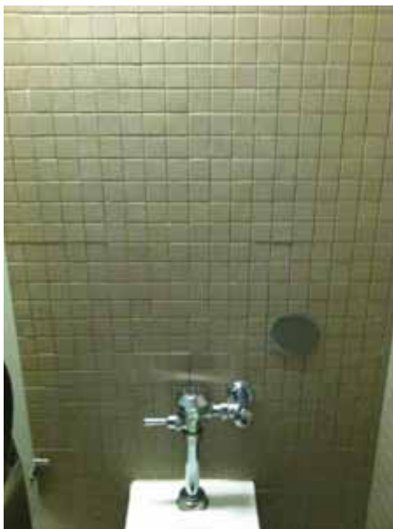
Fig. 3.0.C.12 Pieces of the two-inch square wall tile throughout the restrooms appear to be moving out and away from the wall.
