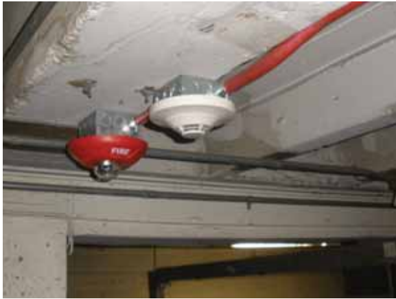
Fig. 2.4.A.4 – Smoke detector and horn strobe
