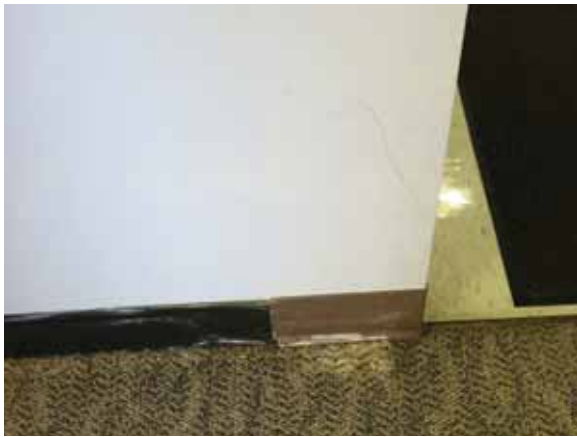
Fig. 3.0.C.11 Instance of mismatched vinyl baseboard noted during the site survey visit.
