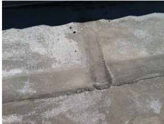
Fig. 2.1.A.16 General deterioration of the roofing membrane noted overall.
