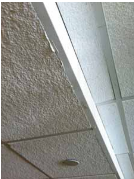
Fig. 3.0.C.2 Deteriorating ceiling tiles noted during the site survey visit.
