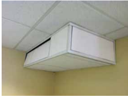
Fig. 3.0.C.3 Deteriorating ceiling tiles noted during the site survey visit.
