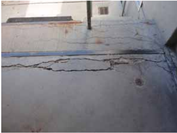
Fig. 2.1.A.33 Spalling and cracking concrete noted at the south loading dock.
