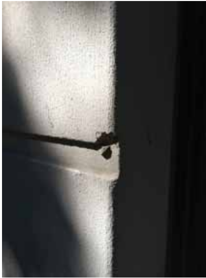
Fig. 2.1.A.2 Spalling of the stucco panels noted around the exterior of the building.
