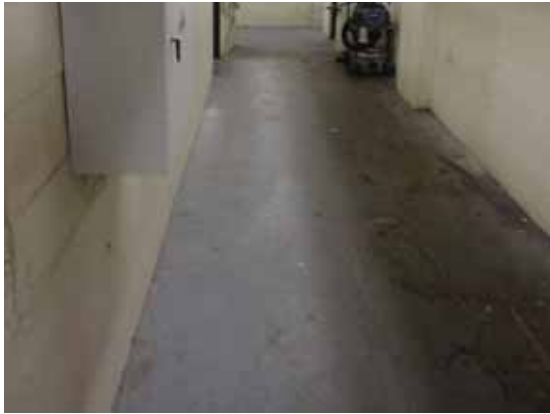
Fig. 3.0.C.26 Generally worn and spalling concrete flooring with signs of water damage on the Basement Floor.
