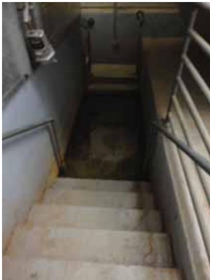
Fig. 3.0.C.28 Evidence of water damage noted on the Basement Floor.
