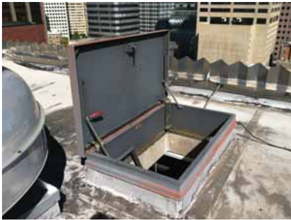
Fig. 2.1.A.20 Corroding access hatch at the Penthouse roof.
