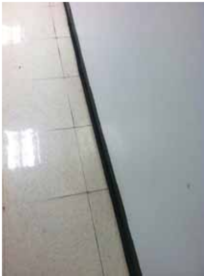
Fig. 3.0.C.21 An instance of deteriorating and soiled linoleum along the edges of the tiles.
