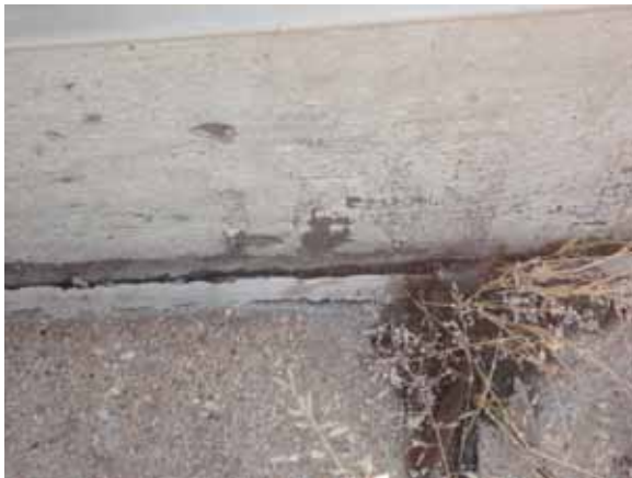
Fig. 2.1.A.9 Deteriorating sealant between the building's walls and the concrete pavers at the Ninth Floor patio.
