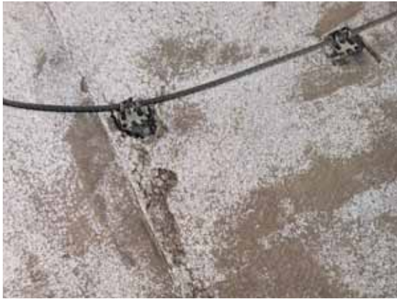
Fig. 2.1.A.19 Deterioration around the metal attachment clips of the lightning protection cable.
