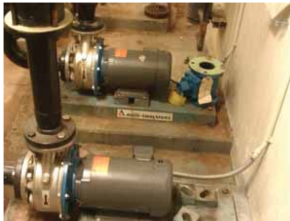
Fig. 2.4.A.9 – Missing insulation on pipes
