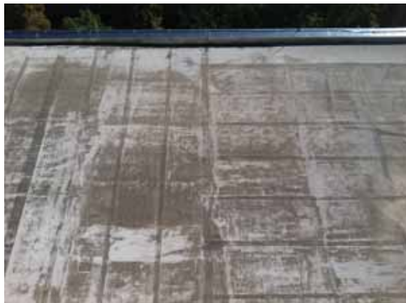
Fig. 2.1.A.15 General deterioration of the roofing membrane noted overall.
