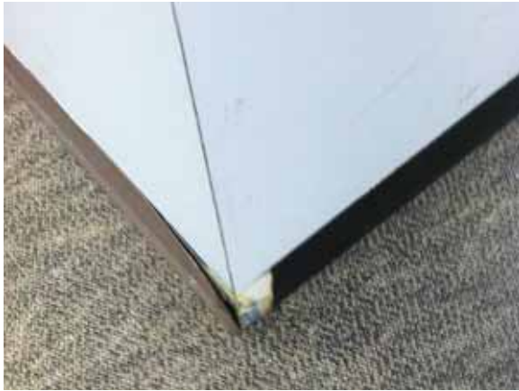
Fig. 3.0.C.10 Instance of damaged vinyl baseboard missing and peeling away from the wall.
