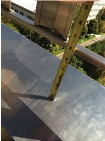
Fig. 2.1.B.3 The distance between the guardrail openings at the Ninth Floor patio exceeds 4 inches in diameter.
