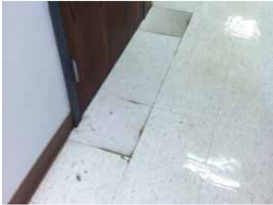
Fig. 3.0.C.20 An instance of soiled and damaged linoleum tile observed during the site survey visit.
