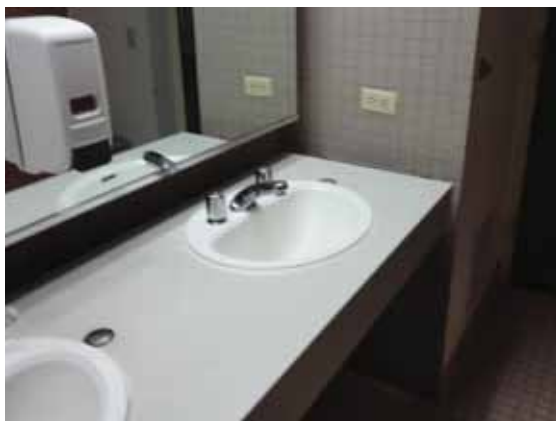
Fig. 2.1.C.3 Typical instance of an electrical receptacle, not equipped with ground-fault circuit interrupter protection, located within 6 feet of the edge of a sink.
