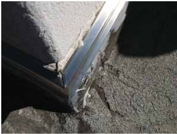
Fig. 2.1.A.26 Typical deterioration of the sealant noted at the flashing around the roof.
