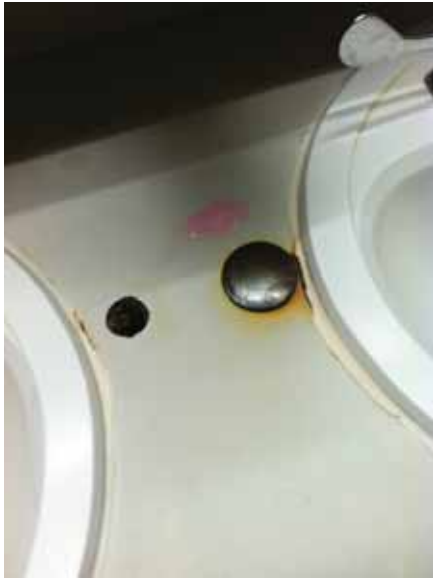
Fig. 3.0.C.31 Typical wear-and-tear and deterioration due to aging of the restroom countertops.
