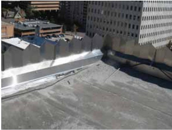
Fig. 2.4.A.1 – Broken air terminals
