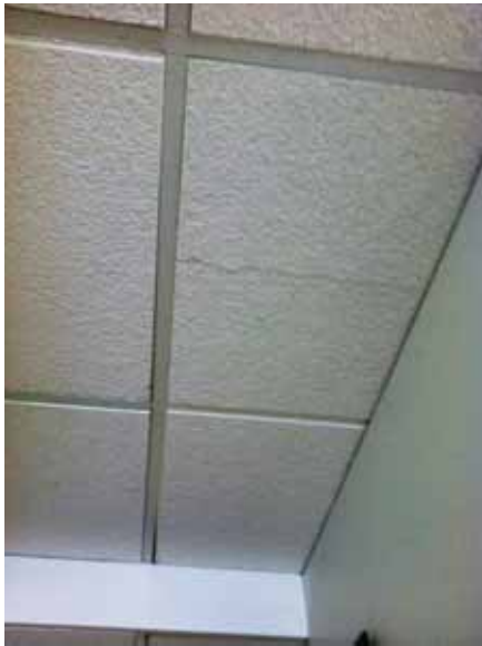
Fig. 3.0.C.1 Typical cracked acoustic ceiling tile noted during the site survey visit.
