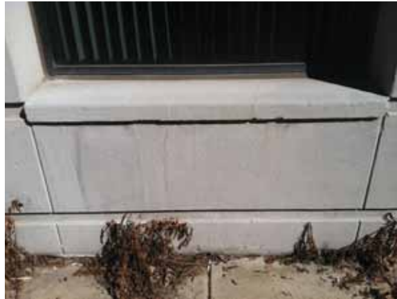
Fig. 2.1.A.5 Soiled, cracked, and spalled stucco noted around the exterior of the building.
