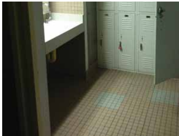
Fig. 3.0.C.24 Generally soiled 2-inch square floor tile noted in the restrooms throughout.
