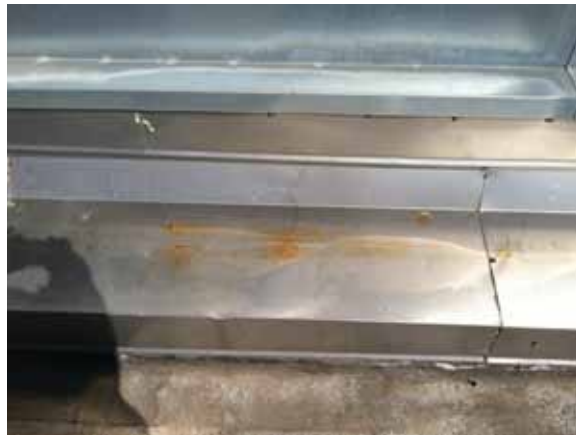
Fig. 2.1.A.22 Corrosion of the flashing noted during the site survey visit.
