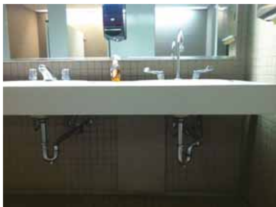
Fig. 2.1.C.1 Typical instance of an accessible lavatory without insulation wrapped around the pipes.
