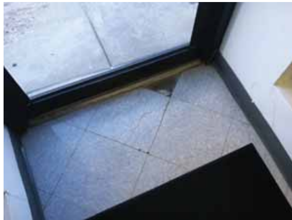
Fig. 3.0.C.23 Deteriorating and damaged linoleum tile noted at the ramp leading to the Ninth Floor patio.
