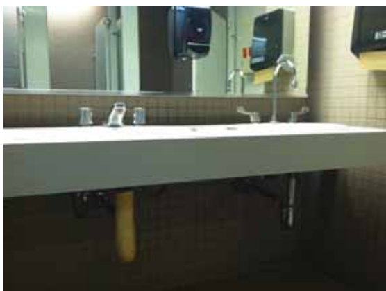
Fig. 2.1.C.2 The non-accessible lavatory in the Women's Ground Floor Restroom is wrapped with insulation around the pipes while the accessible lavatory has no insulation wrapped around the pipes.
