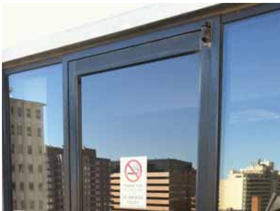
Fig. 2.1.A.13 Minor corrosion noted at the exterior doors.
