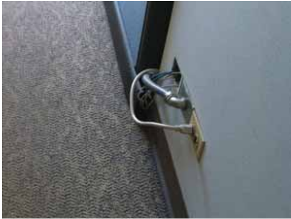
Fig. 3.0.C.16 Cables observed coming out of an unfinished hole in the wall in the Tenth Floor office area.
