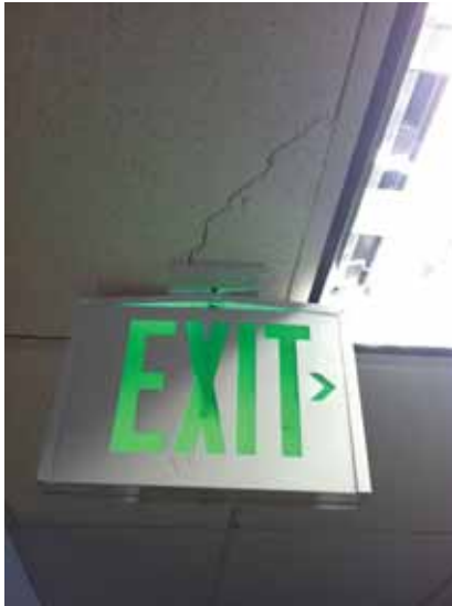
Fig. 3.0.C.6 Typical instance of a cracked acoustic ceiling tile noted at an exit sign that does not appear to be properly secured to the ceiling, creating an unsafe working condition for building occupants.
