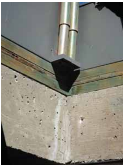
Fig. 2.1.A.21 Spalling concrete and evidence of water infiltration noted just inside the access hatch to the Penthouse roof.
