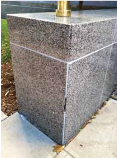
Fig. 2.1.A.36 New sealant that abruptly stops, leaving the wall exposed to water penetration.
