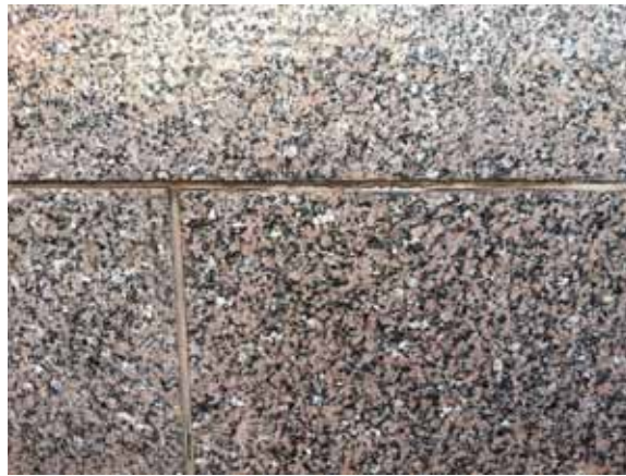
Fig. 2.1.A.34 Typical instance of deteriorating sealant noted at the granite cladding on the low walls around the building.
