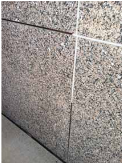
Fig. 2.1.A.9 New sealant that abruptly stops, leaving large gaps between the stone and the base of the building exposed to water penetration.
