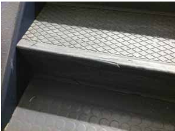
Fig. 3.0.C.20 Deteriorating rubber flooring noted on the stairs.
