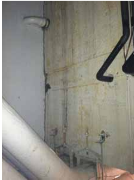
Fig. 3.0.C.12 Water damage noted at the walls near the emergency exit on the Sub-basement Floor.
