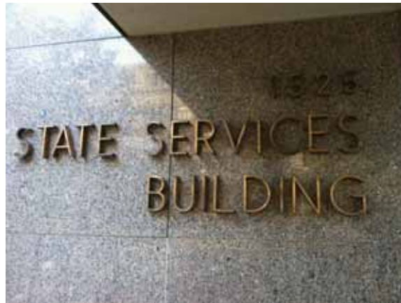
Fig. 2.1.A.40 Soiled brass building signage noted at the Sherman Street Entrance.
