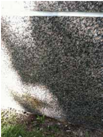
Fig. 2.1.A.4 Cracked granite panel observed during the site survey visit.
