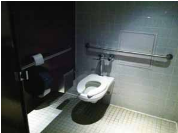
Fig. 3.0.C.19 Areas of soiling noted at the two-inch square floor tile in the restrooms.
