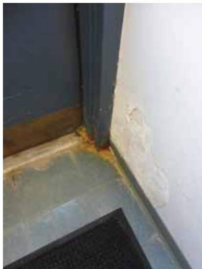
Fig. 3.0.C.4 Water-damaged gypsum board noted near the emergency exit on the west end of the north side of the Ground Floor.
