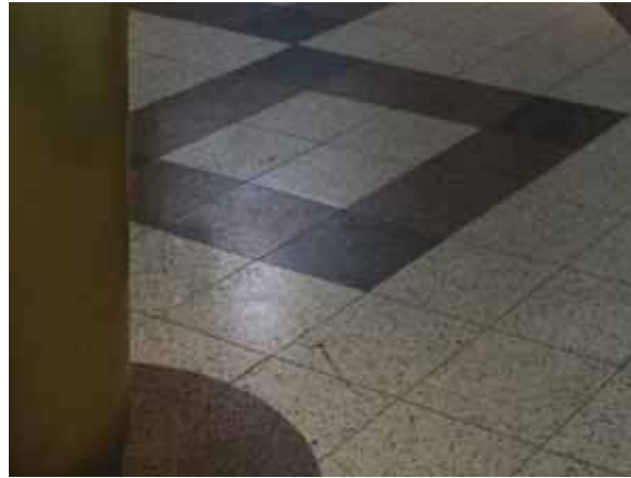
Fig. 3.0.C.15 Areas of soiling and damage noted at the granite tile flooring in the elevator lobbies.
