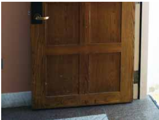
Fig. 3.0.C.25 General wear-and-tear noted at the doors.
