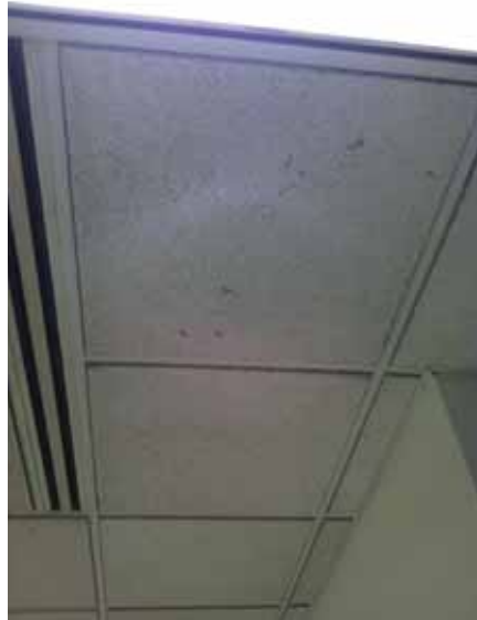
Fig. 3.0.C.2 General wear-and-tear and aging of the acoustic ceilings noted throughout.
