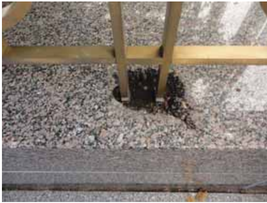
Fig. 2.1.A.37 Sealant or mortar is deteriorating and missing at the guardrail connections to the granite walls at the Sherman Street Entrance and is allowing standing water.
