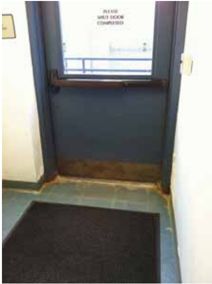
Fig. 2.1.A.20 Water damage observed at the interior side of the emergency door on the west end of the north side of the building.
