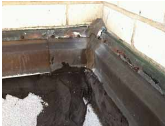
Fig. 2.1.A.31 General corrosion and deterioration of the flashing noted around the roof.
