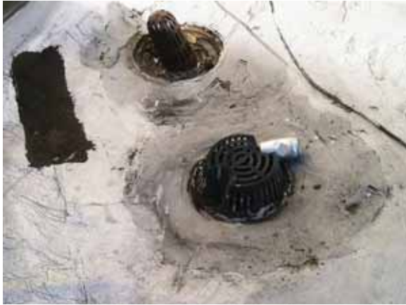
Fig. 2.1.A.29 Debris observed to be collecting near a roof drain.
