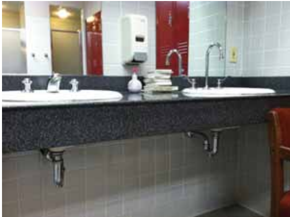
Fig. 2.1.C.2 Typical instance of insulation missing entirely from the pipes of an accessible lavatory.
