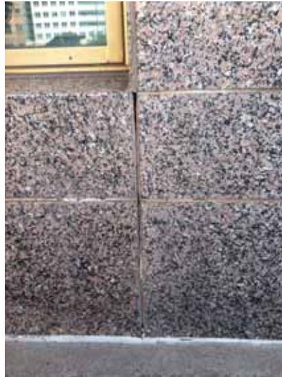
Fig. 2.1.A.5 Typical instance of deteriorating and missing sealant noted at the granite panels around the exterior of the building.
