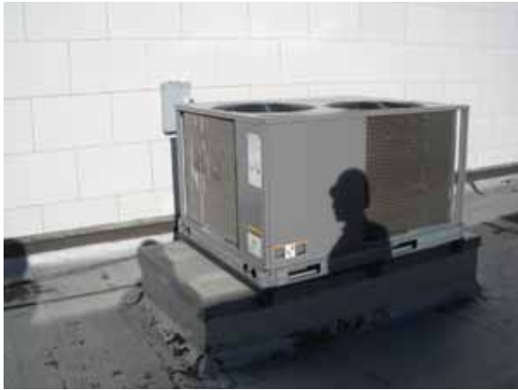
Fig. 2.4.A.15 – Condensing unit with damaged fins
