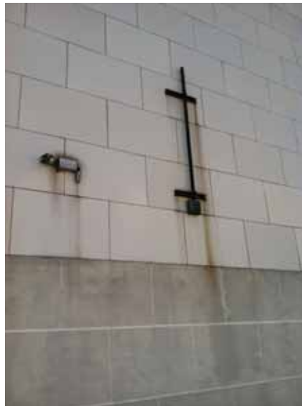
Fig. 2.1.A.12 Soiling and staining of the tile cladding on the Penthouse walls caused by the corrosion of metal equipment mounted to the walls.
