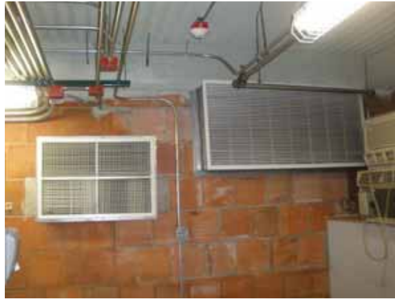
Fig. 2.4.A.12 – Supply and return grilles serving elevator machine room
