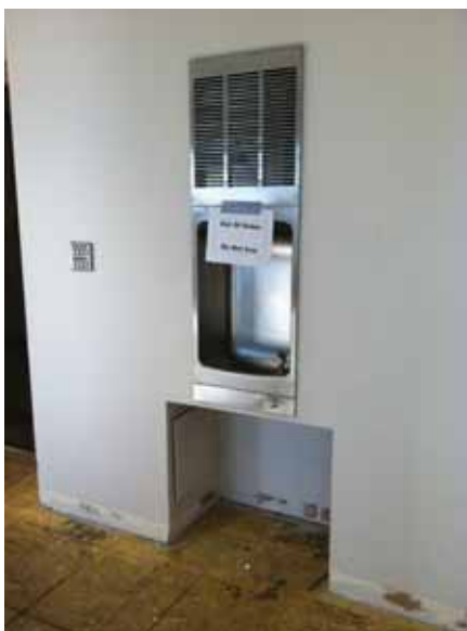
Fig. 2.1.C.3 Generally accessible drinking fountain with the exception of the clear space provided underneath.
