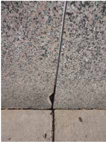
Fig. 2.1.A.3 Damaged granite panel observed during the site survey visit.
