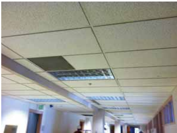
Fig. 3.0.C.1 General deterioration and aging of the acoustic ceilings noted throughout.
