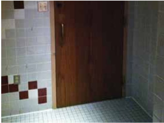
Fig. 3.0.C.9 Soiling of the four-inch square tile wainscoting noted in areas of the restrooms.
