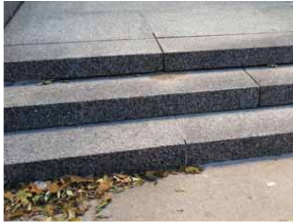
Fig. 2.1.A.33 Sealant deteriorating or missing entirely from the joints between the granite at the Sherman Street Entrance stairway.
