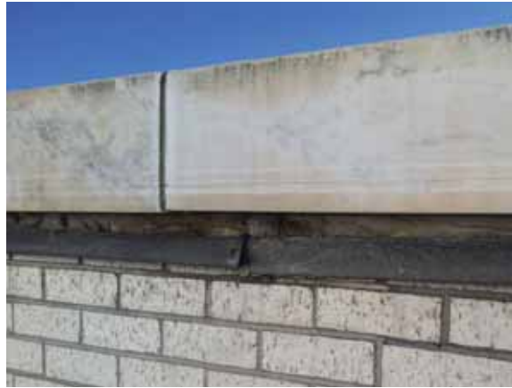
Fig. 2.1.A.17 Deteriorating mortar observed under the marble blocks along the top edge of the roof parapet.
