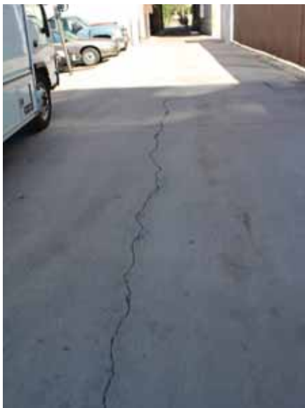
Figure 2.3.A.8 Concrete Crack in alleyway, Recommended for Repair or Replacement
