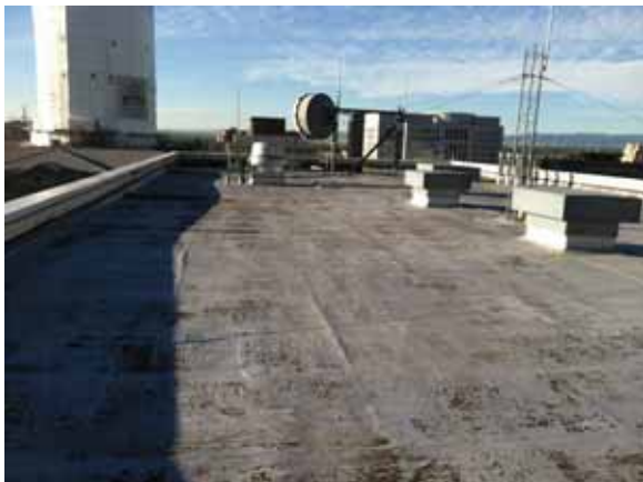
Fig. 2.1.A.24 Typical overall deterioration of the roofing membrane.
