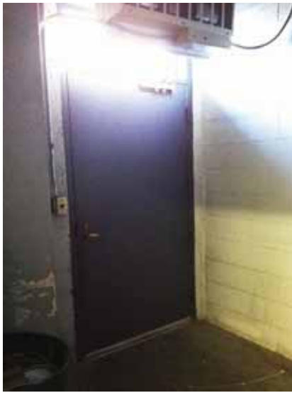
Fig. 3.0.C.10 General wear-and-tear noted at the walls in the loading dock area on the Ground Floor.
