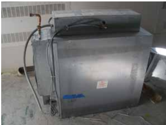
Fig. 2.4.A.22 – Existing VAV box stored in the construction area
