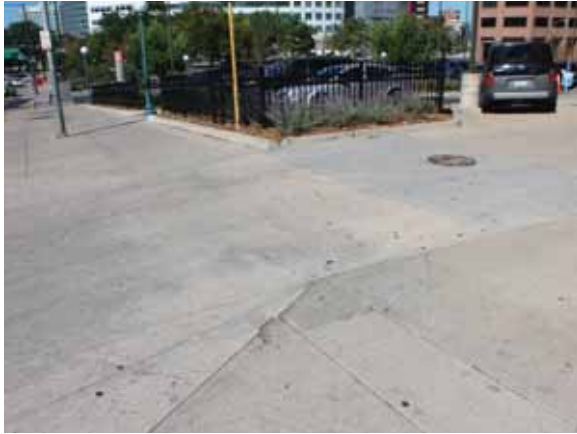
Figure 2.3.A.7 Broken Site Concrete
