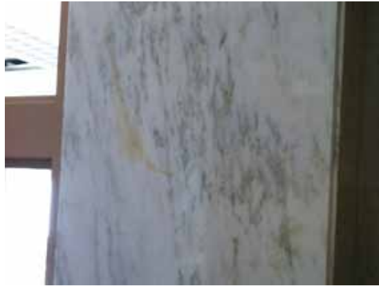
Fig. 3.0.C.6 Areas of soiled marble cladding on the walls noted in the elevator lobbies throughout.
