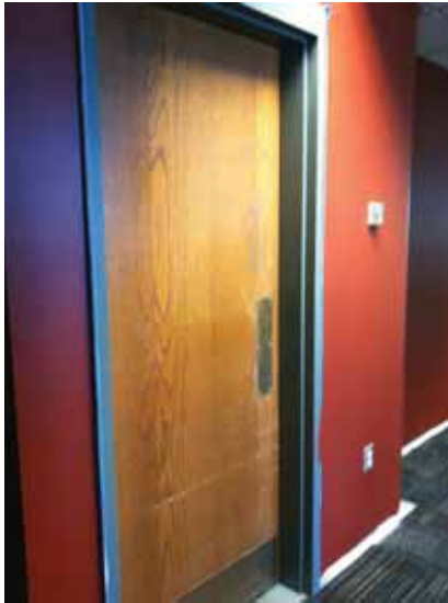
Fig. 3.0.C.24 General wear-and-tear noted at the doors.
