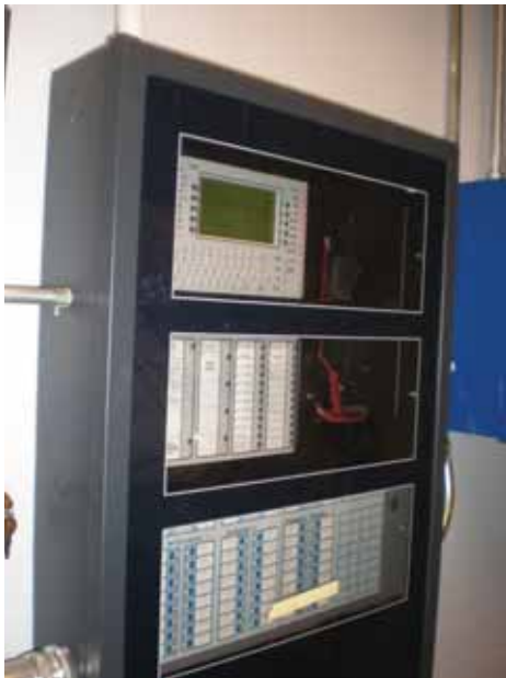
Fig. 2.4.A.6 – Fire alarm control panel
