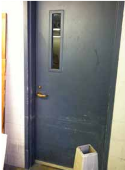
Fig. 3.0.C.26 Wear-and-tear noted at the doors in the loading dock area on the Ground Floor.
