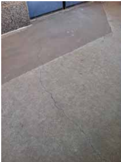
Fig. 2.1.A.38 A large crack noted at the concrete landing of the employee entrance at the north end of the west side of the building.
