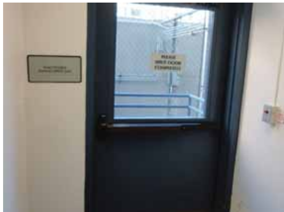
Fig. 2.1.B.1 Pushing the button of a locking device is required to open the Ground Floor emergency exit door located at the west end of the north side of the building.
