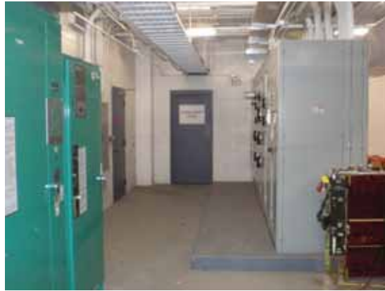
Fig. 2.4.A.2 – Main electrical gear
