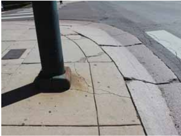
Figure 2.3.A.6 Site Concrete Crack
