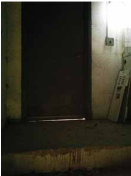
Fig. 2.1.A.21 Daylight is visible along the bottom edge of the emergency door on the east end of the north side of the building and evidence of water damage was observed on the interior side of the door.
