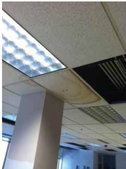
Fig. 3.0.C.3 Water damage to the acoustic ceiling noted in spots throughout the building.
