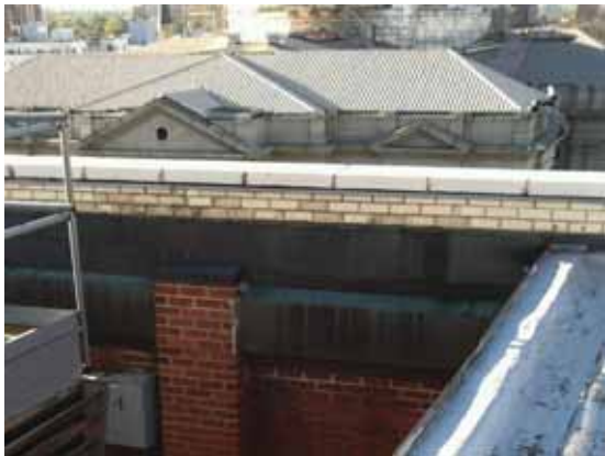
Fig. 2.1.A.10 Deteriorating and spalling brick observed along the west side of the Penthouse roof.
