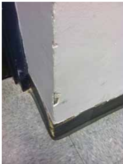
Fig. 3.0.C.5 Damaged gypsum board and vinyl baseboard observed on the Sub-basement Floor.
