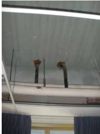
Fig. 2.4.A.18 – Pipes serving upper floor convectors
