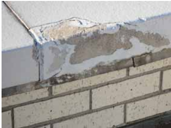
Fig. 2.1.A.15 Sealant deteriorating, or missing entirely, from the joints between the masonry blocks along the top edge of the Penthouse roof parapet, is likely resulting in damage to the coating on the blocks.
