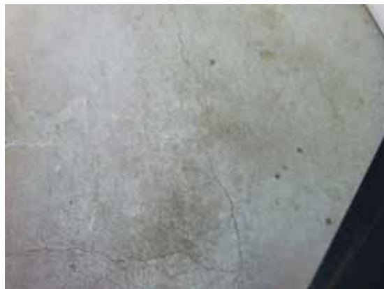
Fig. 3.0.C.21 Cracked concrete flooring observed on the Sub-basement Floor.
