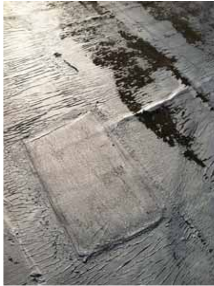
Fig. 2.1.A.25 Typical overall deterioration of the roofing membrane, including at membrane patches.
