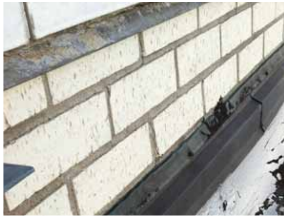
Fig. 2.1.A.11 Areas of cracking mortar noted along the brick joints around the roof and Penthouse roof parapets.
