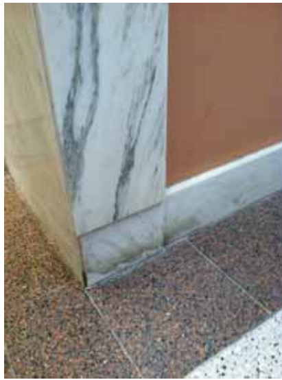
Fig. 3.0.C.7 Areas of soiled marble cladding on the walls noted in the elevator lobbies throughout.
