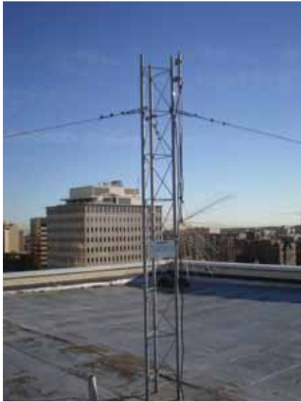
Fig. 2.4.A.9 – Broken lightning protection
