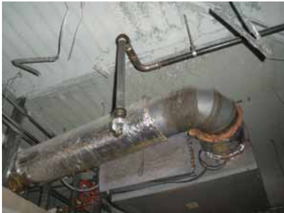
Fig. 2.4.A.16– Pro-press fitting used for sprinkler piping
