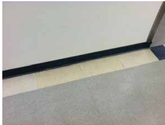
Fig. 3.0.C.16 Discolored 1x1 linoleum tile flooring noted during the site survey visit.
