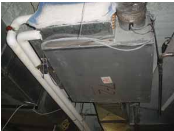
Fig. 2.4.A.17 – VAV filters are clogged
