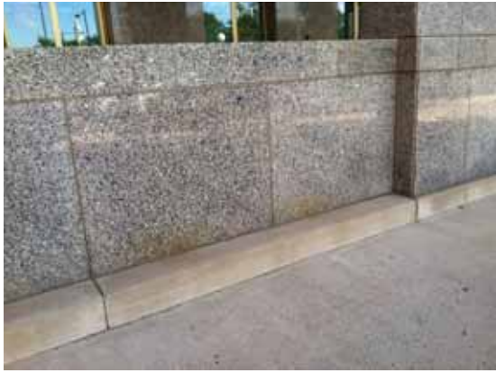
Fig. 2.1.A.2 Soiled granite panels noted around the base of the building, especially on the west side.
