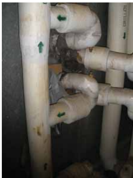
Fig. 2.4.A.11 – Air leakage from opening around pipes
