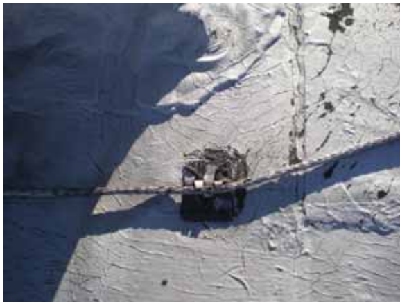
Fig. 2.4.A.10 – Lightning protection wire on roof
