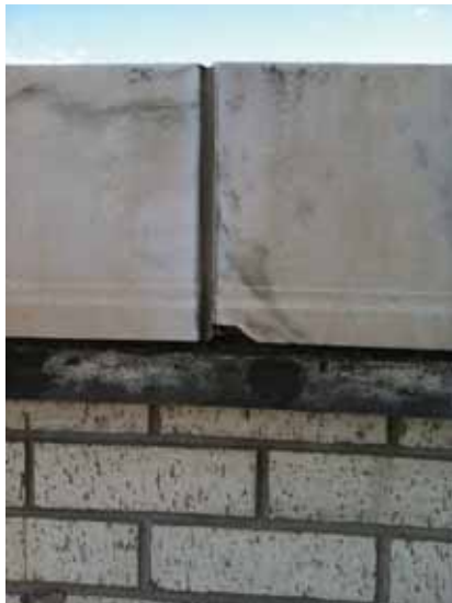
Fig. 2.1.A.16 Damaged marble blocks noted in a few spots around the top edge of the roof parapet.
