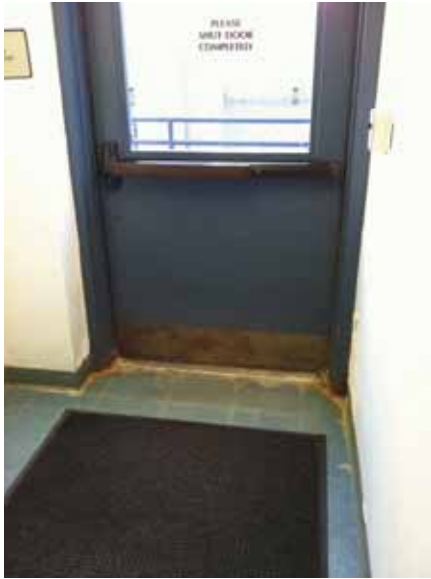
Fig. 3.0.C.18 Water damage noted at the 1x1 floor tile near the emergency exit at the west end of the north side of the Ground Floor.
