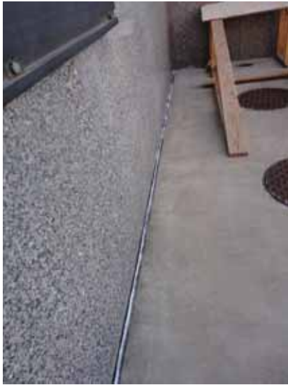
Fig. 2.1.A.8 Sealant deteriorating and missing along the base of the building, allowing water penetration.
