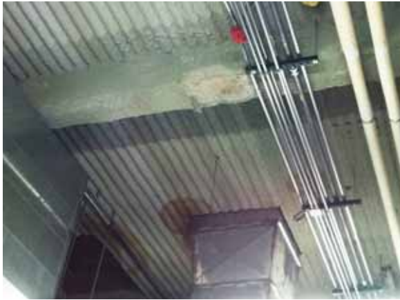
Fig. 2.1.A.22 Evidence of water intrusion at the Penthouse ceiling.
