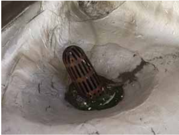
Fig. 2.1.A.28 Drain cover with signs of corrosion and with moss growing near the base.
