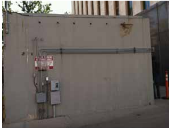
Fig. 2.1.A.39 Spalling and cracking noted at the west wall of the one-story concrete structure along the north side of the building.
