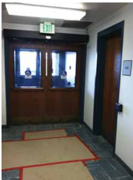
Fig. 2.1.A.18 Interior doors at the accessible entrance vestibule on the south end of the west side of the building have an air gap between the door slabs.
