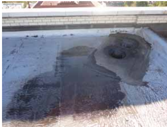
Fig. 2.1.A.26 Ponding observed in several spots near the roof drains.
