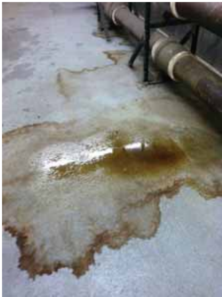
Fig. 2.1.A.23 Water observed on the floor of the Penthouse.
