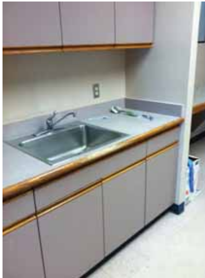
Fig. 3.0.C.27 Generally worn wood trim noted in the Break Rooms throughout.
