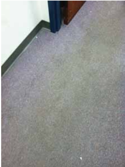
Fig. 3.0.C.13 Deteriorating and soiled carpet noted throughout the Sub-basement Floor.
