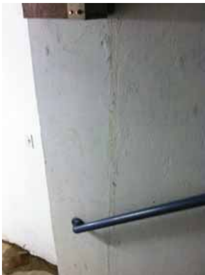
Fig. 3.0.C.11 Water damage noted at the walls near the emergency exit on the Sub-basement Floor.
