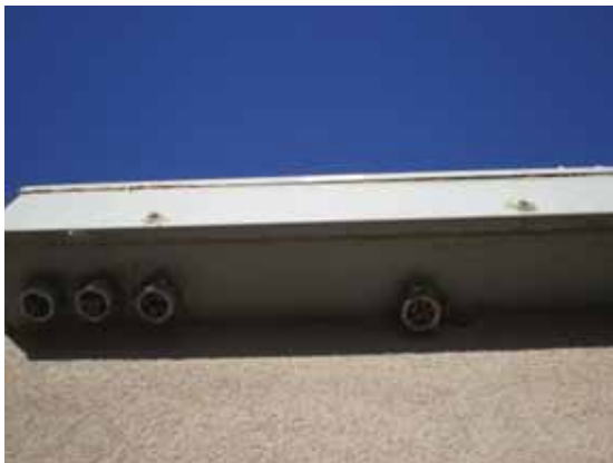
Fig 2.4.B.1 – Openings in the wireway
