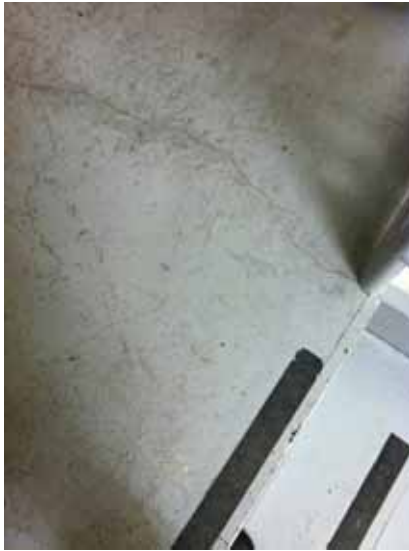
Fig. 3.0.C.35 Cracking noted throughout the north exit stairway.
