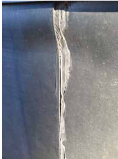
Fig. 2.1.A.16 Deteriorating sealant along the seams of the roofing membrane covering the inside face of the parapet.
