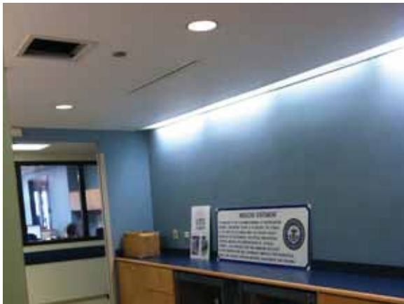
Fig. 3.0.C.2 Cover missing from a ceiling access hatch in the elevator lobby on the Fourth Floor.
