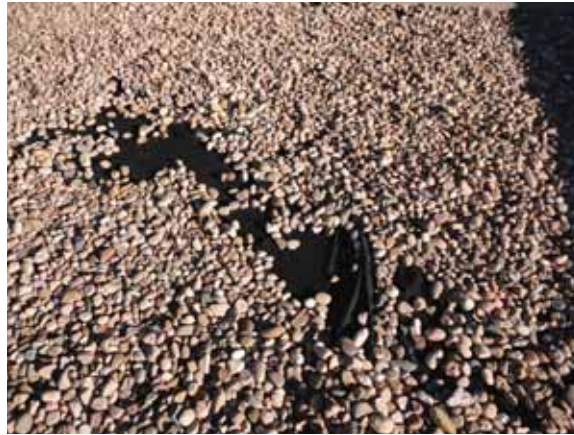
Fig. 2.1.A.10 Typical areas of thin ballast exposing the roof membrane.
