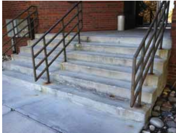
Fig. 2.1.A.26 Spalling and cracking concrete and corroding railings at the North Entrance.
