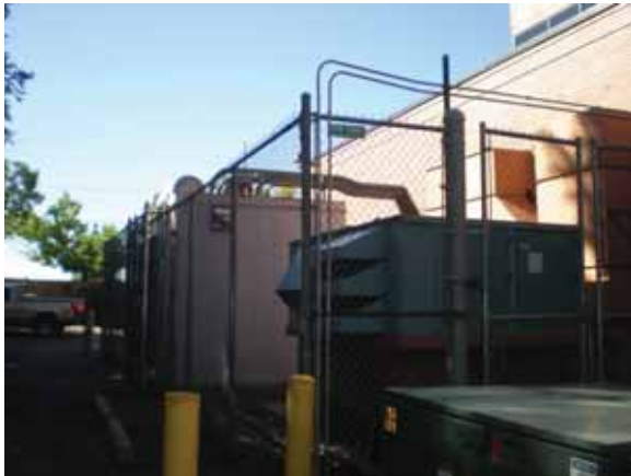
Fig 2.4.A.9 – Generator in back of the building
