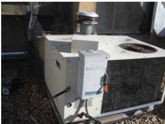
Fig 2.4.A.13 – RTU serving gun room
