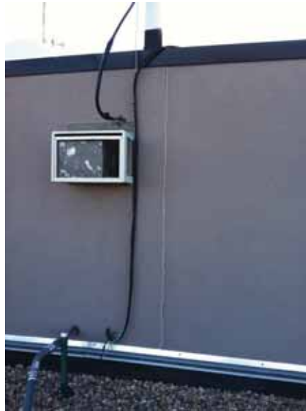
Fig. 2.1.A.5 Stucco panels cladding the Penthouse with expanding space between the panels.
