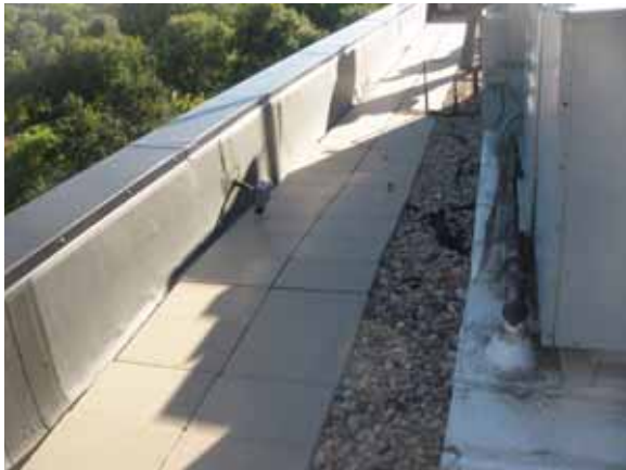
Fig 2.4.A.12 – No railing provided for fall protection
