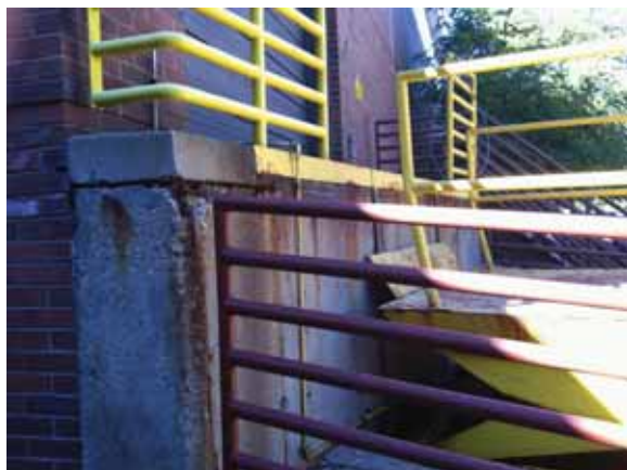
Fig. 2.1.A.25 Spalling concrete and corroding metal at the north loading dock.
