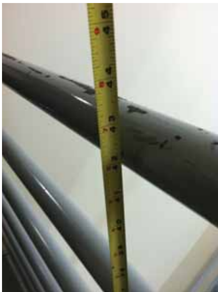
Fig. 2.1.B.9 The spacing between the railings exceeds the code-maximum of four inches.
