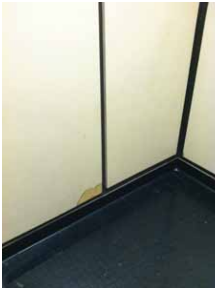
Fig. 2.1.D.1 Typical instance of damage to the panels cladding the interior walls of the elevator cabs.
