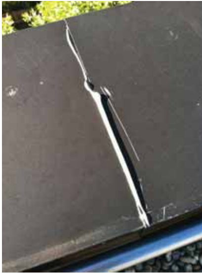
Fig. 2.1.A.19 Poor sealant repair along the seams of the parapet's coping.
