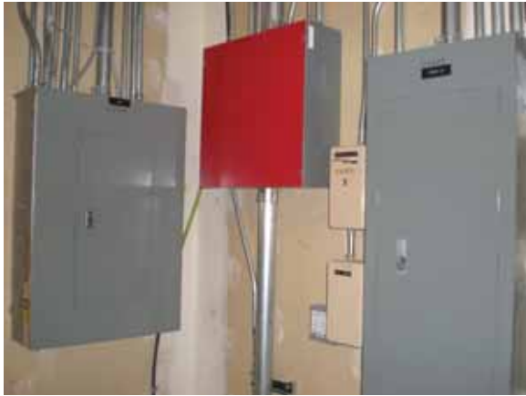
Fig 2.4.A.2 – Electrical room panelboards
