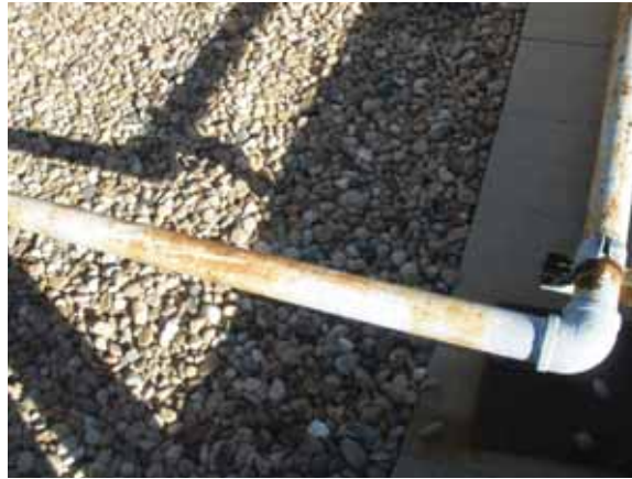
Fig 2.4.A.14 – Rusted gas piping on roof
