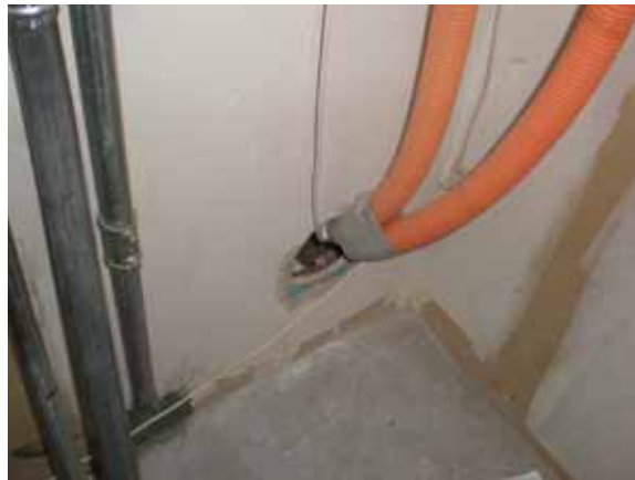
Fig 2.4.B.4 – Wall penetrations not sealed
