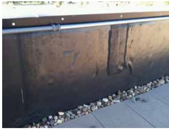
Fig. 2.1.A.17 Deteriorating sealant along the seams of the roofing membrane and bubbling of the roofing membrane covering the inside face of the parapet.
