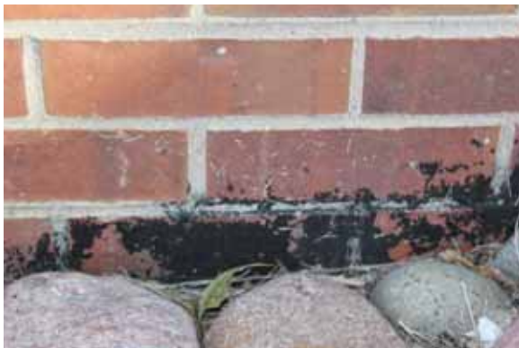
Figure 2.3.B.2 – Black Mold-Like Substance on Side of Building
