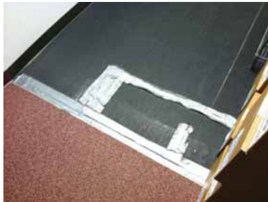
Fig. 3.0.C.28 Tape on the surface of the ramp leading up to the server and technology rooms located on the northeast side of the Third Floor is creating a tripping hazard.
