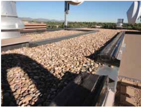
Fig. 2.1.A.20 Evidence of water pooling along the Penthouse parapet's coping.
