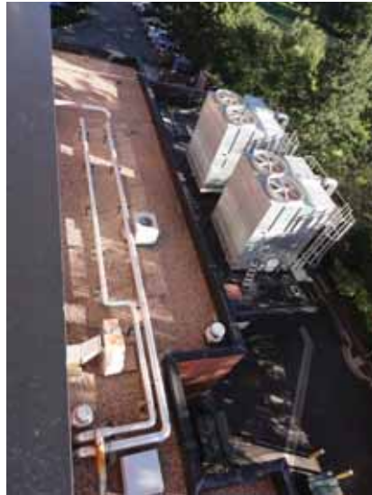
Fig. 2.1.A.22 View of the roof above the two-story section of the building along the east side.
