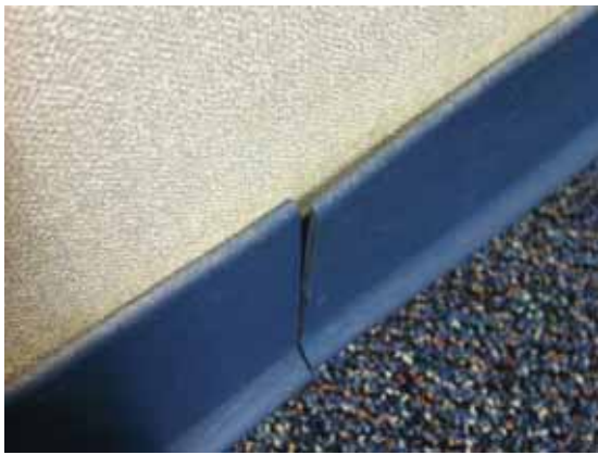
Fig. 3.0.C.16 Vinyl baseboard pulling away from the wall in spots throughout the Second and Third Floor corridors.
