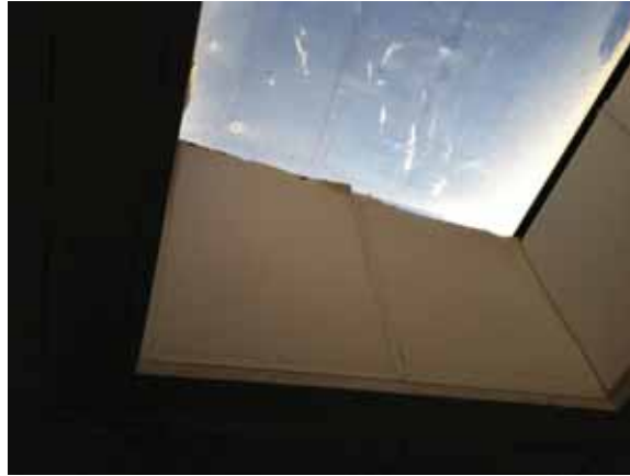
Fig. 2.1.A.11 Water damage noted at the skylight.
