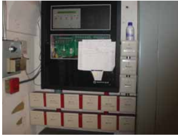
Fig 2.4.A.8 – Fire alarm control panel
