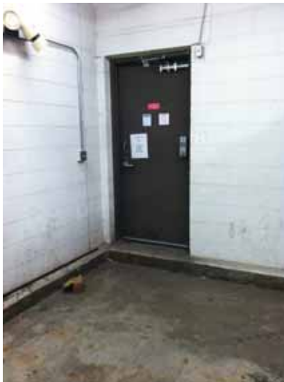
Fig. 3.0.C.26 Evidence of water damage noted at the concrete floor in the battery storage room at the southeast corner of the First Floor.
