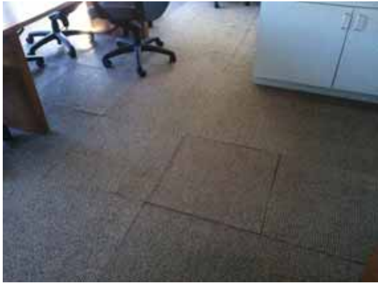
Fig. 3.0.C.24 Carpet flooring pulling loose along the seams and creating a potential tripping hazard.
