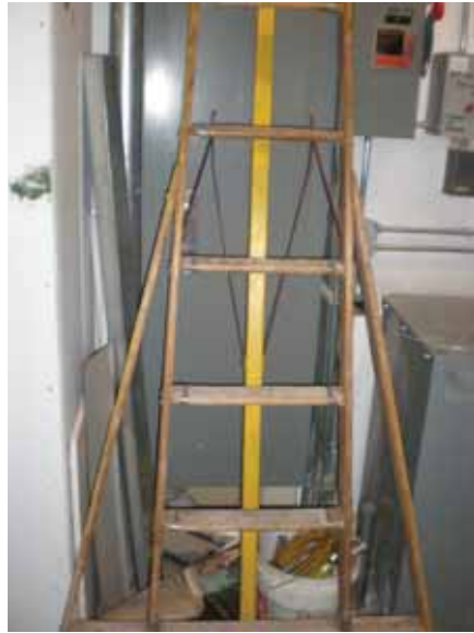
Fig 2.4.B.3 – Ladder in front of the panel board
