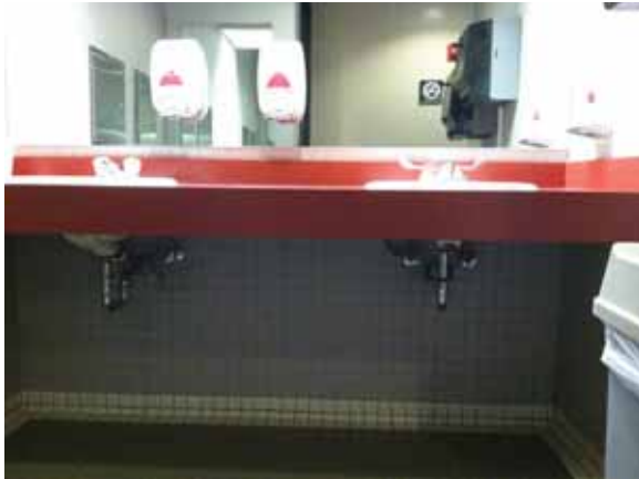
Fig. 2.1.C.2 Accessible lavatory without insulation wrapped around the pipes.
