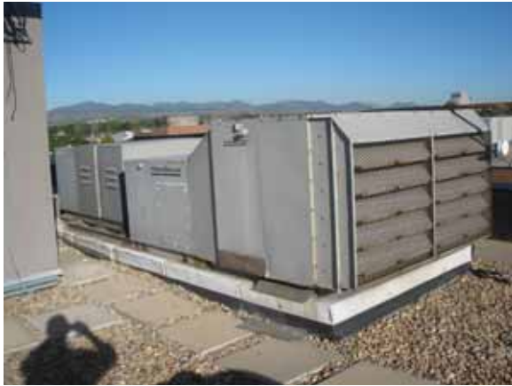
Fig 2.4.A.11 – Unit serving labs on fourth floor
