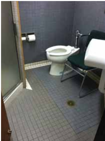
Fig. 3.0.C.32 Area of newer-looking tile noted on the floor in the First Floor Unisex Shower Room.
