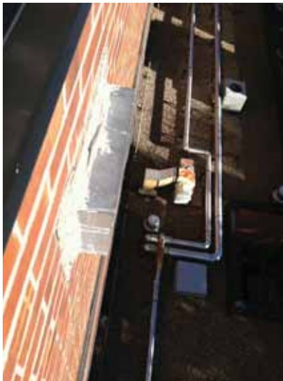
Fig. 2.1.A.21 Deteriorating sealant which has been poorly repaired at the through-parapet drains.
