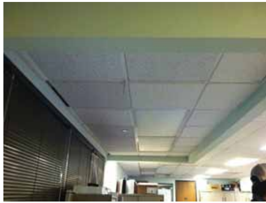
Fig. 3.0.C.4 Deteriorating and sagging 2x2 acoustic ceiling.
