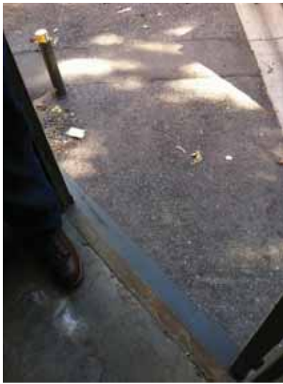
Fig. 2.1.B.6 Interior view looking out of the emergency exit near the center of the east side of the building with no direct access to grade per code requirements.
