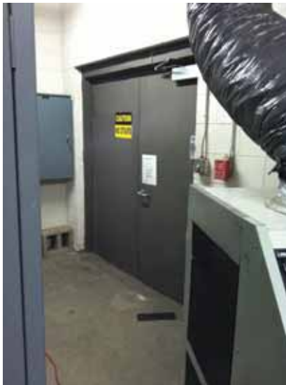
Fig. 2.1.B.7 Warning sign at interior side of emergency exit near the center of the east side of the building does not provide exemption from code requirements for direct access to grade.
