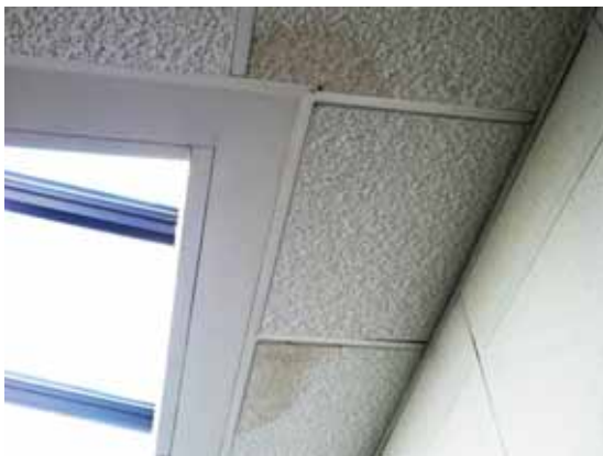
Fig. 3.0.C.8 Water damage noted to the 2x2 acoustic ceiling tiles around the skylight at the Penthouse level.
