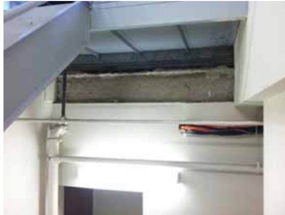
Fig. 3.0.C.38 Area of exposed floor structure under a landing in the north exit stairway.
