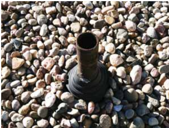
Fig. 2.1.A.14 Corroding roof exhaust vent.
