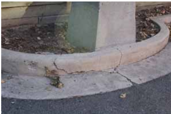
Figure 2.3.A.7 – Broken Site Concrete, Recommended for Replacement
