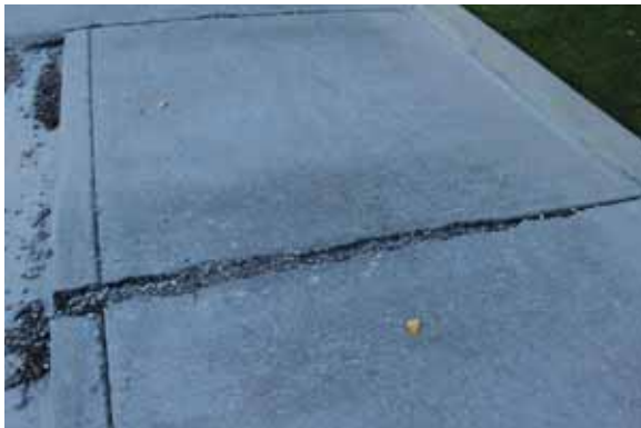
Figure 2.3.A.6 – Broken Site Concrete, Recommended for Replacement
