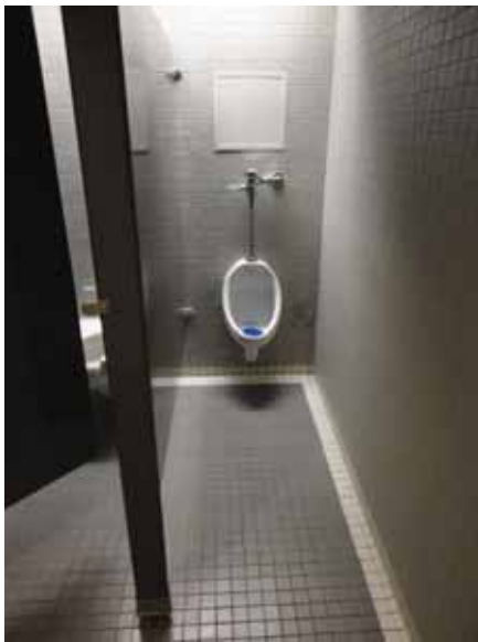
Fig. 2.1.C.3 Fourth Floor urinal alcove is too narrow per accessibility standards.
