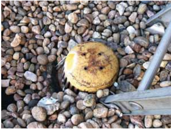
Fig. 2.1.A.13 Corroding roof drain cover.
