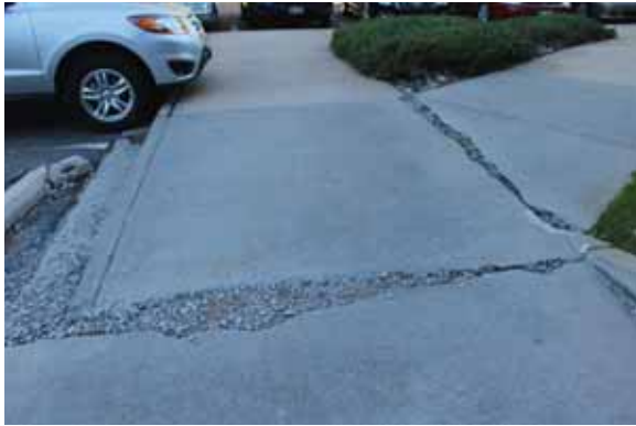
Figure 2.3.A.5 – Broken Site Concrete, Recommended for Replacement
