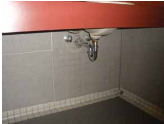
Fig 2.4.A.21 – Under sink piping insulation cover not provided
