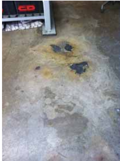
Fig. 3.0.C.27 Corrosion noted at the concrete floor in the middle of the battery storage room at the southeast corner of the First Floor.
