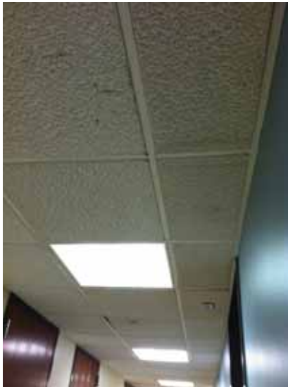
Fig. 3.0.C.7 General sagging and deterioration of the 2x2 acoustic ceiling tiles on the Fourth Floor.
