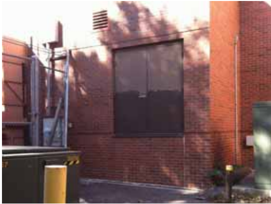
Fig. 2.1.B.5 Exterior view of the emergency exit near the center of the east side of the building with no direct access to grade per code requirements.
