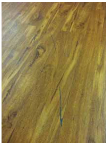
Fig. 3.0.C.20 Scuff marks noted to the vinyl flooring in the entrance and elevator lobbies on the First Floor.
