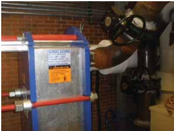
Fig 2.4.A.19 – Flat plate heat exchanger
