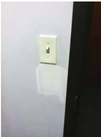
Fig. 3.0.C.17 An area of the gypsum board wall that was repaired but left unfinished in the First Floor Unisex Shower Room.
