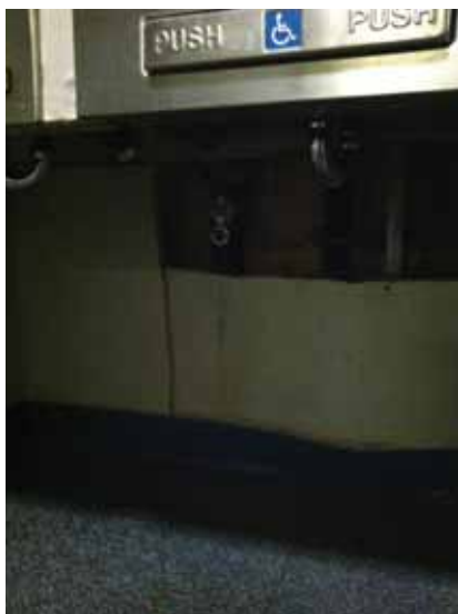
Fig. 3.0.C.12 Area of missing gypsum board and damaged gypsum board and vinyl baseboard located underneath the drinking fountains on the Third Floor.
