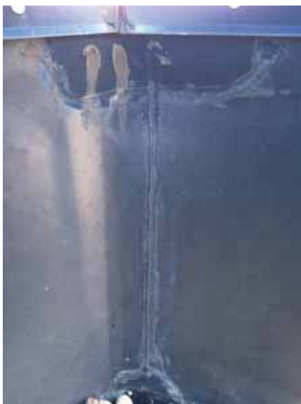
Fig. 2.1.A.15 Deteriorating sealant along the seams of the roofing membrane covering the inside face of the parapet.
