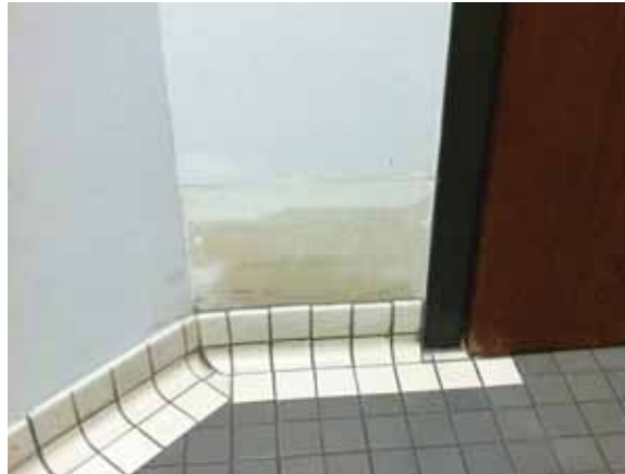
Fig. 3.0.C.18 Damaged gypsum board noted in the First Floor Women's Restroom.
