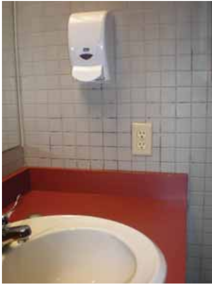
Fig 2.4.B.6 – No GFI receptacle by sink
