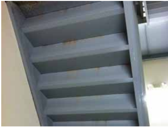
Fig. 3.0.C.36 Corrosion noted at the bottom side of the north exit stairway with roof access.
