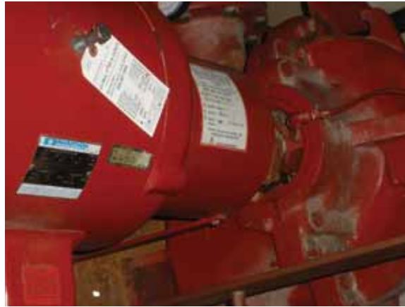
Fig 2.4.A.20 – Fire Pump Room
