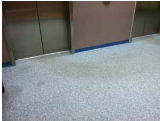
Fig. 3.0.C.21 Areas of worn and soiled carpet in the Second and Third Floor elevator lobbies.
