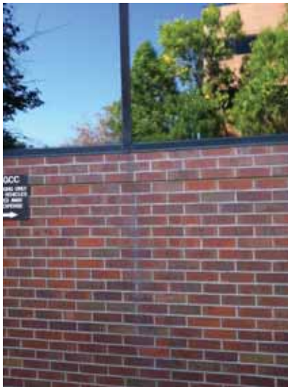
Fig. 2.1.A.3 Soiling of the brick observed under the continuous ribbon windows.
