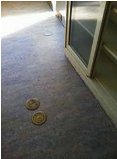
Fig. 3.0.C.31 Raised floor-mounted receptacles noted throughout the Fourth Floor Break Room.
