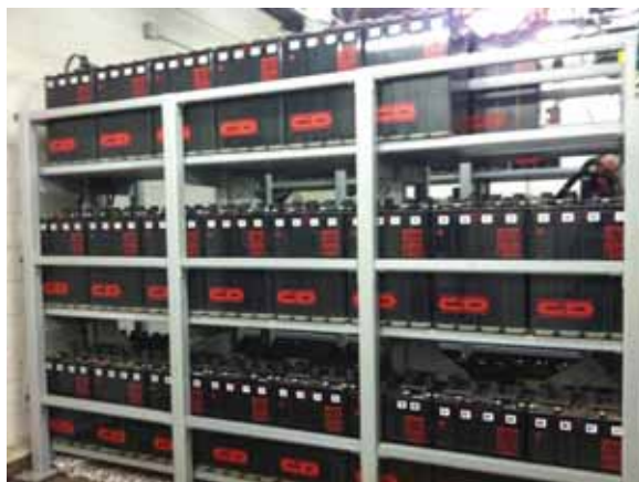
Fig. 2.1.B.1 Battery storage room.
