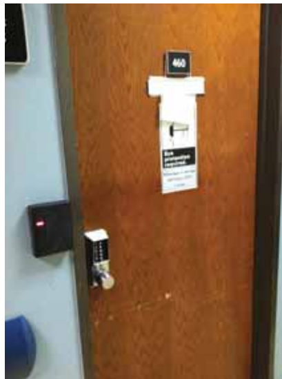
Fig. 3.0.C.33 General wear-and-tear noted at the doors throughout the building.
