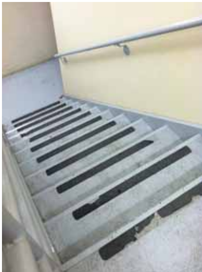
Fig. 3.0.C.37 General soiling and wear-and-tear noted throughout the north exit stairway.
