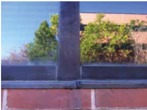
Fig. 2.1.A.7 Typical corrosion noted at the metal window frames.
