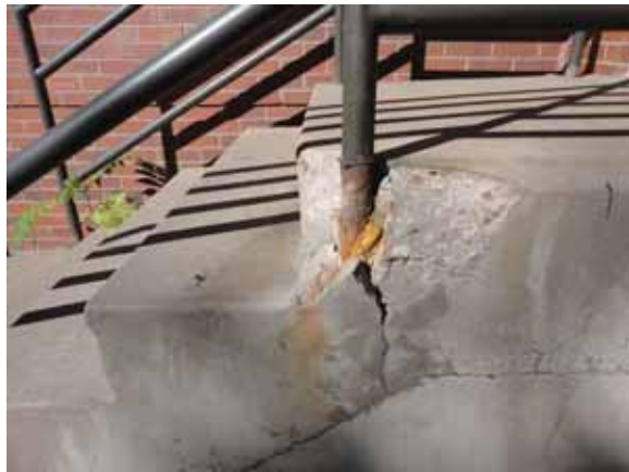
Fig. 2.1.A.24 Spalling concrete at the exterior southeast stairway.
