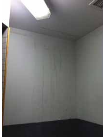
Fig. 3.0.C.3 Evidence of water damage to the ceiling and walls in the Unisex Shower Room on the First Floor.
