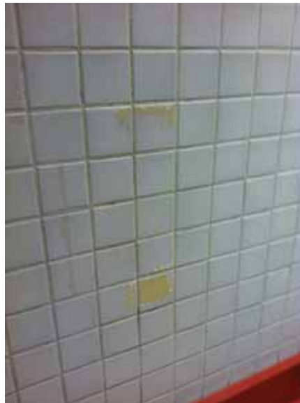
Fig. 3.0.C.19 Residue noted on the 2-inch square wall tiles in the First Floor Women's Restroom.
