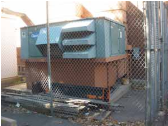
Fig 2.4.A.18 – Backup unit serving electrical room
