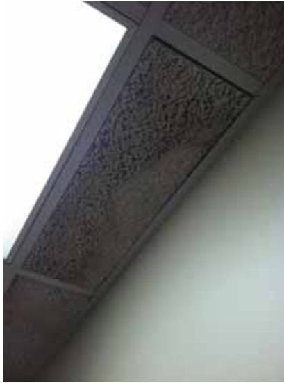
Fig. 3.0.C.6 Typical instance of water damage noted at the 2x2 acoustic ceiling on the Fourth Floor.
