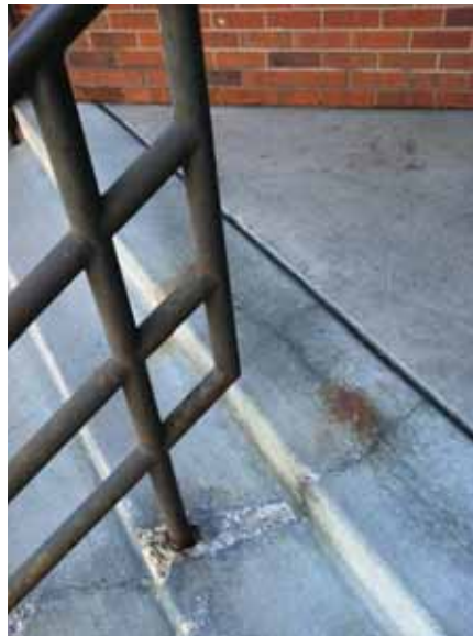
Fig. 2.1.A.27 Spalling and cracking concrete and corroding railings at the North Entrance.
