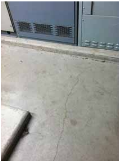
Fig. 3.0.C.25 Typical cracking noted in the concrete in the equipment rooms on the east side of the First Floor.
