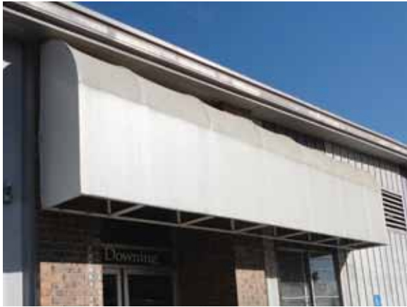
Fig. 2.1.A.24 Generally soiled canopy with a corroding metal frame observed at the entrance on the south side of the building.
