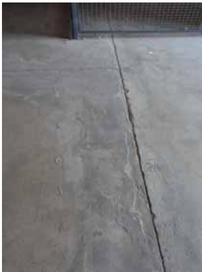
Fig. 3.0.C.7 Deterioration and spalling of the concrete flooring observed throughout the building.
