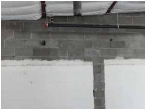
Fig. 3.0.C.2 Holes observed in the masonry block wall separating the building in half.
