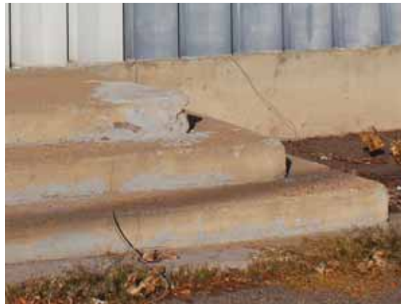
Fig. 2.1.A.25 Typical instance of deteriorating paint and spalling and cracking concrete observed at the exterior stairways and ramps on the north and east sides of the building.
