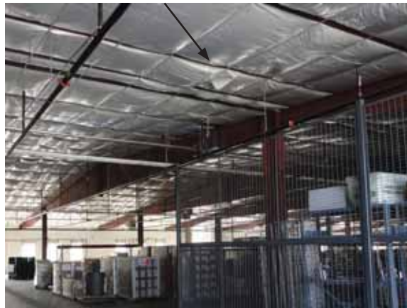
Fig. 3.0.C.1 Insulation observed hanging loose during the site survey visit..
