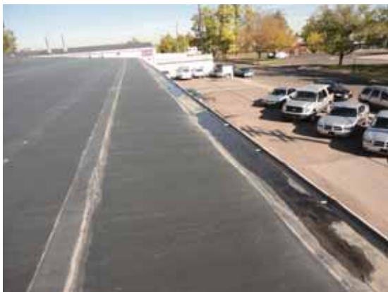
Fig. 2.1.A.22 Areas of standing water observed during the site survey visit.
