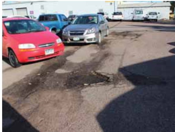
Figure 2.3.B.3 – Broken, Depressed Asphalt
