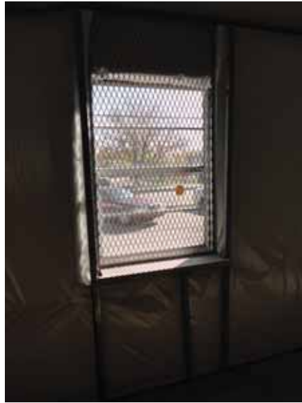
Fig. 2.1.B.21 Typical instance of a metal security grille observed at the windows around the exterior of the building.
