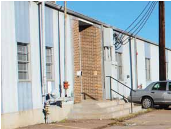
Fig. 2.1.B.11 A stairway on the east side of the building that is not equipped with handrails on both sides as required by code and with spalling and cracking concrete creating a potential tripping hazard.
