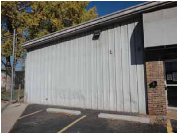
Fig. 2.1.A.3 Damaged metal panels observed along parking areas around the exterior of the building.
