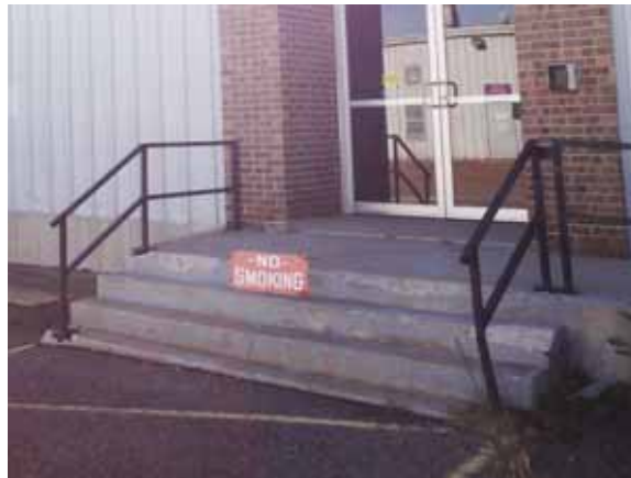
Fig. 2.1.A.26 Spalling and cracking of the concrete stairway and corroding and damaged metal railings observed at the entrance on the west end of the north side of the building.
