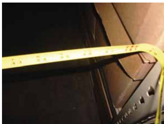
Fig. 2.1.B.5 Aisles generally observed to be 36 inches or greater in the areas included in the site survey visit.
