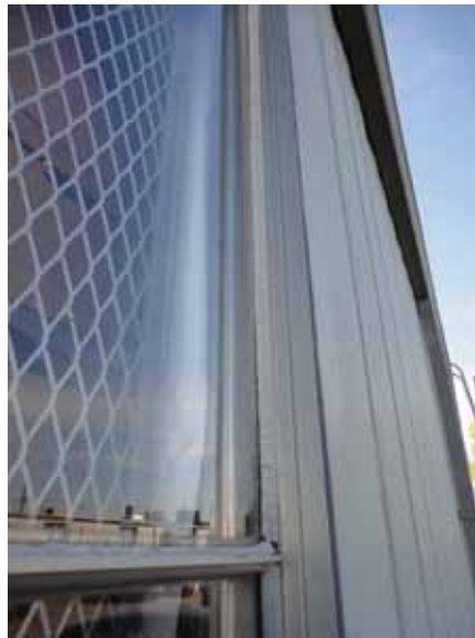
Fig. 2.1.A.10 Typical instance of deteriorating sealant observed at the windows around the exterior of the building.
