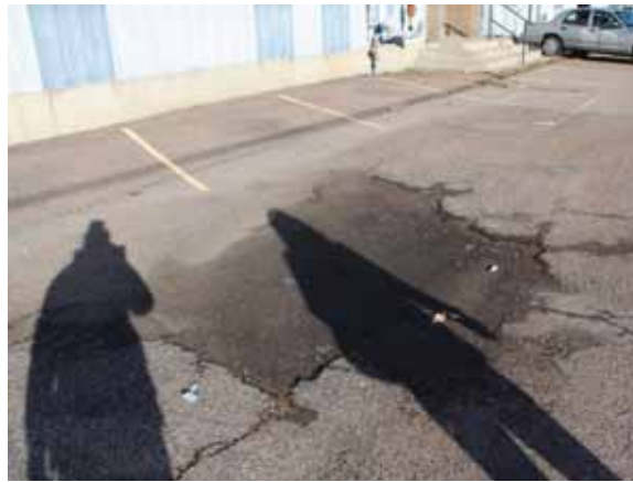
Figure 2.3.B.2 – Broken Asphalt at a location of depressed grade
