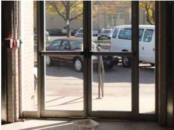
Fig. 2.1.A.11 Deterioration of the weatherstripping along the base of a door noted to be creating an air gap.
