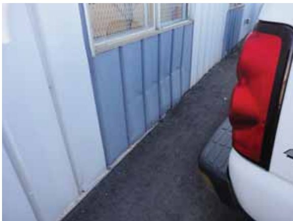
Fig. 2.1.A.4 Damaged metal panels observed along parking areas around the exterior of the building.
