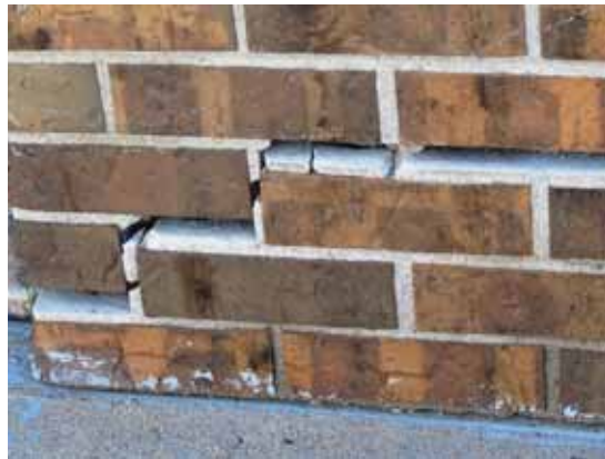
Fig. 2.1.A.6 Cracking and deterioration of a brick infill wall noted on the north side of the building.
