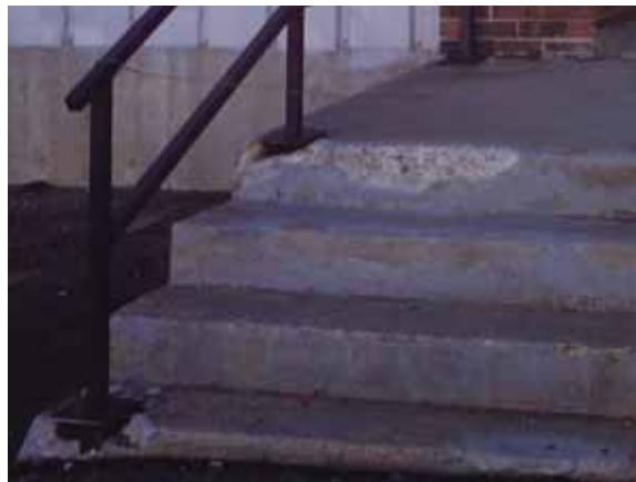
Fig. 2.1.B.13 Spalling and cracking concrete at railing posts observed at an exterior stairway on the north side of the building.
