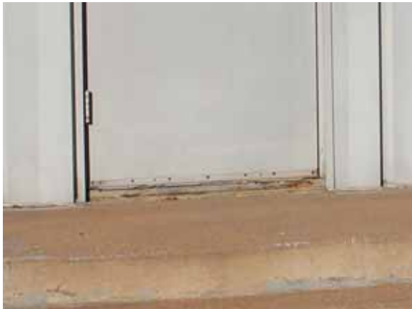
Fig. 2.1.A.12 Deterioration of the weatherstripping and corrosion of the metal observed at the base of an exterior door on the east side of the building.
