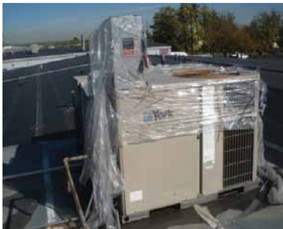
Fig. 2.4.A.6 – Decommissioned rooftop unit
