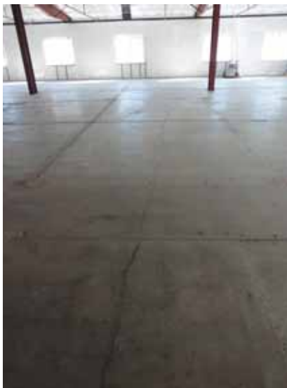
Fig. 3.0.C.8 Cracking areas of the concrete flooring observed throughout the building.
