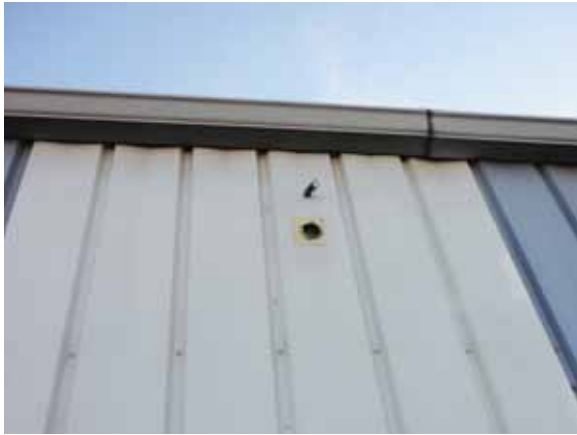
Fig. 2.1.A.2 Unrepaired holes leaving the building envelope vulnerable to water penetration observed in areas around the exterior of the building.
