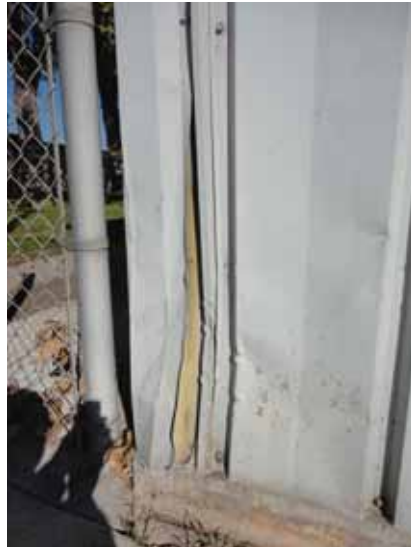
Fig. 2.1.A.5 Extensive damage to the metal panels noted during the site survey visit.
