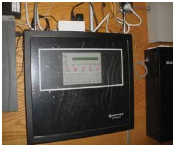
Fig. 2.4.A.5 – Fire alarm control panel
