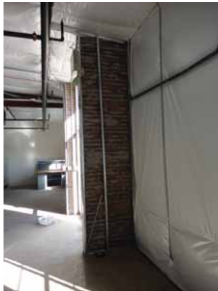
Fig. 3.0.C.5 Areas of unfinished walls observed during the site survey visit.
