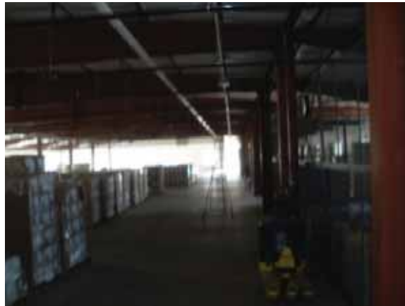
Fig. 2.4.A.4 – Linear fluorescent luminaires
