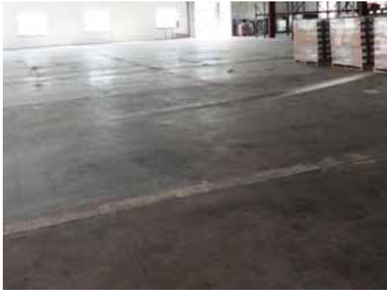
Fig. 3.0.C.6 General deterioration of the concrete flooring observed during the site survey visit.
