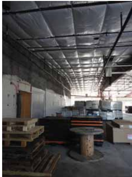
Fig. 2.1.B.4 Wood pallets, stacks of flat cardboard boxes, and other items being stored on the south side of the building.
