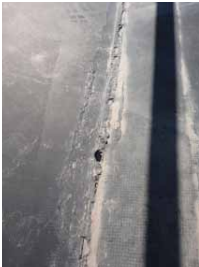
Fig. 2.1.A.16 Typical instance of deteriorating sealant along the seams of the rubber roofing membrane.
