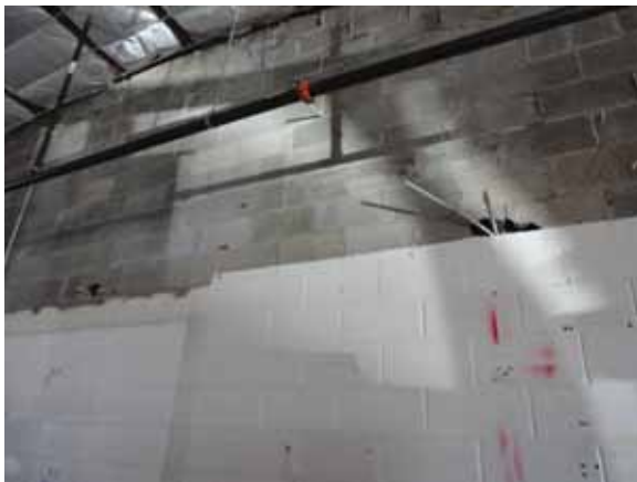
Fig. 3.0.C.3 Pieces of pipes or tubes sticking out of a few of the holes observed in the masonry block wall separating the building in half.
