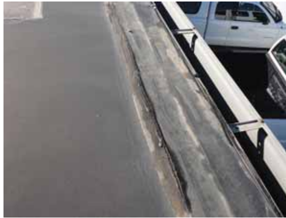
Fig. 2.1.A.17 Typical instance of sealant missing entirely along the seams of the rubber membrane and exposing the roof system to water penetration.
