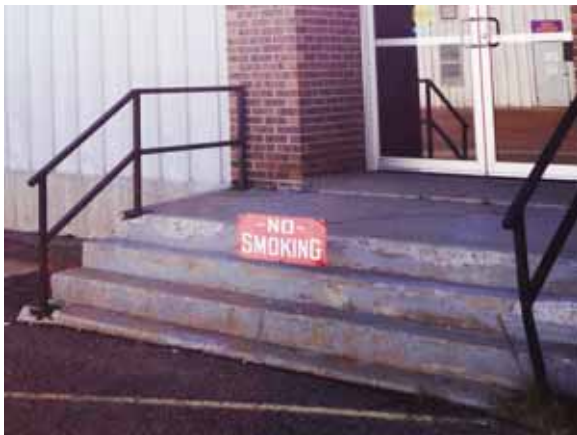
Fig. 2.1.B.8 A “No Smoking” sign strung with wire between the stairway railings and blocking the means of egress from the entrance on the west end of the north side of the building.
