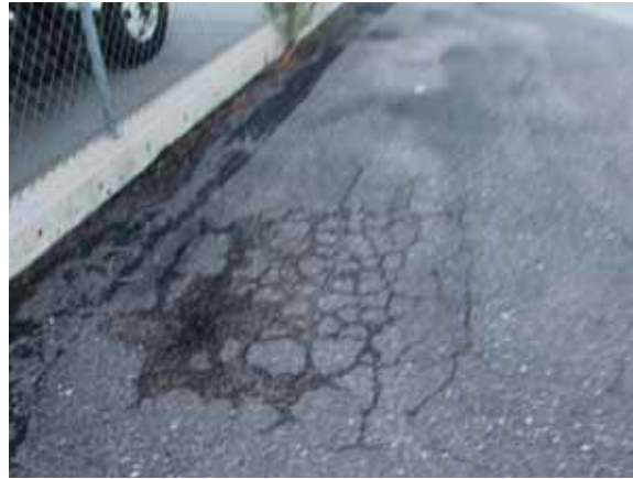
Figure 2.3.A.6 – Poor Site Asphalt Condition
