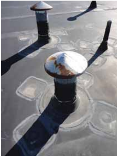
Fig. 2.1.A.20 Evidence of corrosion noted at a roof vent cover.
