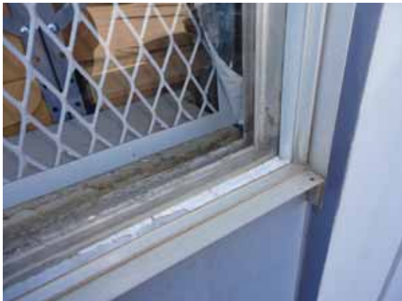
Fig. 2.1.A.8 Evidence of deterioration and water intrusion noted at the windows around the exterior of the building.
