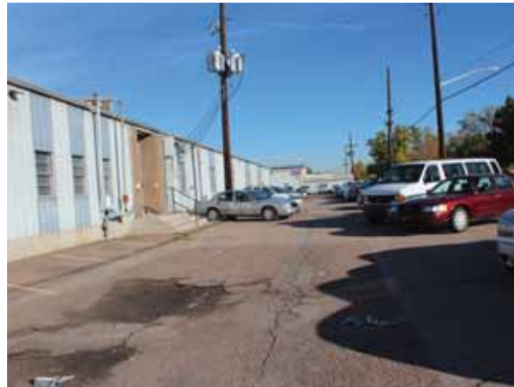
Figure 2.3.A.7 – Poor Site Asphalt Condition
