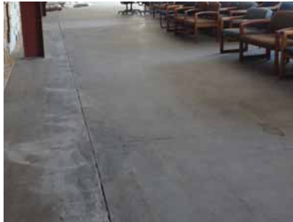
Fig. 3.0.C.9 An area of potential water damage observed at the concrete flooring on the north side of the building.
