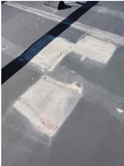
Fig. 2.1.A.15 Typical instance of deteriorating sealant at patched areas of the rubber roofing membrane.
