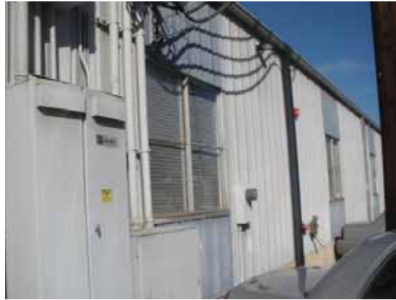
Fig. 2.4.A.3 – Electrical Service Entrance
