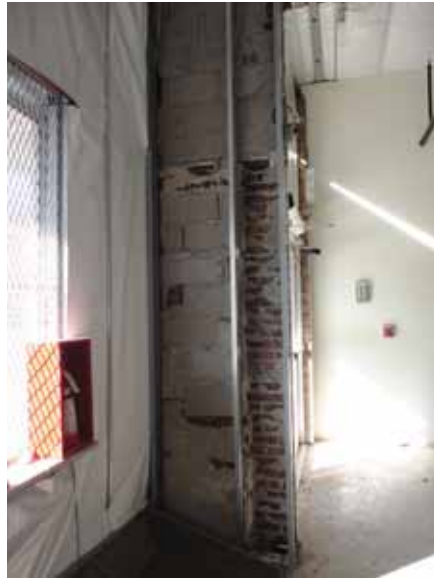
Fig. 3.0.C.4 Areas of unfinished walls observed during the site survey visit.
