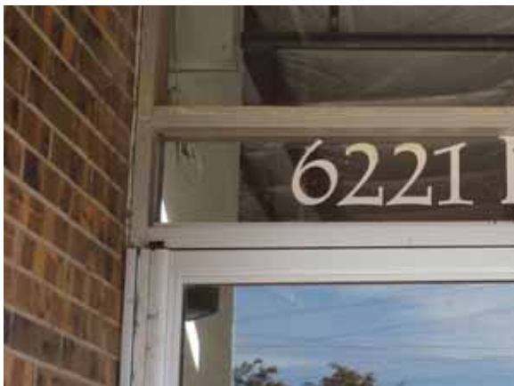
Fig. 2.1.A.13 General deterioration of the sealant noted at the doors around the exterior of the building.
