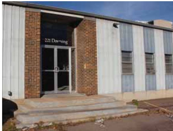
Fig. 2.1.B.12 A stairway on the east side of the building that is not equipped with handrails as required by code and with spalling and cracking concrete creating a potential tripping hazard.
