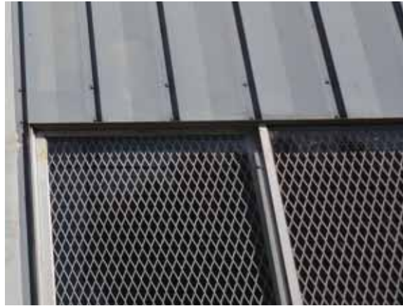
Fig. 2.1.A.9 Evidence of corrosion noted at the window frames around the exterior of the building.
