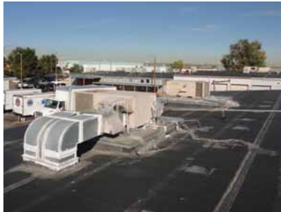
Fig. 2.1.A.18 Thin plastic sheeting wrapped around the rooftop equipment noted to be deteriorating.
