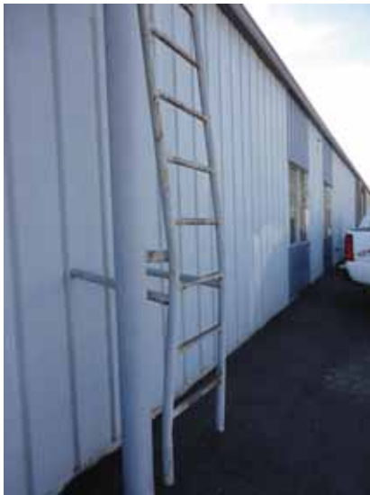
Fig. 2.1.A.21 Evidence of corrosion noted at the ladder leading up to the roof on the west side of the building.
