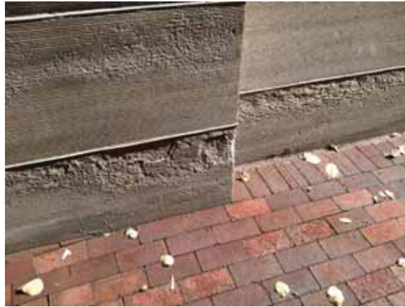
Fig. 2.1.A.4 Spalling of the foundation blocks.
