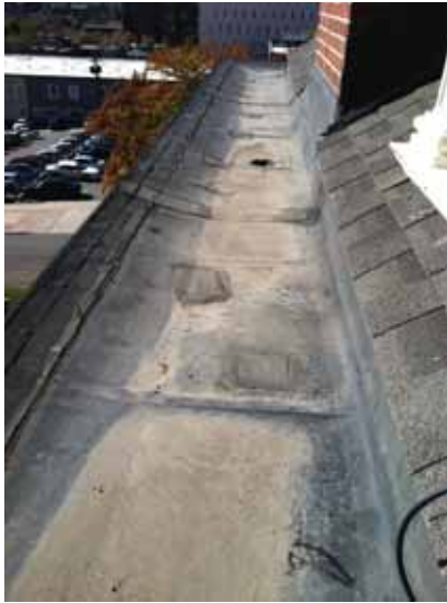
Fig. 2.1.A.39 Leaves and debris collecting at the roof over the front porch on the north side of the building.
