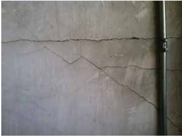
Fig. 3.0.C.6 Widespread areas of water damage, cracking, and spalling observed at the walls throughout the attic storage space on the Third Floor.
