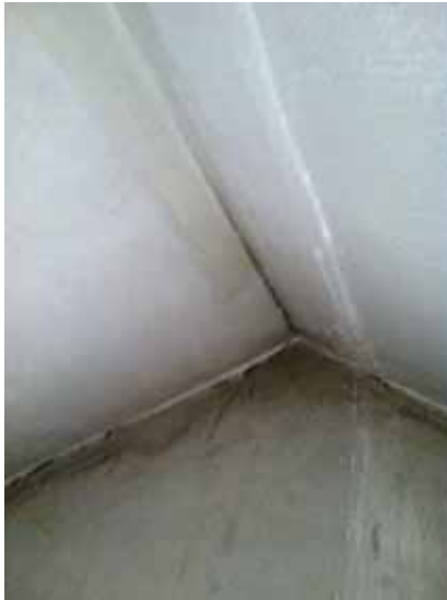
Fig. 2.1.A.33 Evidence of widespread water intrusion and damage noted throughout the attic.
