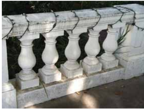
Fig. 2.1.A.61 Soiling noted at the railings along the curved white retaining wall.
