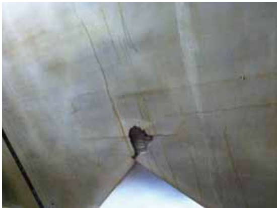
Fig. 2.1.A.34 Evidence of widespread water intrusion and damage noted throughout the attic.
