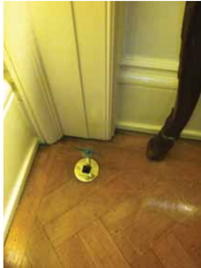
Fig. 3.0.C.17 A metal valve, or control, noted to be projecting above the floor of the Family Game Room/Bar in the northeast corner of the First Floor and creating a potential tripping hazard.
