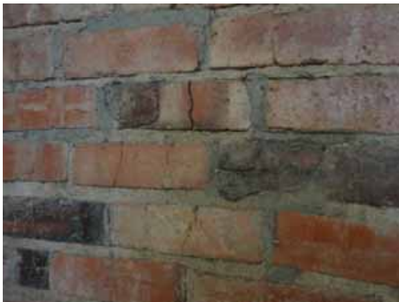
Fig. 3.0.C.13 Deterioration and cracking noted at the brick wall in the southeast stairway at the Basement Floor.
