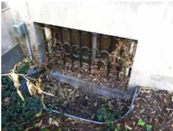
Fig. 2.1.A.28 Debris observed in a few of the window wells around the building.
