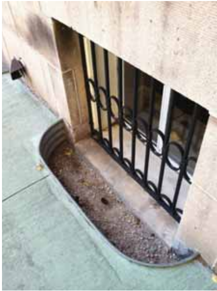
Fig. 2.1.A.27 Window well on the east side of the building observed to have evidence of water saturation.
