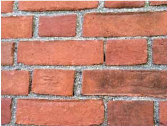
Fig. 2.1.A.1 Areas of deteriorating or missing mortar noted in a few areas of the brick walls around the exterior of the building.
