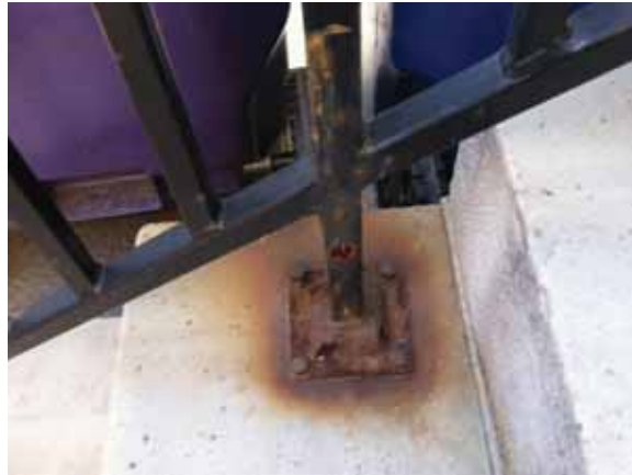
Fig. 2.1.B.5 Corroding railing posts at the exterior stairway of the southeast service entrance.
