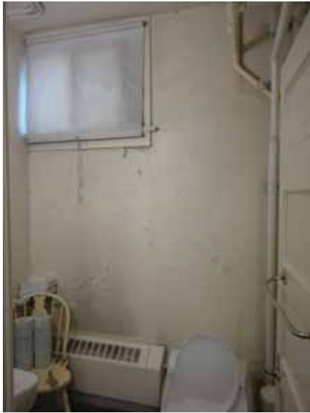
Fig. 3.0.C.12 Damage observed at the east wall of the window in the restroom located north of the Laundry Room on the Basement Floor.
