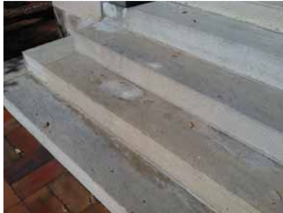
Fig. 2.1.A.54 Areas of spalling and damage observed at the exterior stairways around the building.
