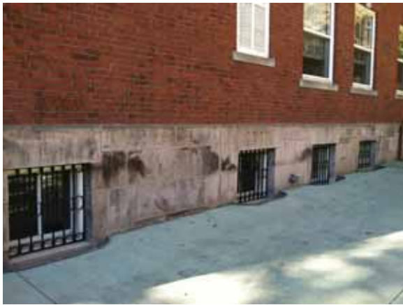
Fig. 2.1.A.2 Areas of widespread soiling of the foundation noted around the exterior of the building.
