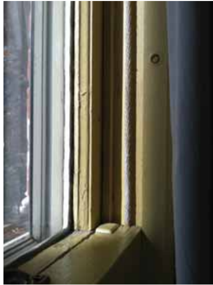
Fig. 2.1.A.24 Damage noted on the interior side of a few of the First through Third Floor windows.
