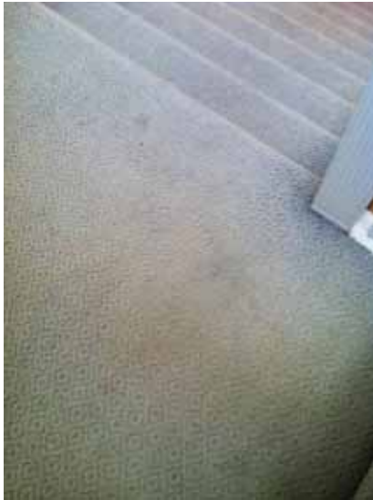
Fig. 3.0.C.26 Typical instance of soiled and worn carpet observed on the Grand Stairway.
