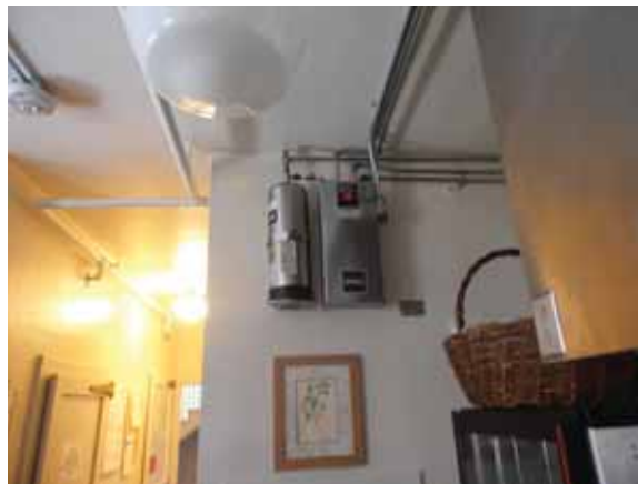
Fig. 2.4.A.21 – Fire suppression for kitchen hood
