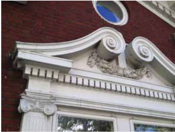
Fig. 2.1.A.13 Generally soiled decorative trim with cracking and peeling paint.
