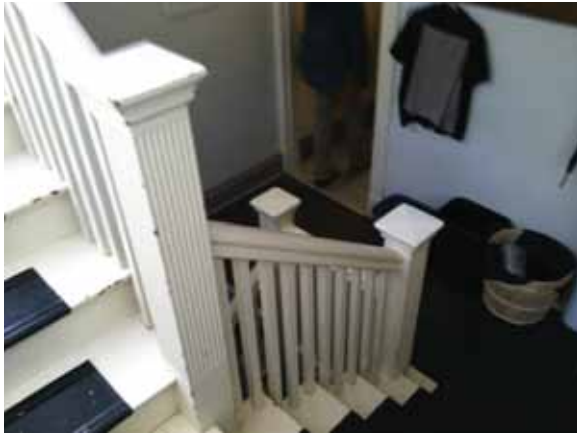
Fig. 3.0.C.32 Areas of worn pain noted throughout the southeast stairway.
