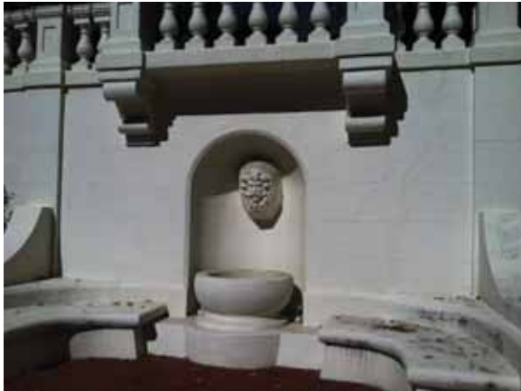
Fig. 2.1.A.57 Widespread cracking observed at the curved white retaining wall and soiling of the seating and flat surfaces.
