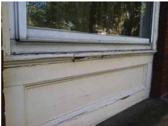
Fig. 2.1.A.15 Widespread peeling and cracking paint noted at the wood trim around the exterior of the building.
