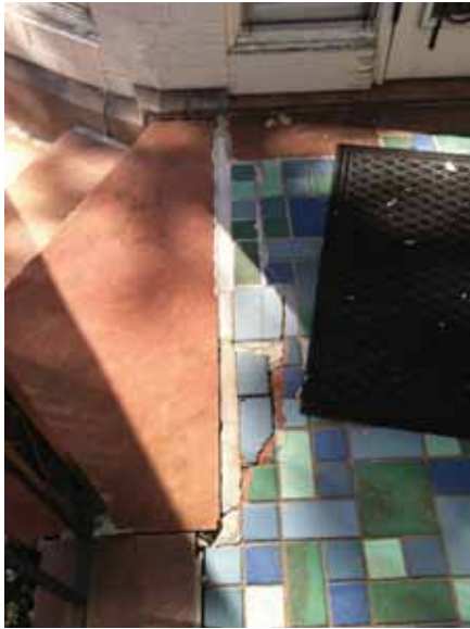
Fig. 2.1.A.51 An area of damaged tile pavers creating a potential tripping hazard noted at the patio on the southeast side of the First Floor Palm Room.
