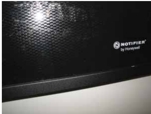
Fig. 2.4.A.13 – Fire alarm system
