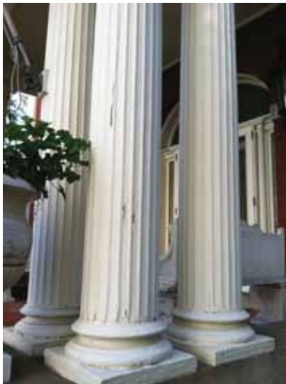
Fig. 2.1.A.21 Cracking and peeling paint observed at the columns.
