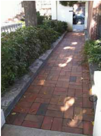
Fig. 2.1.A.46 Deterioration and spalling noted at areas of the concrete edging.
