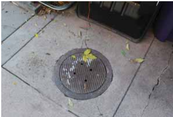
Figure 2.3.A.5 – Site Concrete Crack
