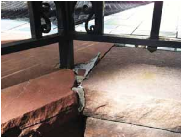
Fig. 2.1.A.52 Cracked paving noted at the guardrail posts along the edge of the patio on the southeast side of the First Floor Palm Room.
