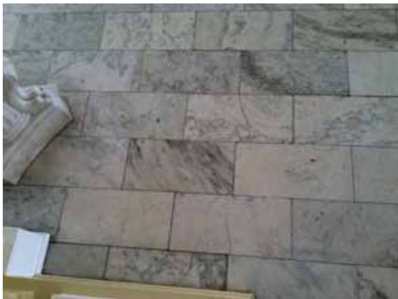
Fig. 3.0.C.22 Areas of cracked, deteriorating, and soiled marble flooring observed in the Palm Room on the south side of the First Floor.
