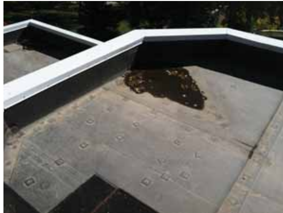
Fig. 2.1.A.42 Areas of standing water observed at the flat roof decks covered with an EPDM membrane.
