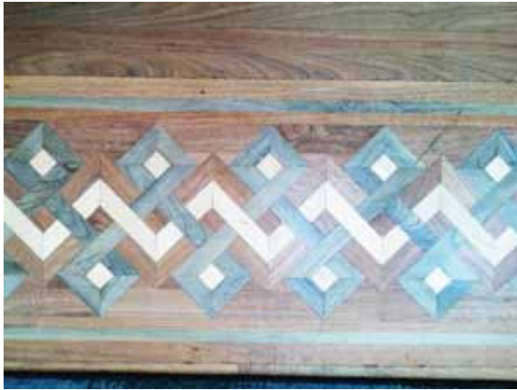
Fig. 3.0.C.20 General wear-and-tear observed at the wood floors in the Governor's Spouse's Home Office on the Second Floor.
