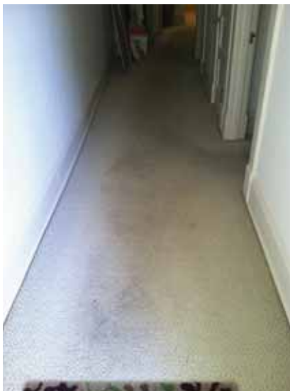
Fig. 3.0.C.28 Typical instance of soiled and worn carpet observed throughout the personnel office spaces on the east side of the building between the First and Second Floors.
