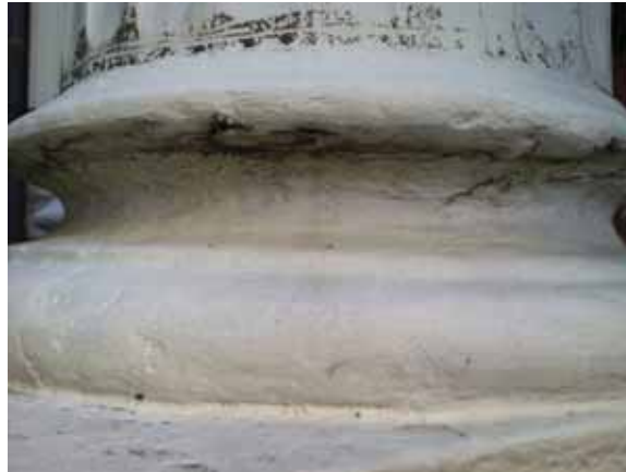
Fig. 2.1.A.22 Cracking and peeling paint exposing the column's substrate material underneath to the elements.
