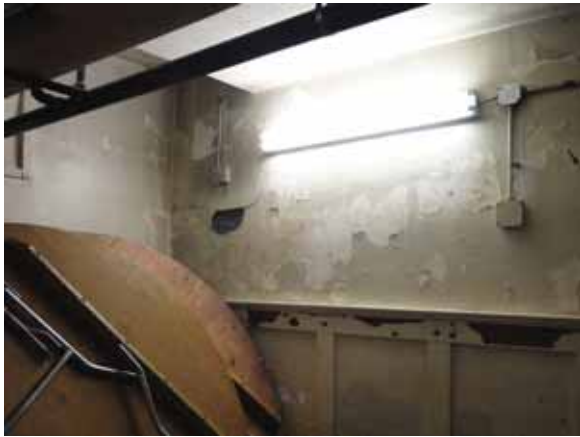
Fig. 3.0.C.7 Peeling paint and cracking noted at a wall of the storage space located on the north side of the Basement Floor.
