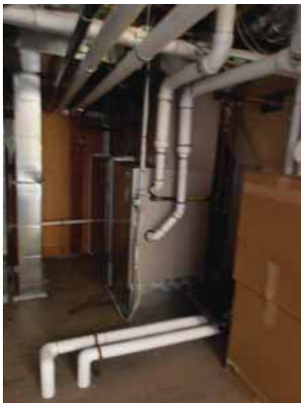
Fig. 2.4.A.19 – Furnace in attic
