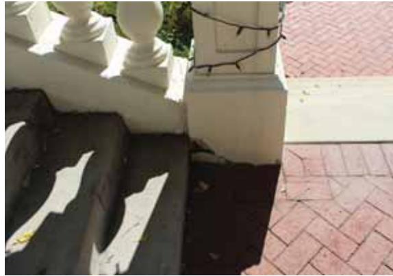
Figure 2.3.B.4 – Broken Pillar Base
