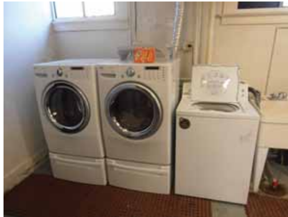
Fig. 2.4.A.27 – Dryer vented to outside
