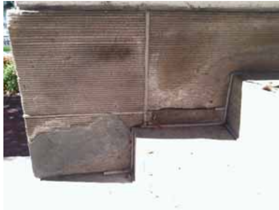
Fig. 2.1.A.10 Areas of poor repairs of the foundation are beginning to deteriorate.
