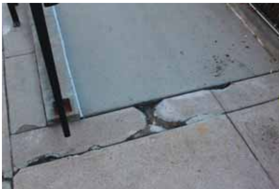
Figure 2.3.A.6 – Broken Site Concrete, Recommended for Replacement
