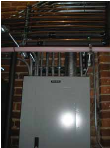
Fig. 2.4.B.3 – Water and coolant lines above panel
