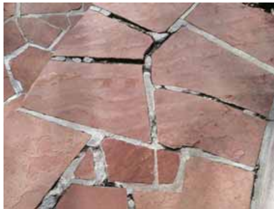
Fig. 2.1.A.49 Deteriorating mortar noted between areas of the stone pavers throughout the site.
