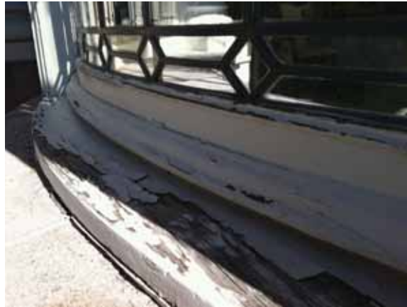
Fig. 2.1.A.16 Widespread peeling and cracking paint noted at the wood trim around the exterior of the building.
