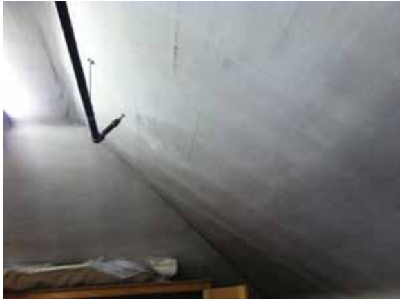
Fig. 3.0.C.2 Water damage and cracking observed at the ceilings throughout the attic storage space on the Third Floor.
