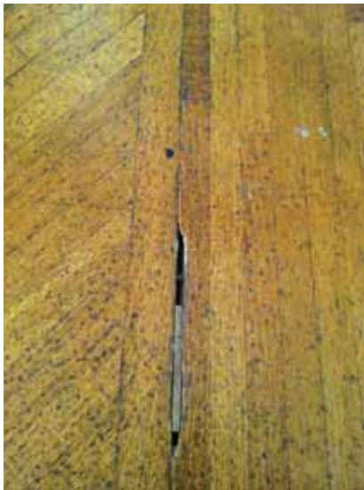
Fig. 3.0.C.16 Damaged sections of the wood floors observed throughout the First Floor.
