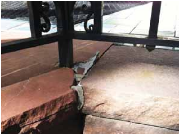
Fig. 2.1.B.3 Spalling and cracking paving at the patio on the southeast side of the First Floor Palm Room.
