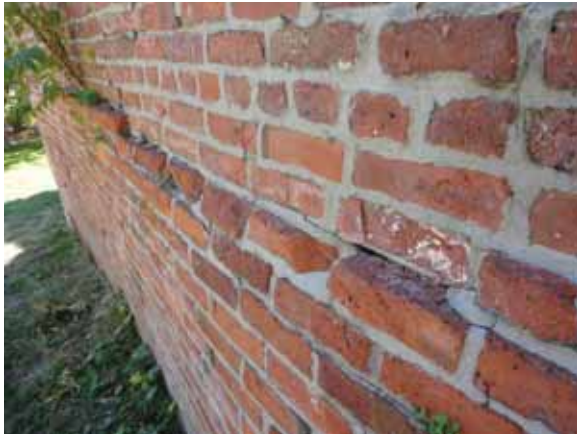
Fig. 2.1.A.63 Portion of the brick perimeter wall noted to be failing structurally along the eastern and southern portions of the terraced grounds, near the Tebo Visitor's Center.
