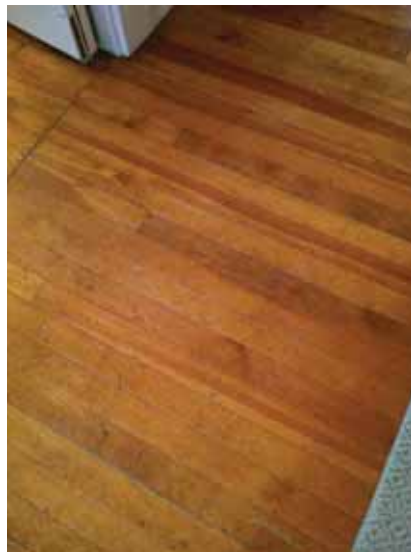
Fig. 3.0.C.18 General wear-and-tear noted at the wood floors in the Living Room on the Second Floor.
