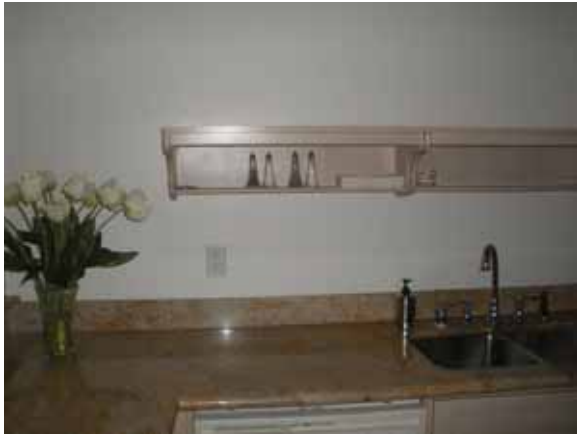
Fig. 2.4.B.2 – Receptacle without GFI protection
