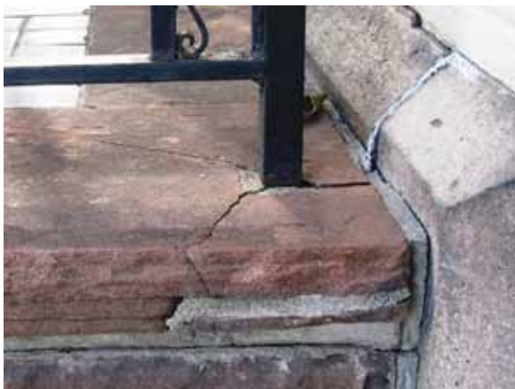
Fig. 2.1.B.4 Spalling and cracking paving at the patio on the southeast side of the First Floor Palm Room.
