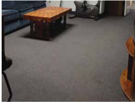
Fig. 3.0.C.29 Soiled and worn carpet observed in the Trooper Down Room on the Basement Floor.
