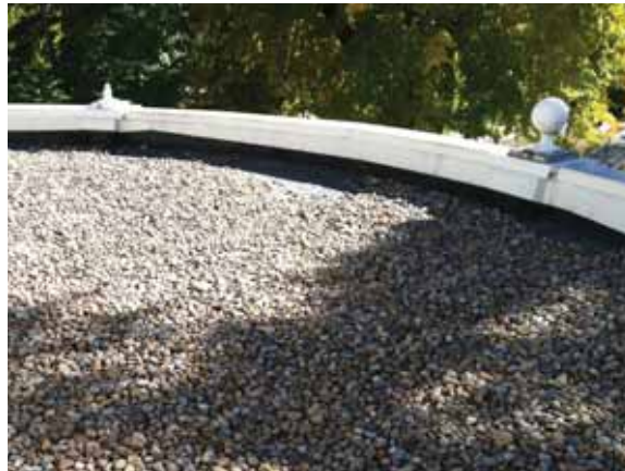
Fig. 2.1.A.43 Areas with thin or no ballast along the perimeter edges of the flat roof decks.
