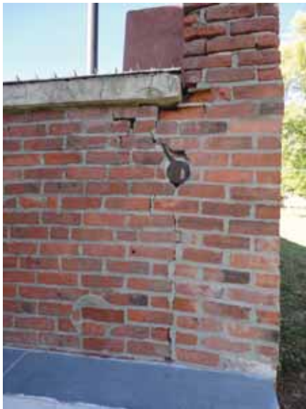
Fig. 2.1.A.64 Portion of the brick perimeter wall noted to be failing structurally along the eastern and southern portions of the terraced grounds, near the Tebo Visitor's Center.
