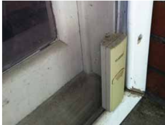
Fig. 2.1.B.11 A security device observed on the exterior side of a window.
