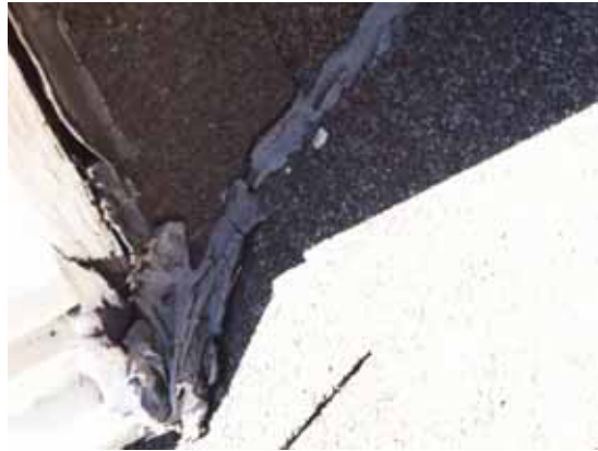
Fig. 2.1.A.36 Areas of deteriorating flashing and sealant observed on the roof.
