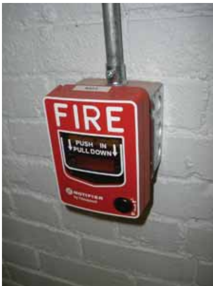
Fig. 2.4.A.11 – Fire alarm pull station
