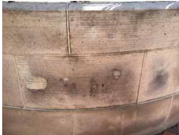
Fig. 2.1.A.11 Areas of poor repairs of the foundation are beginning to deteriorate.
