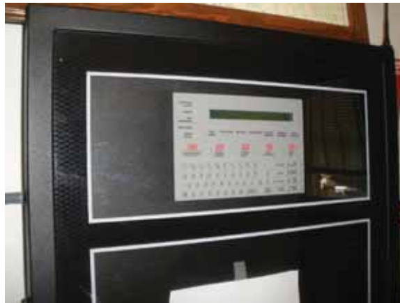
Fig. 2.4.A.12 – Fire alarm control panel
