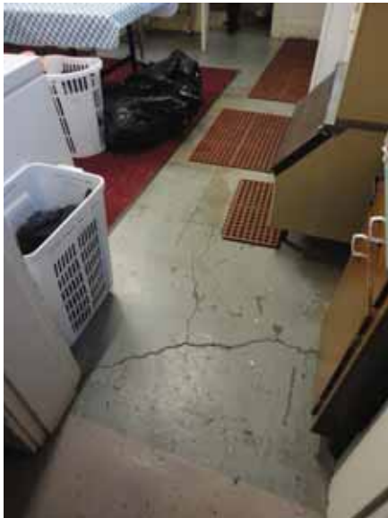
Fig. 3.0.C.33 Cracked concrete flooring observed in areas throughout the Basement Floor.
