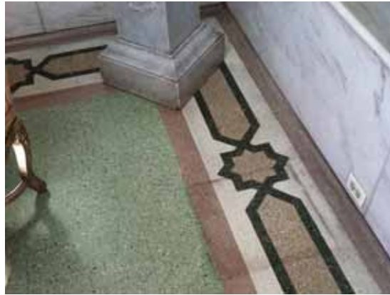
Fig. 3.0.C.23 Area of soiled terrazzo flooring observed in the Well Room at the southwest corner of the First Floor.
