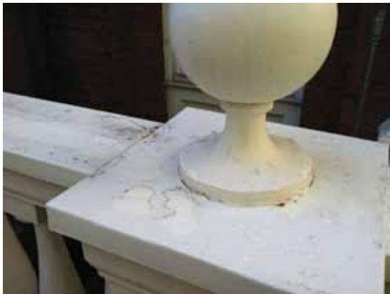
Fig. 2.1.A.20 The top surface of the roof deck railings appears to be generally flat, allowing water to stand and cause damage.
