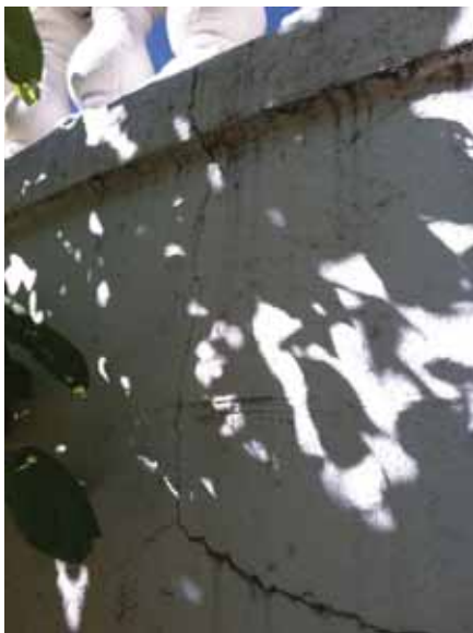
Fig. 2.1.A.59 Widespread cracking observed at the curved white retaining wall with soiling noted along the landscaped areas.
