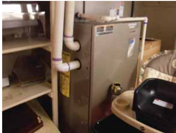
Fig. 2.4.A.15 – Furnace in basement
