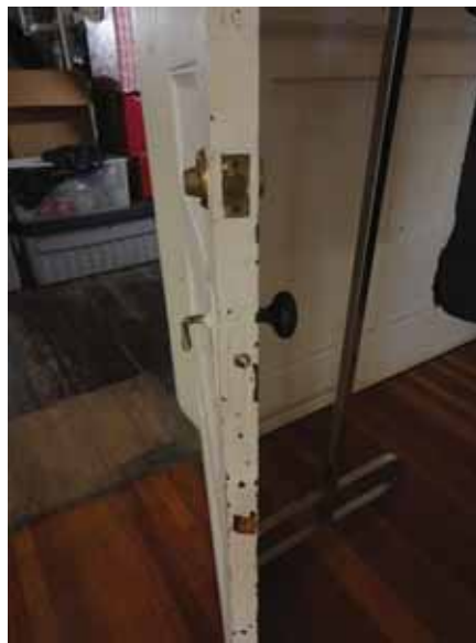
Fig. 3.0.C.35 Wear-and-tear observed at the doors throughout the Basement Floor.
