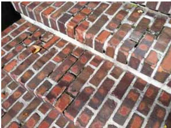
Fig. 2.1.A.47 Deteriorating mortar noted at areas of the brick pavers and stairways throughout the site.
