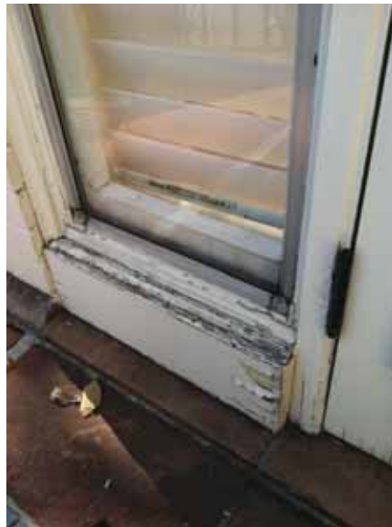
Fig. 2.1.A.30 Cracking and peeling paint noted at the side-lites on either side of the patio doors on the east end of the south side of the First Floor Palm Room.
