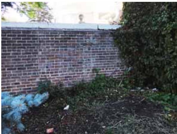
Fig. 2.1.A.65 General deterioration of the brick perimeter walls noted during the site survey visit.
