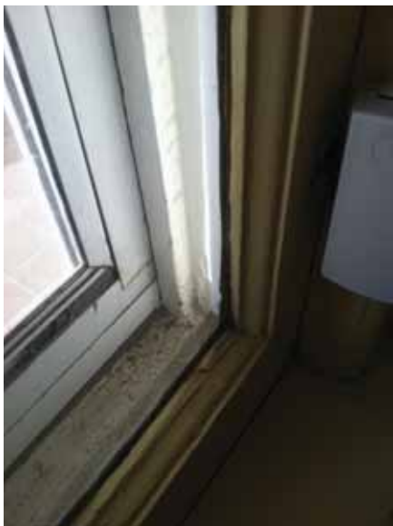
Fig. 2.1.A.23 Damage noted on the interior side of a few of the First through Third Floor windows.
