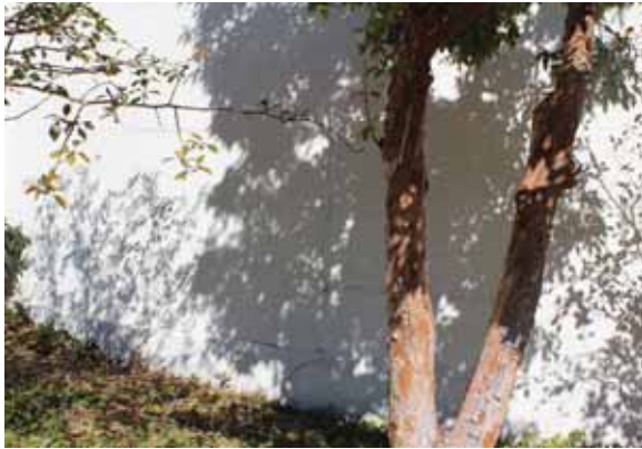
Figure 2.3.B.1 – Retaining Wall Cracking
