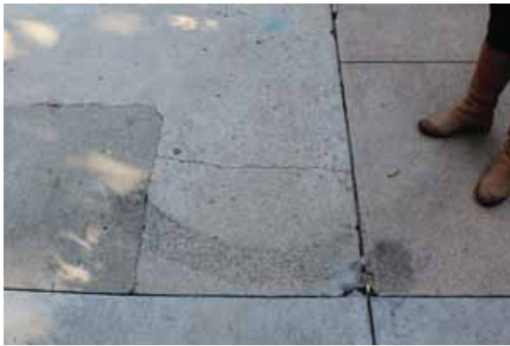
Figure 2.3.A.4 – Site Concrete Crack
