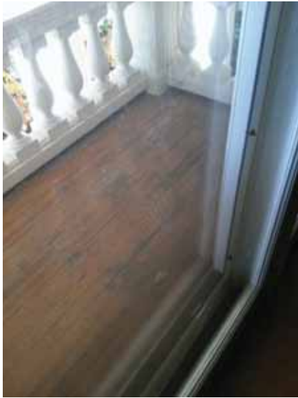
Fig. 2.1.A.45 Deterioration of the wood decking noted at the porch outside of the Second Floor office on the west side of the building.
