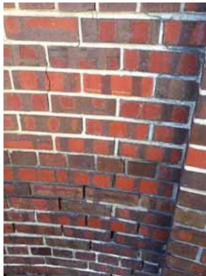
Fig. 2.1.A.67 Cracking of the brick perimeter walls with deteriorating and missing mortar noted during the site survey visit.
