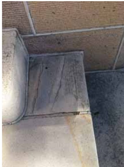
Fig. 2.1.A.55 Areas of spalling and soiling observed at the exterior stairways around the building.
