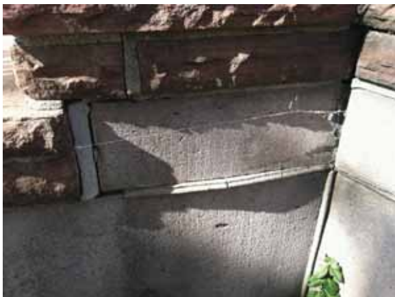
Fig. 2.1.A.9 Deterioration of the mortar noted at the brick and at the foundation.
