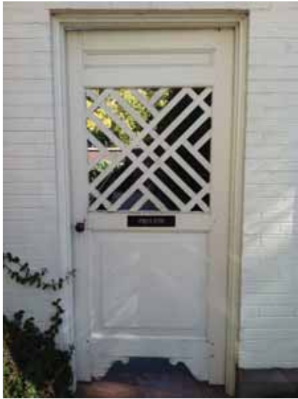
Fig. 2.1.A.32 Wood door in the east brick perimeter wall observed to have cracking wood and peeling paint.
