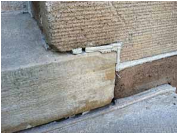
Fig. 2.1.A.8 Deterioration of the mortar noted at the foundation.
