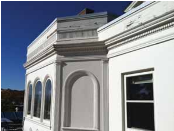
Fig. 2.1.A.14 Widespread peeling and cracking paint noted at the wood trim around the exterior of the building.
