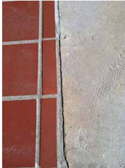
Fig. 2.1.A.48 Deteriorating mortar noted between the stone stairway and tile paving at the porch on the west side of the building.
