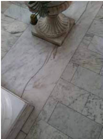
Fig. 3.0.C.21 Areas of cracked and deteriorating marble flooring observed in the Palm Room on the south side of the First Floor.
