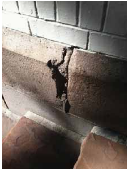
Fig. 2.1.A.5 Cracking and spalling noted at the foundation.
