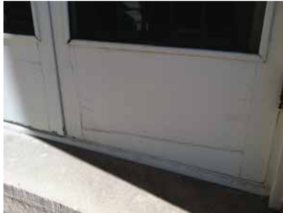
Fig. 2.1.A.29 Doors with peeling and cracking paint and general deterioration at the covered porch on the west side of the building.
