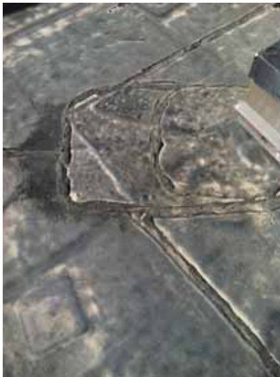
Fig. 2.1.A.41 General deterioration of the EPDM membrane, former patchwork, and sealant noted at the flat roof deck areas.
