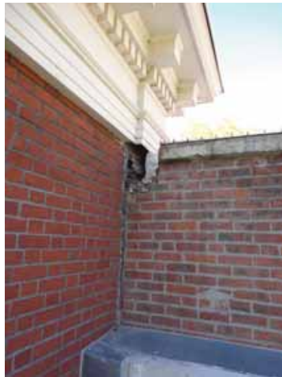
Fig. 2.1.A.66 General deterioration and damage noted at the brick perimeter walls during the site survey visit.
