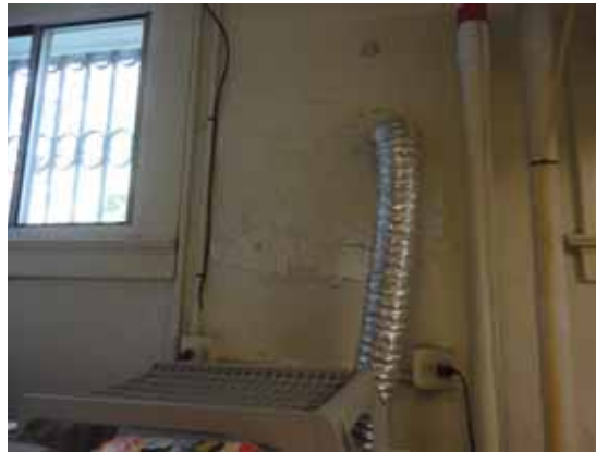
Fig. 3.0.C.10 Damage observed at the east wall and south of the window in the Basement Floor Laundry Room.
