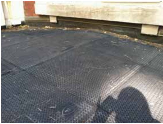
Fig. 2.1.A.40 Leaves and standing water observed along the front edge of the roof over the front porch on the north side of the building.
