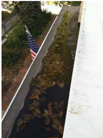
Fig. 2.1.A.37 Corrosion and deteriorating sealant noted at the readily observable roof vents.
