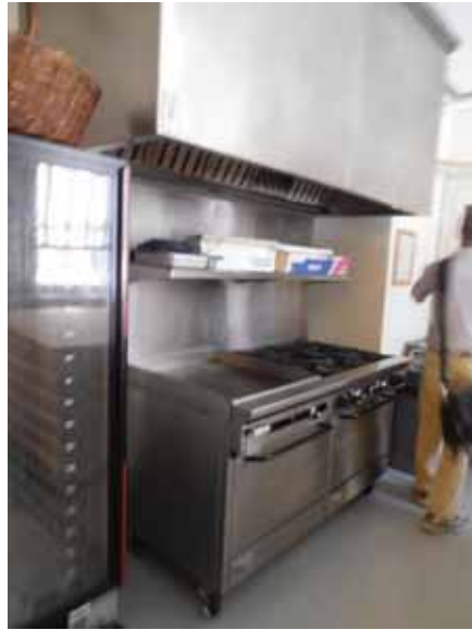
Fig. 2.4.A.20 – Kitchen exhaust hood
