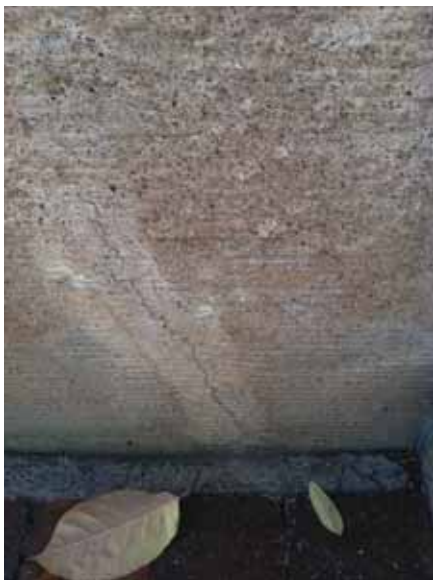
Fig. 2.1.A.3 Cracking of the foundation.
