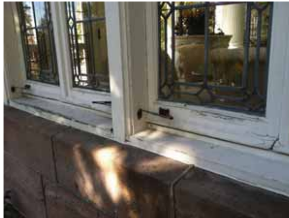
Fig. 2.1.A.25 First Floor windows noted to have peeling and cracking paint at the wood frames.
