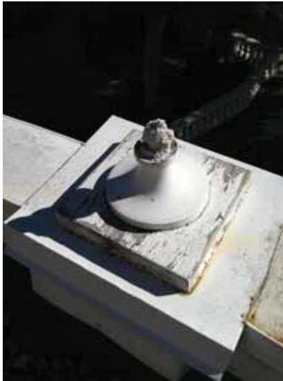
Fig. 2.1.A.19 Extensive deterioration noted at the decorative elements along the roof deck railings.
