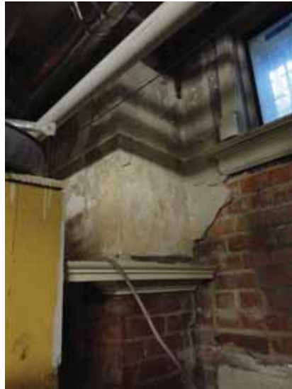
Fig. 3.0.C.9 Wall coating observed to be cracking off of the east wall under a window in the Furnace Room at the northeast corner of the Basement Floor.
