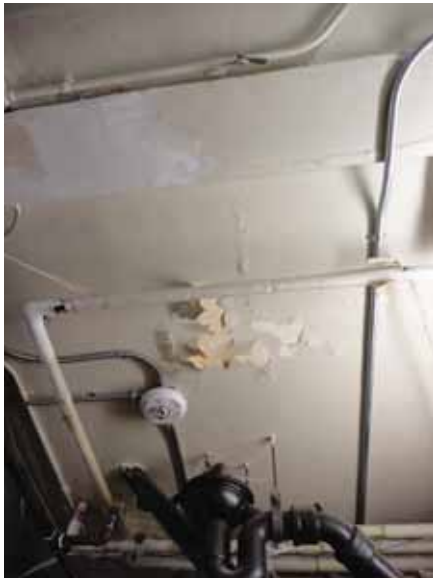
Fig. 3.0.C.3 Peeling paint observed at the ceiling on the Basement Floor.
