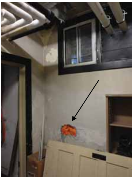
Fig. 3.0.C.8 Damage noted along the south wall of the building in the Mechanical Room on the east end of the south side of the Basement Floor.
