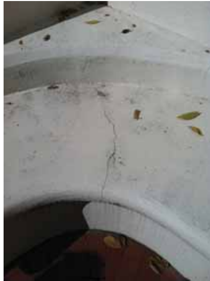
Fig. 2.1.A.60 Cracking observed at the seating and flat surfaces at the curved white retaining wall.
