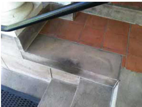
Fig. 2.1.A.53 Soiling noted to the paving at the covered porch on the west side of the building.
