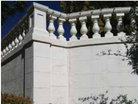
Fig. 2.1.A.58 Widespread cracking observed at the curved white retaining wall.
