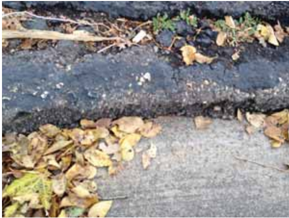
Figure 2.1.A.25 – Asphalt Thickness above Gutter
