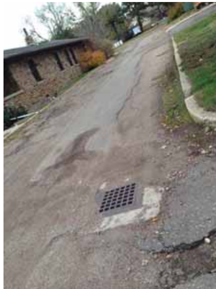
Figure 2.1.A.14 – Area Drain near Building #67
