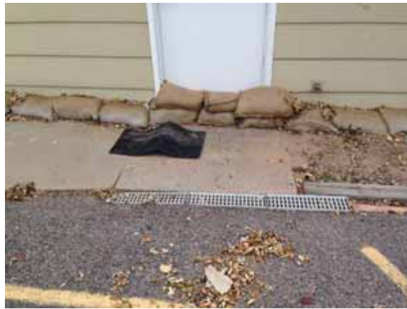
Figure 2.1.A.13 – Trench Drain and Sandbags at Building #97
