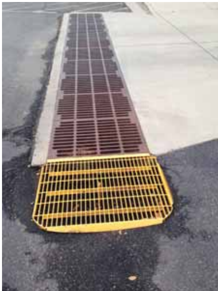
Figure 2.1.A.11 – Trench Drain near Building #47
