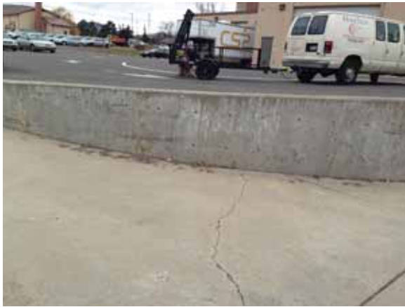
Figure 2.1.A.21 – Site Concrete Crack
