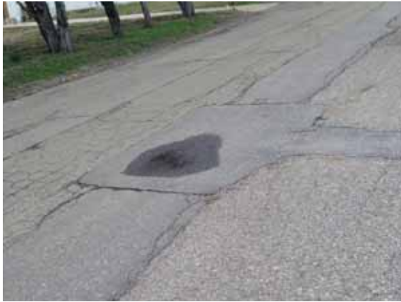
Figure 2.1.A.31 – Uneven, Patched Asphalt
