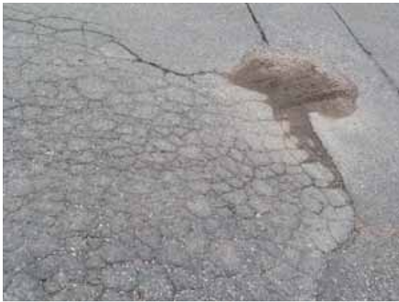
Figure 2.1.A.32 – Poor Asphalt Condition in Parking Area
