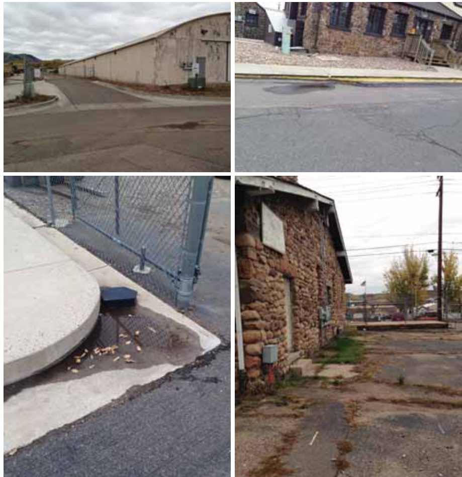
Figure 2.1.A.7 – Evidence of Local Ponding
