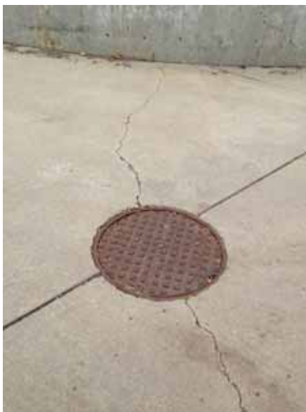
Figure 2.1.A.22 – Site Concrete Crack
