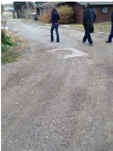
Figure 2.1.A.33 – Poor Asphalt Condition in Drive Aisle
