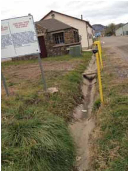
Figure 2.1.A.17 – Drainage Channel/ Culvert System
