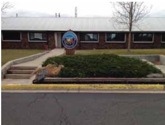
Figure 2.1.A.27 – Asphalt Cracking near Building #120
