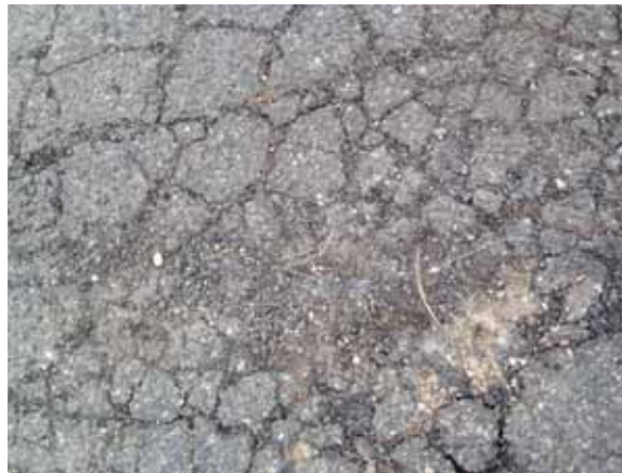
Figure 2.1.A.29 – Broken Asphalt in Poor Condition
