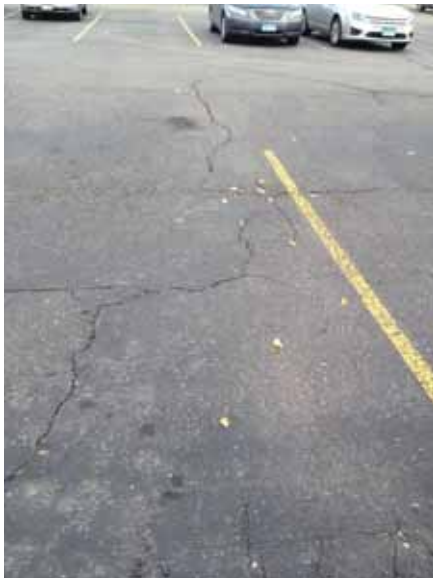
Figure 2.1.A.26 – Asphalt Cracking near Building #120
