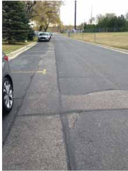
Figure 2.1.A.28 – Uneven Asphalt and Sealed Cracks
